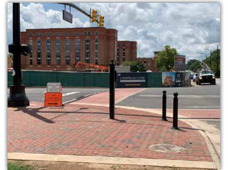
Installation of new curbing, brick pavers and crosswalks is complete on East Thach Avenue in front of the Chapel.
