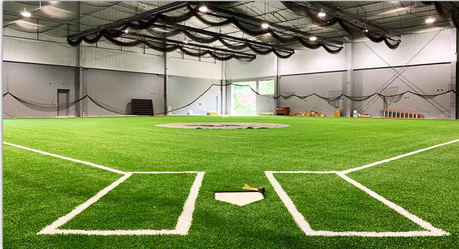
Artificial turf and field plates have been installed, while finishing work takes place on the pitcher's mound.
