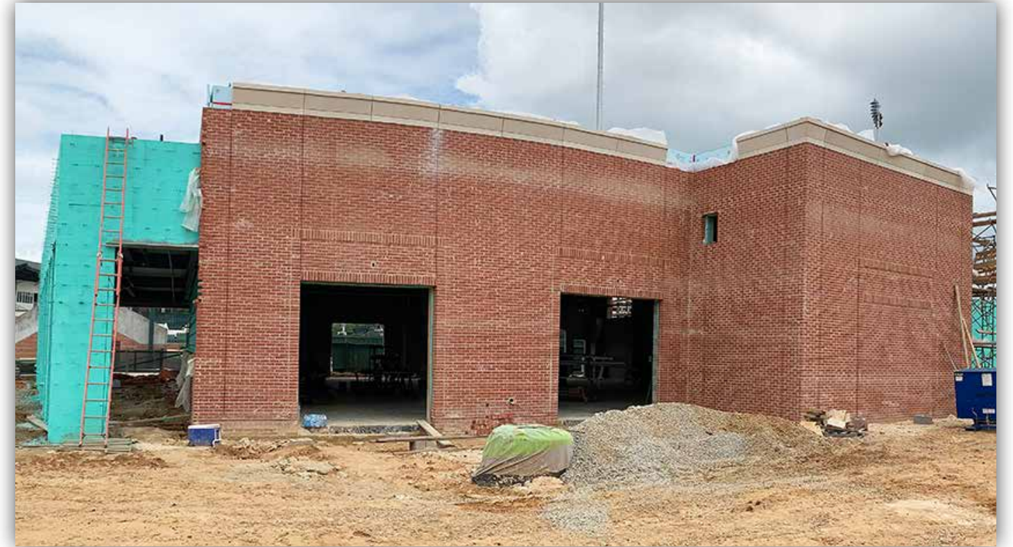
Brick installation is nearly complete on the south side, and precast concrete caps have been placed on top of the brick.
