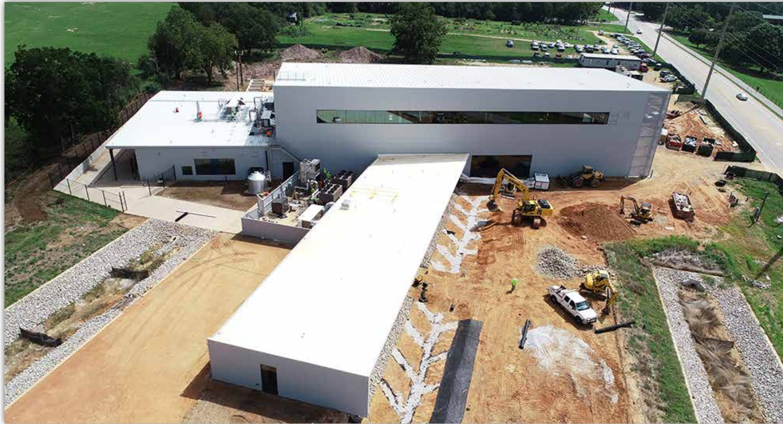
An aerial view of the Advanced Structural Engineering Laboratory site at the corner of West Samford Avenue and Shug Jordan Parkway.
