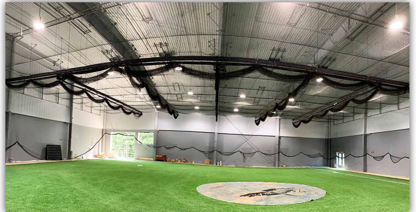
The netting shown at the top of this photo can be lowered to create batting lanes. Installation of this netting is complete.
