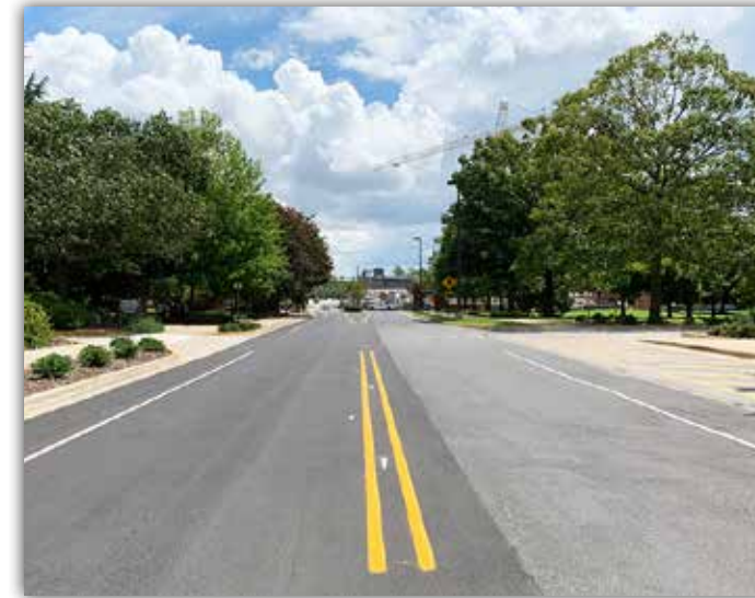
West Thach Avenue, beside the RBD Library, has been repaved following installation of underground power and water piping.
