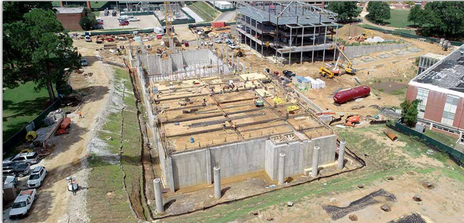
The ACLC's storm shelter walls are complete, and the first floor support structure is being installed.
