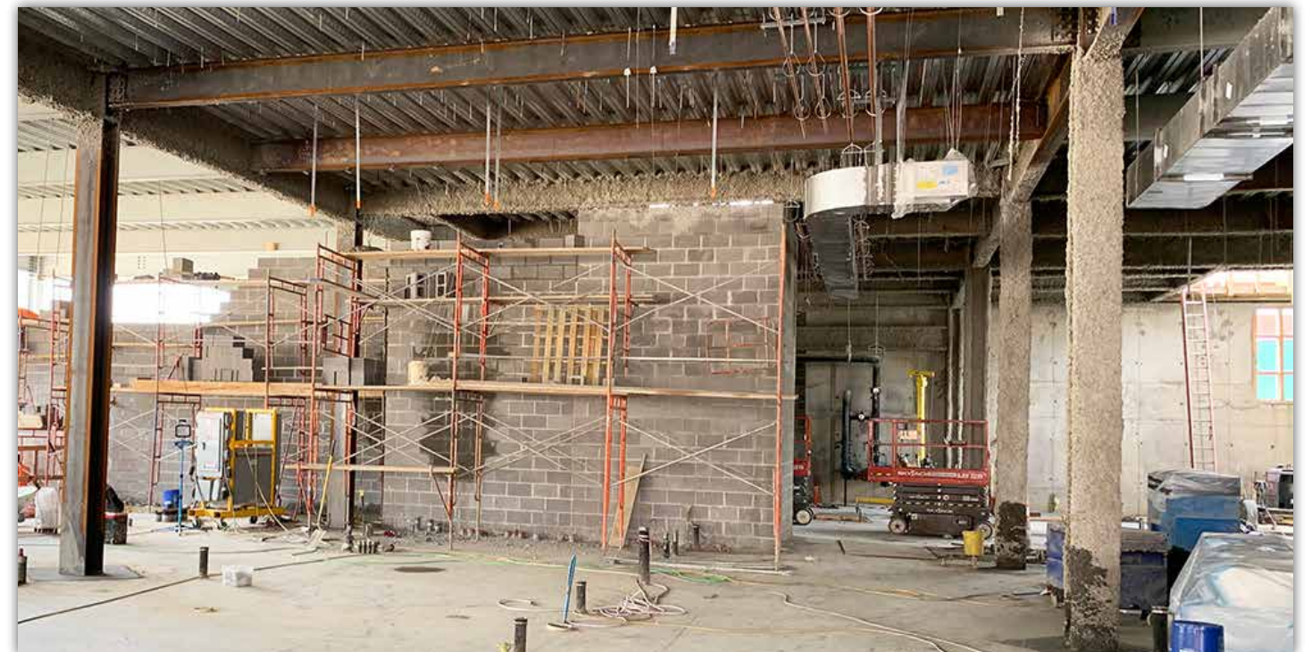
Installation of interior walls, and mechanical, electrical and plumbing systems is underway on the ground floor. The main kitchen and Tiger Dining offices will be located in this area.
