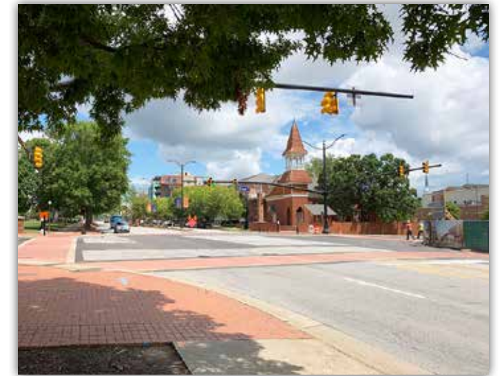
All lanes within the intersection of Thach Avenue and South College Street are now open.
