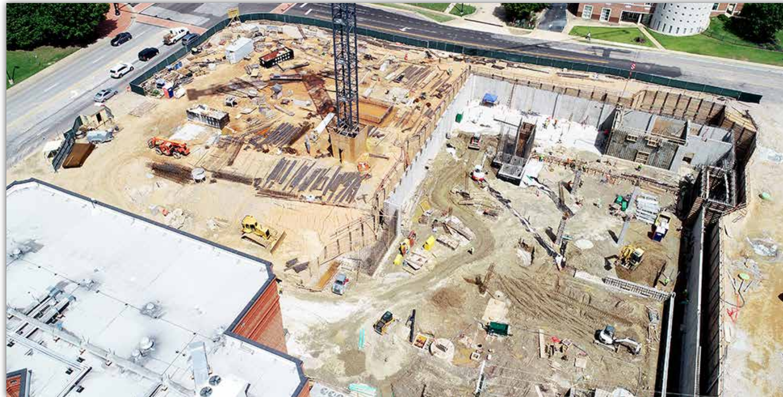
The basement level of the Tony and Libba Rane Culinary Science Center is quickly taking shape as foundation walls, elevator shafts and concrete columns are being installed.
