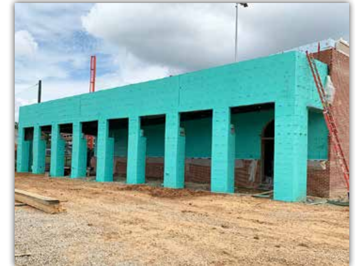
Application of the waterproofing layer is now complete and ready for brick.
