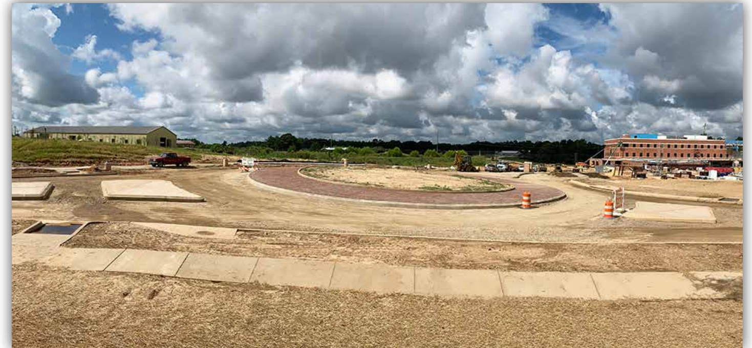
Curbing and concrete islands, which frame the traffic circle, are complete and ready for paving to begin.
