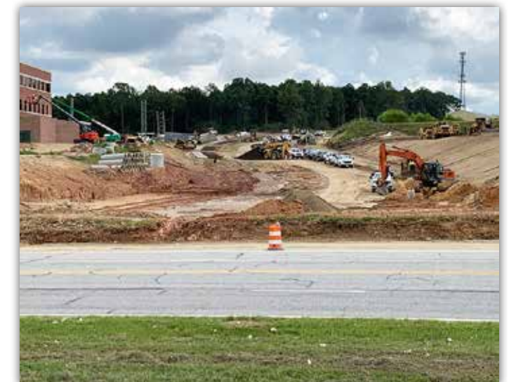
Grading is taking place as the infrastructure work reaches Shug Jordan Parkway.
