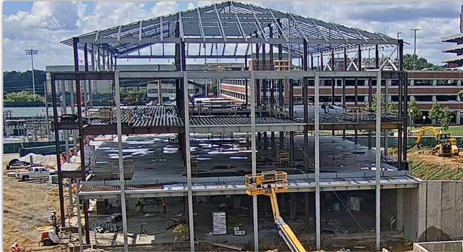
The Central Dining Hall's structural steel framing is in place, and each level is being prepped for concrete floors to be poured.
