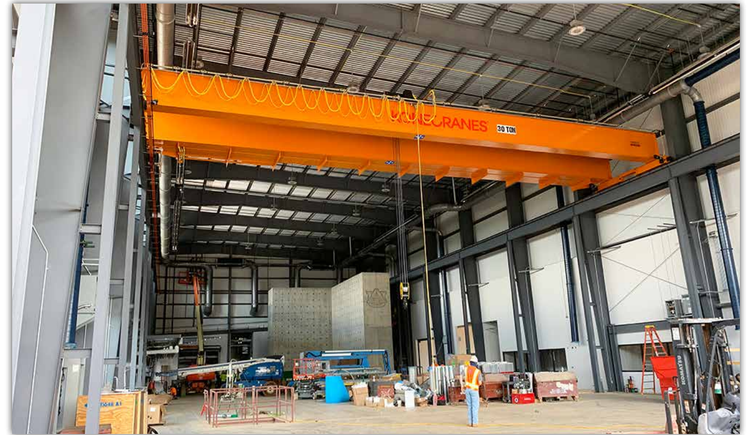
One of the two overhead, heavy lifting cranes was recently installed in the high bay testing laboratory.
