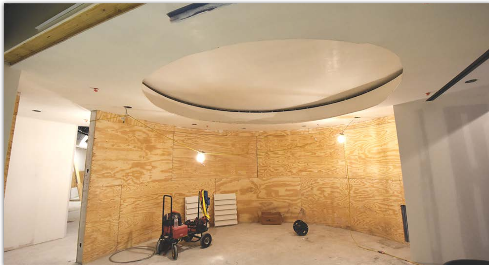
The plywood wall in the men's hype room is ready for accent trim finishes.
