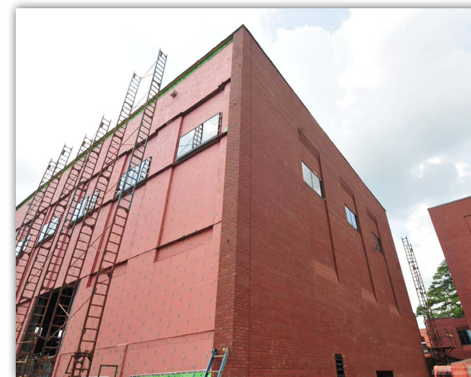
Brick installation on the north side is complete, while installation is ongoing on the east side.
