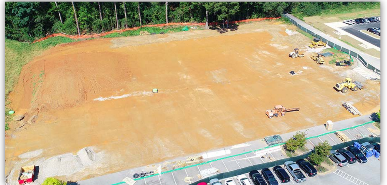
Site work in the southwest area of West Campus parking is ongoing.
