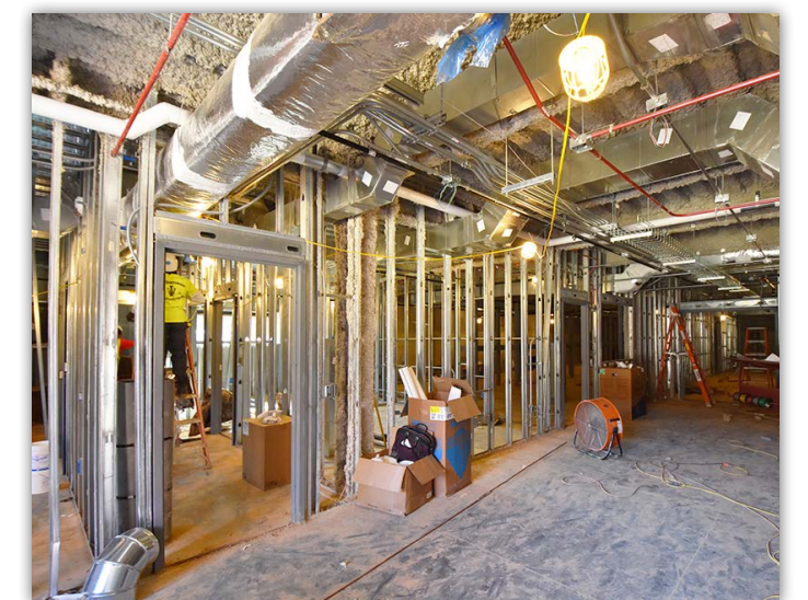
Walls are being framed in the basement area which will include storage space.
