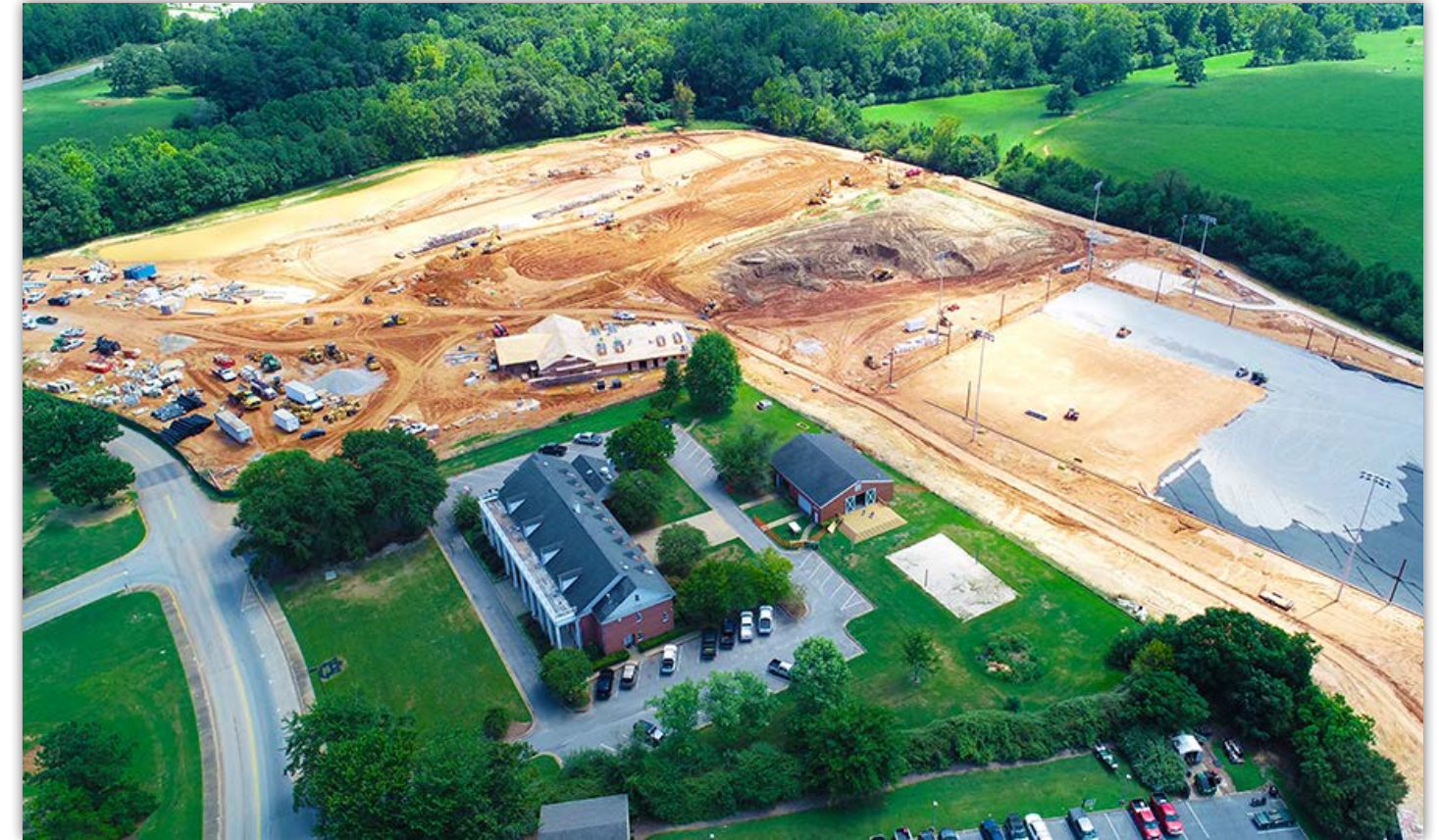
The gravel drainage layer is being applied to the soccer field (right), while site work for two multi-purpose fields and construction of the field house continues.
