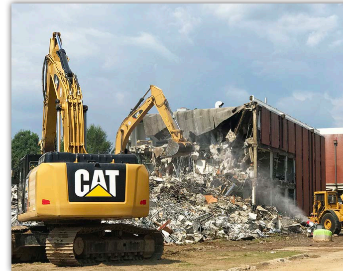
Demolition of Allison Laboratory took place during the summer of 2019. It took just two weeks to demo and remove construction debris from the site.
