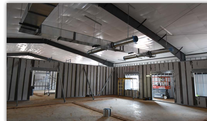
The processing plant panels and roof are complete. Interior wall installation work is in progress.
