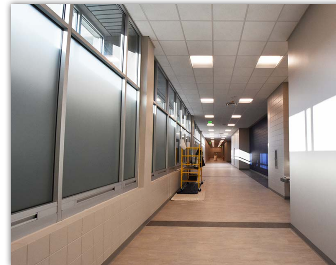
This second floor hallway, which includes recently tinted windows and new luxury vinyl flooring, nears completion.
