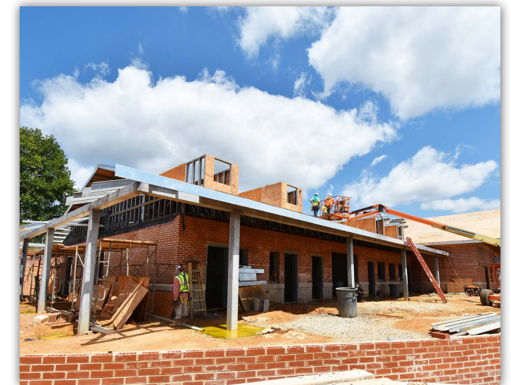
The field house roof decking is installed and is ready for asphalt shingles.
