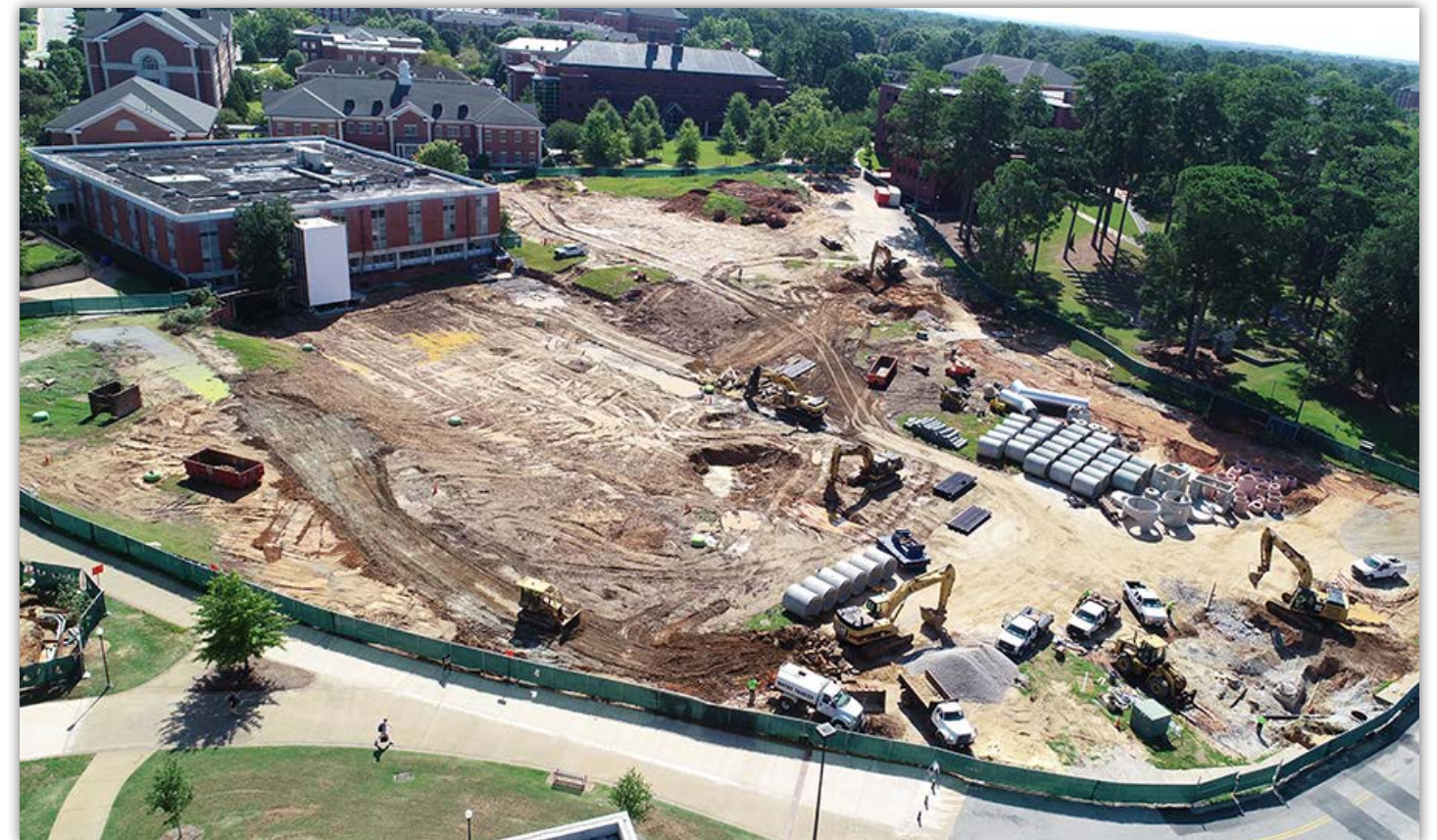
Underground work, such as storm and domestic waterlines and electrical conduits, are currently being installed at the site.
