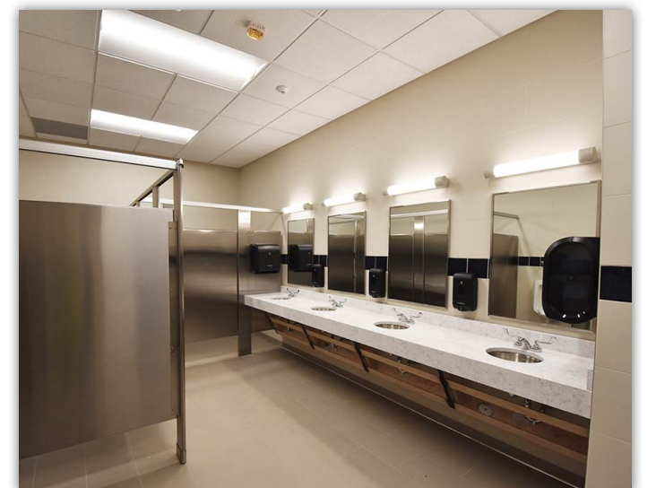
The new men's and women's restrooms are complete. Demolition and new plumbing is in progress on the pre-existing restrooms.
