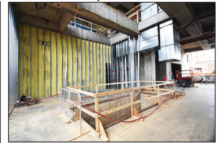
Installation of the interior metal walls, and mechanical, electrical and plumbing systems are ongoing.
