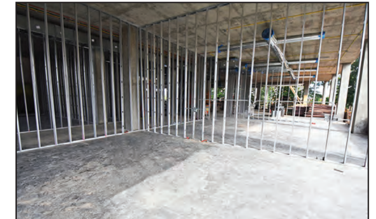
Metal framing of the interior walls is taking place on the first floor.
