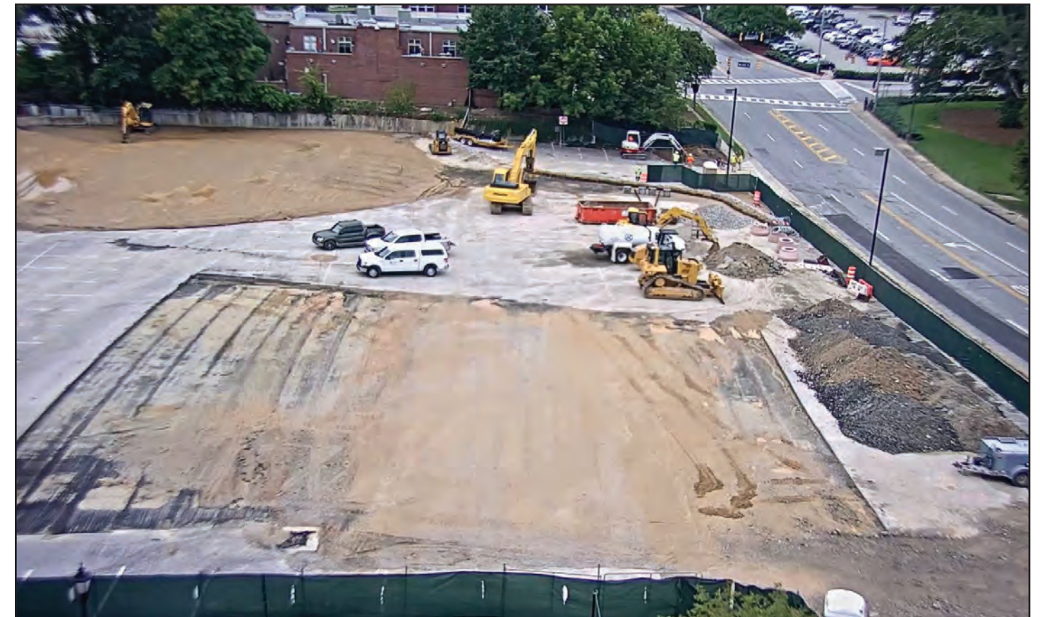
This construction webcam view shows earthwork underway to prepare for drilling of the South College Street Parking Deck's concrete foundation.
