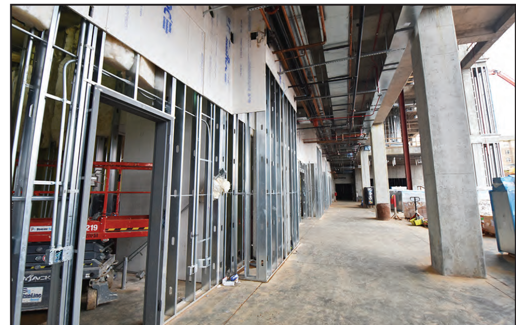
Entrance to the Graduate Business Building from what will be the renovated Lowder Courtyard.
