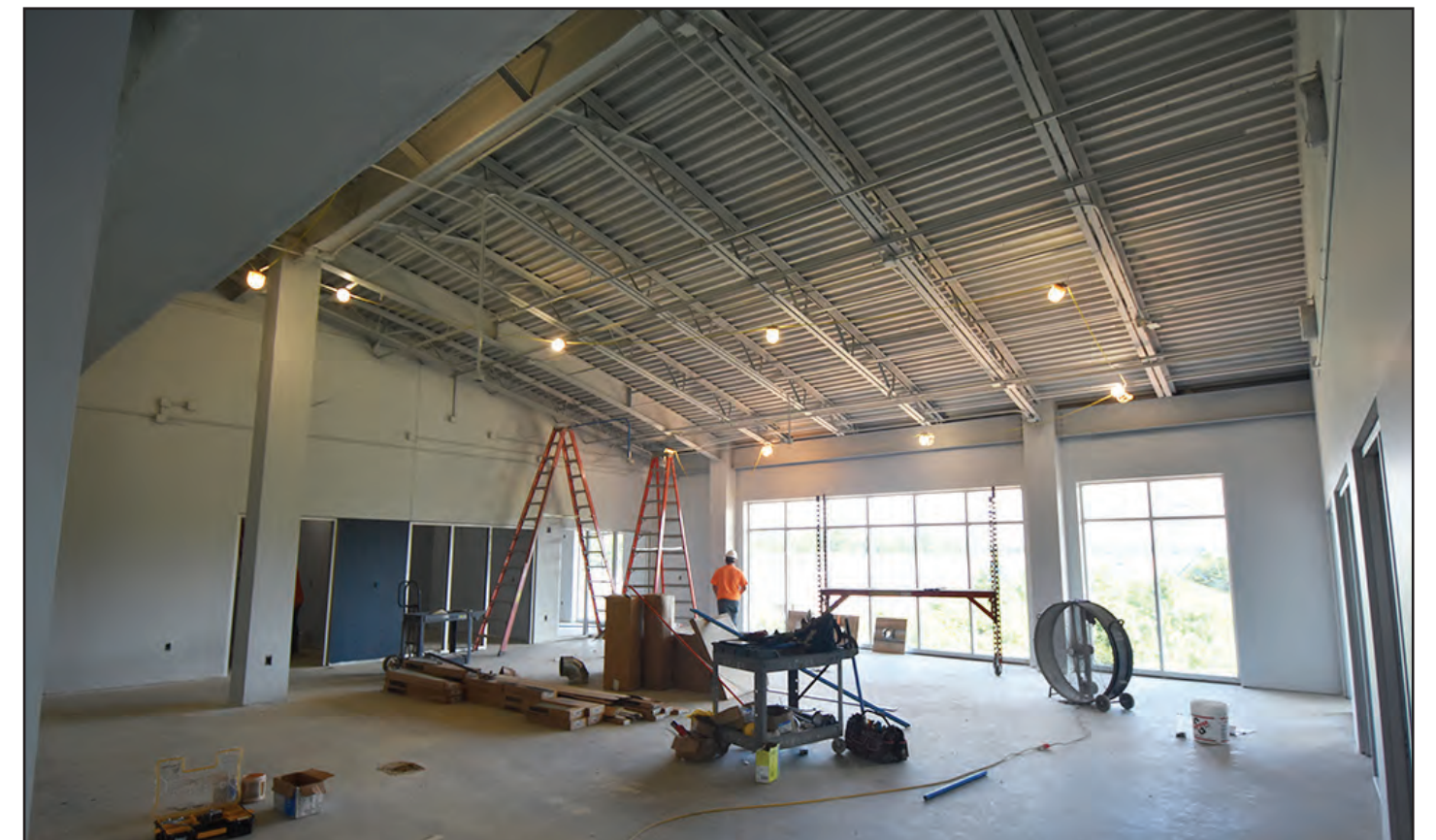
The arched ceiling angles toward large windows overlooking the Auburn Regional Airport.
