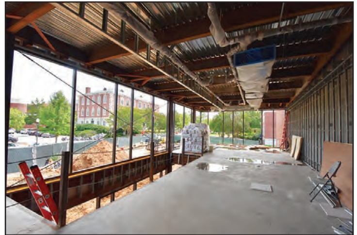
Overhead electrical and mechanical systems going up in the new pavilion area.
