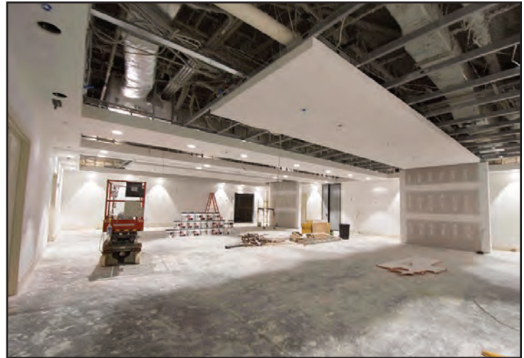
The ceiling is being primed for paint and the walls prepared for wall coverings.
