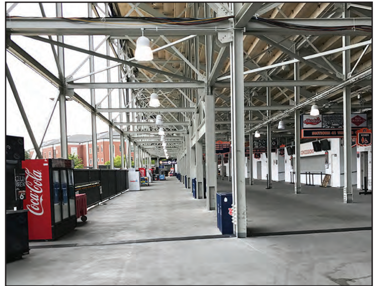
Looking east, the area to the left shows the new north concourse expansion.
