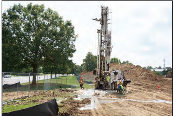
Crew drilling a well to feed the pond that will be located in front of the Center.
