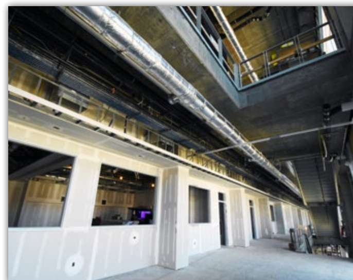
Second floor drywall is taking shape and will soon be ready for paint.
