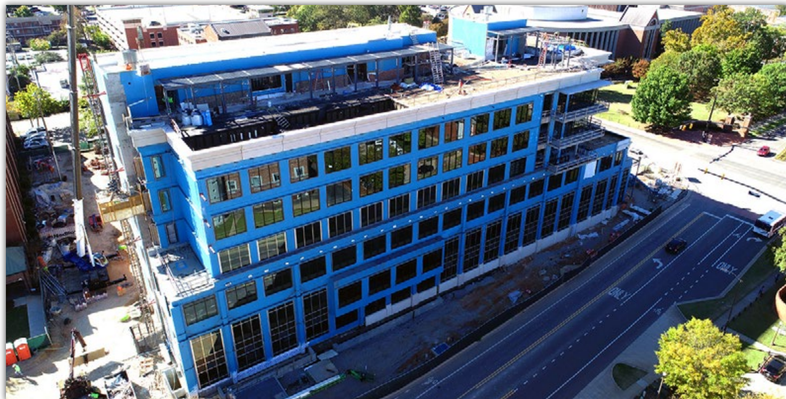
Aerial photo of the Tony and Libba Rane Culinary Science Center taken over East Thach Avenue.
