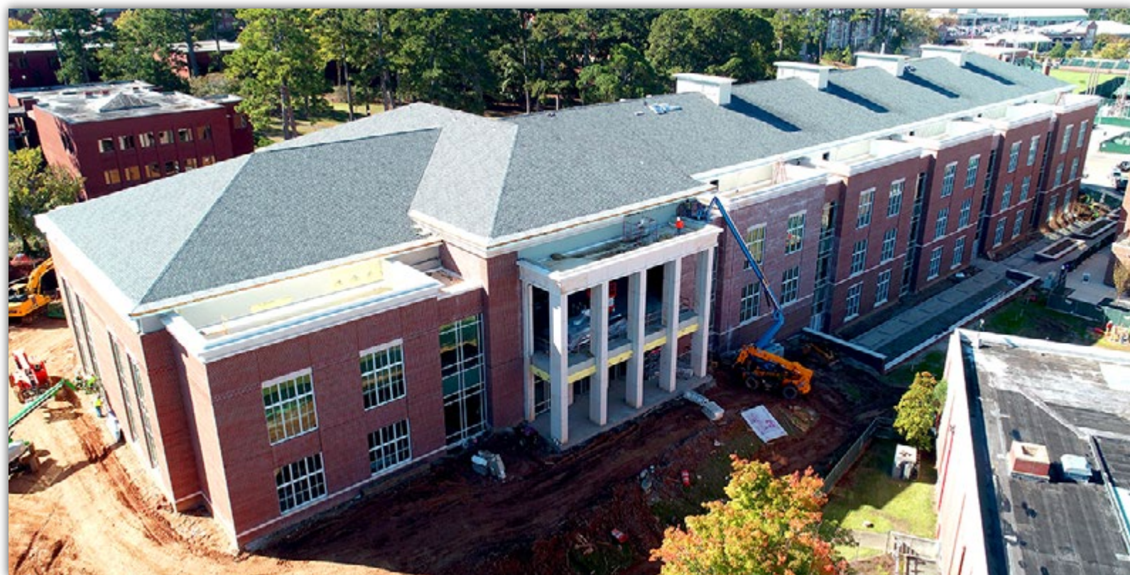
The exterior envelope for the Academic Classroom and Laboratory Complex is nearing completion.
