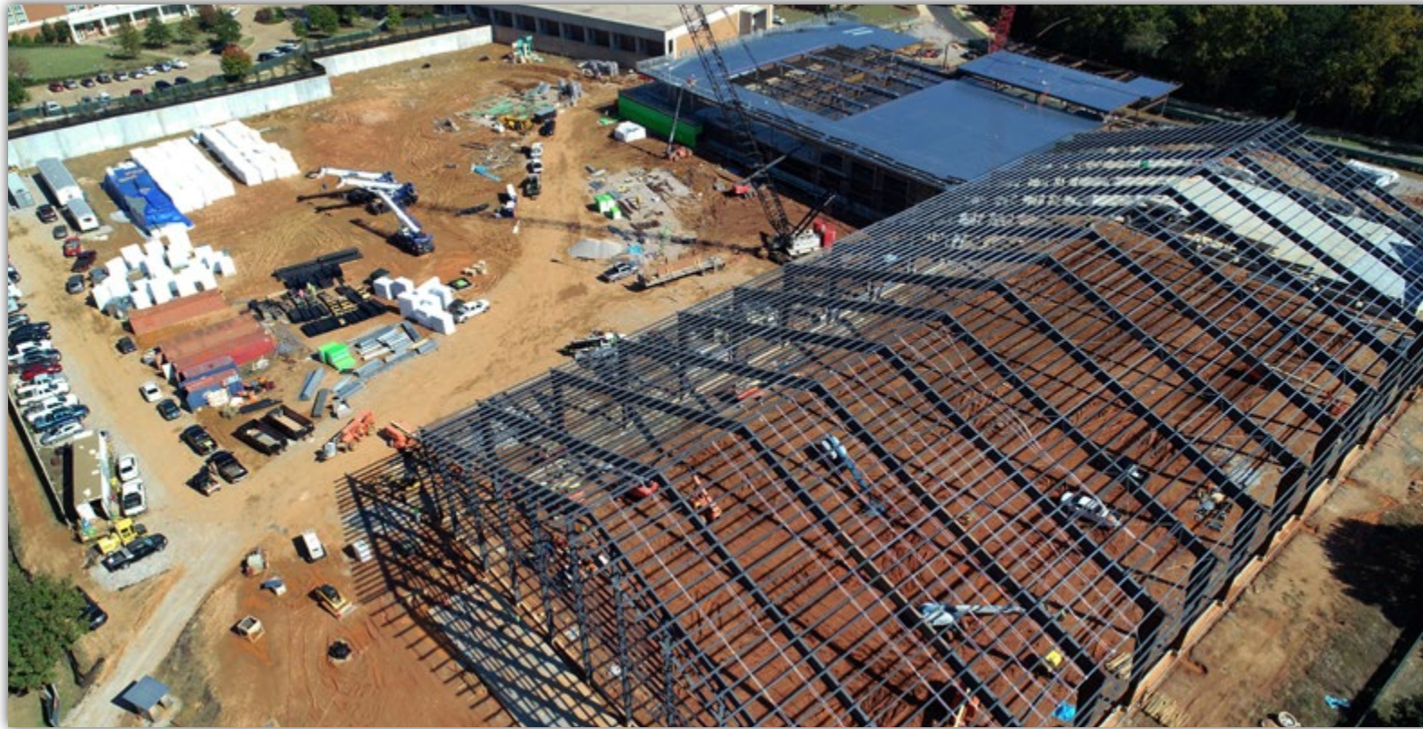
An aerial view of the Football Performance Center site shows the steel going up for the indoor practice field and the operations building.
