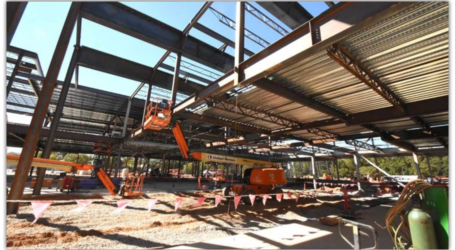
This ground-level view shows ongoing steel work for the locker room, equipment storage and main utility areas.
