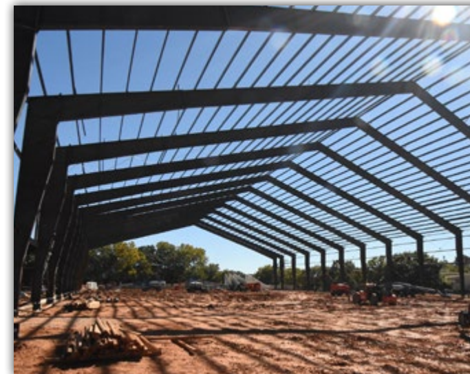
The indoor practice facility's pre-engineered primary and secondary steel frames are nearing completion.
