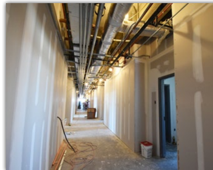
Drywall is going up in The Laurel Hotel & Spa area on the fourth floor of the building.
