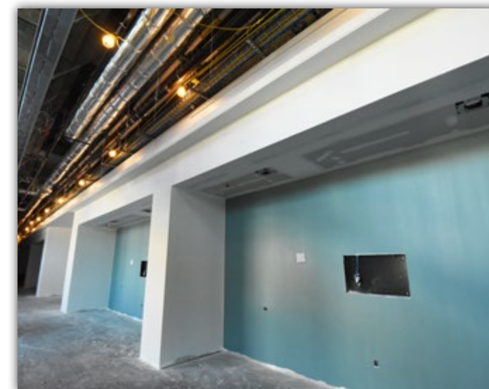
Paint has been applied to the informal learning spaces outside of the first floor classrooms.
