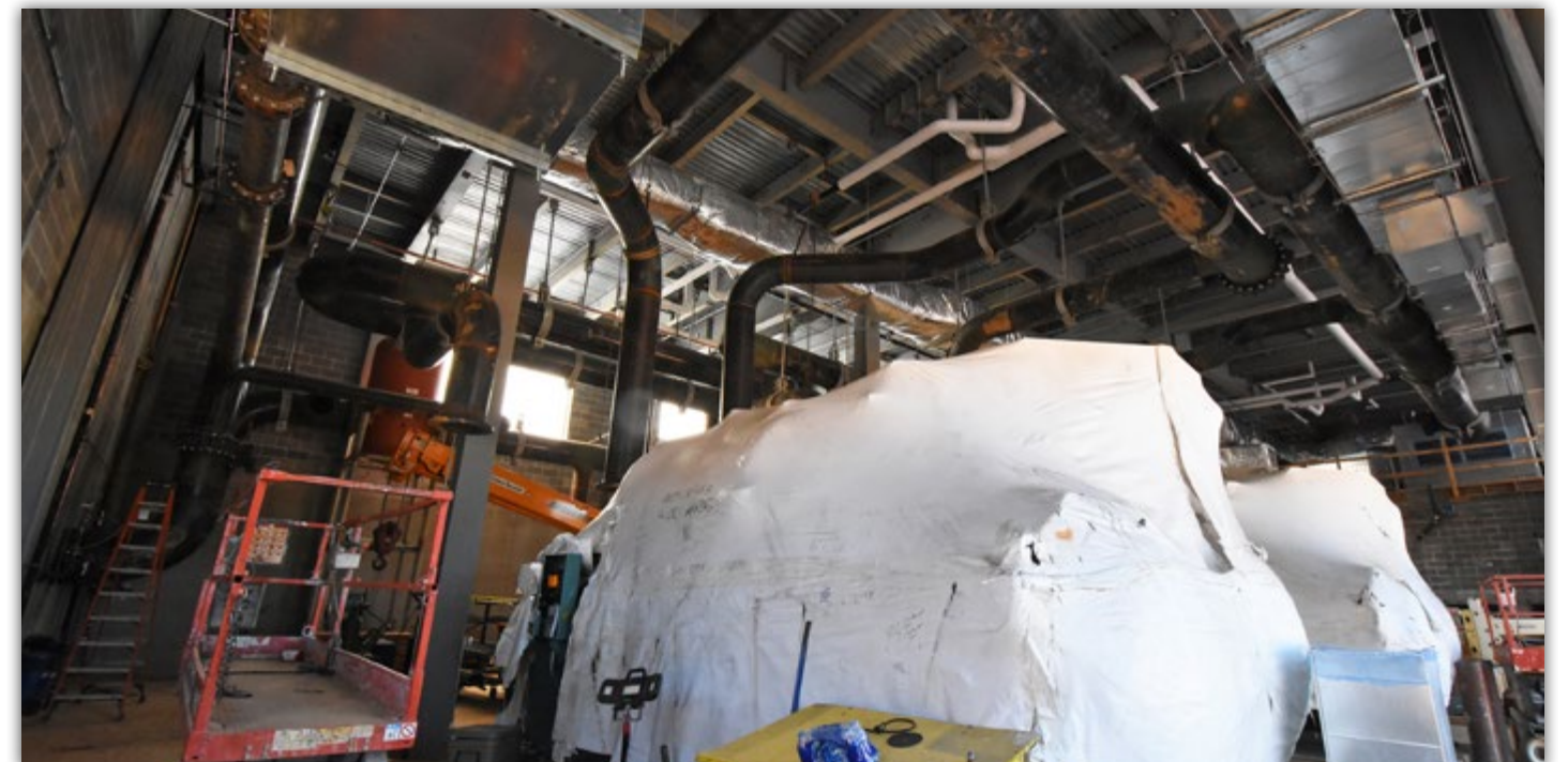
The two 2,500-ton chiller units are ready for final connections. They are currently covered to keep them protected prior to installation.
