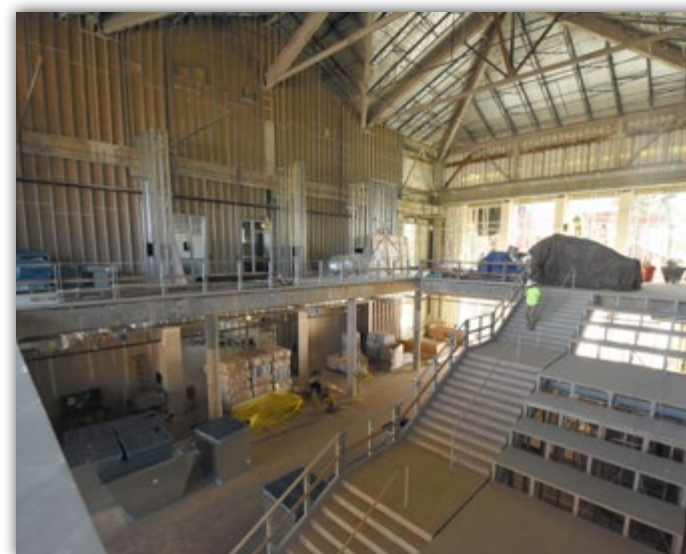
The main entrance monumental staircase has been roughed-in, and the lobby walls are ready for drywall.
