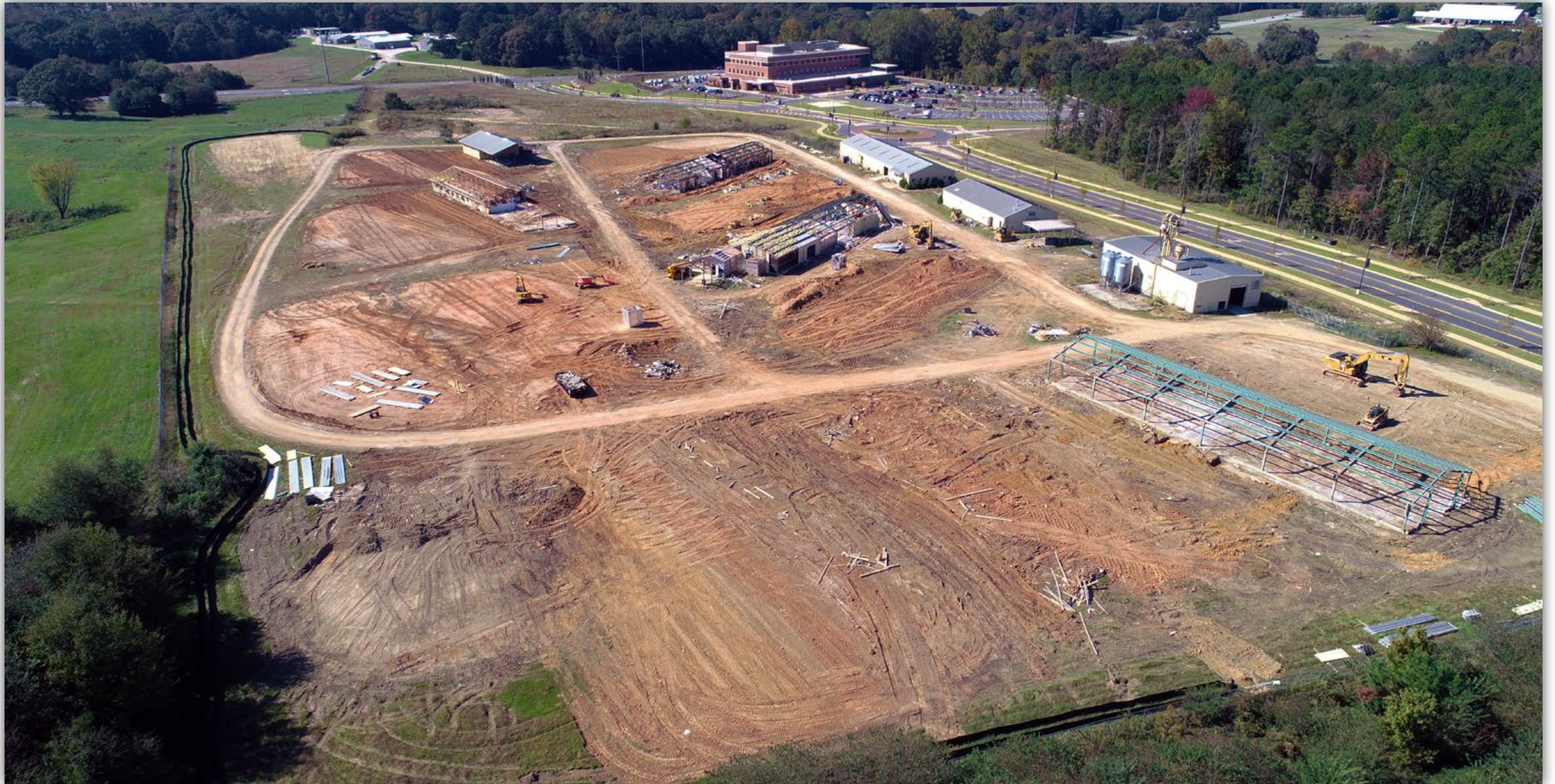
An aerial view of the previous Poultry Research Farm being demolished off Camp Auburn Road where 12 of the farm's 20 buildings have been taken down. The new Charles C. Miller, Jr. Poultry Research and Education Center is located in North Auburn.
