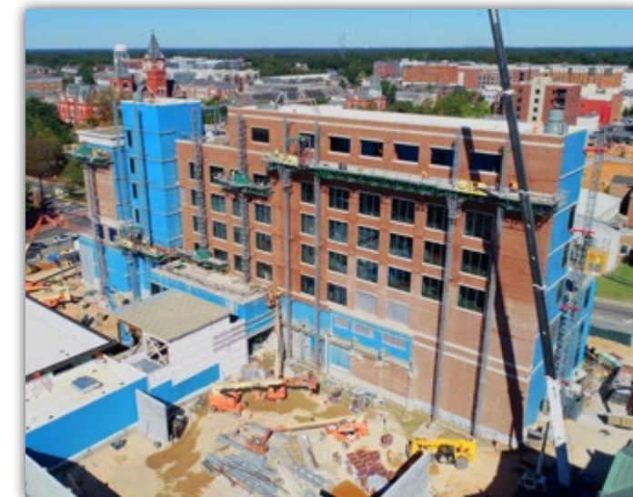
Brick work continues on the south side of the Culinary Science Center.
