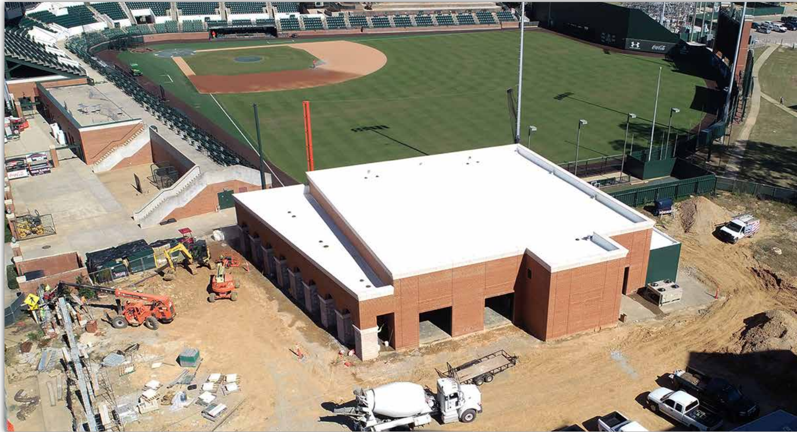
Brick and concrete installation is complete on the exterior of the Plainsman Park Player Development facility.
