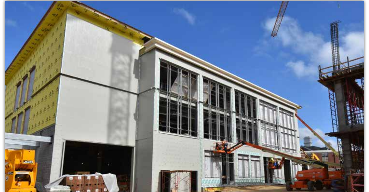
Both the north and south side of the facility will include large windows, which will let in a lot of natural light. This photo is of the building's south side.
