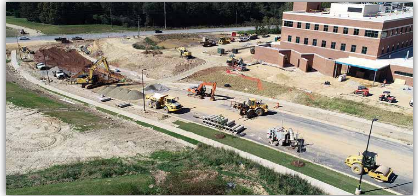
Curbing, paving and landscaping continue to make progress toward Shug Jordan Parkway.
