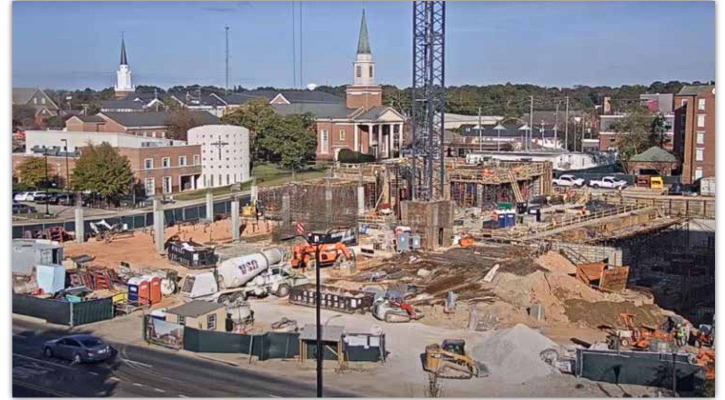
This photo was taken from a camera looking toward the site from the RBD Library. Watch construction live by visiting the Facilities Management webcam page: https://aub.ie/facilitieswebcams .
