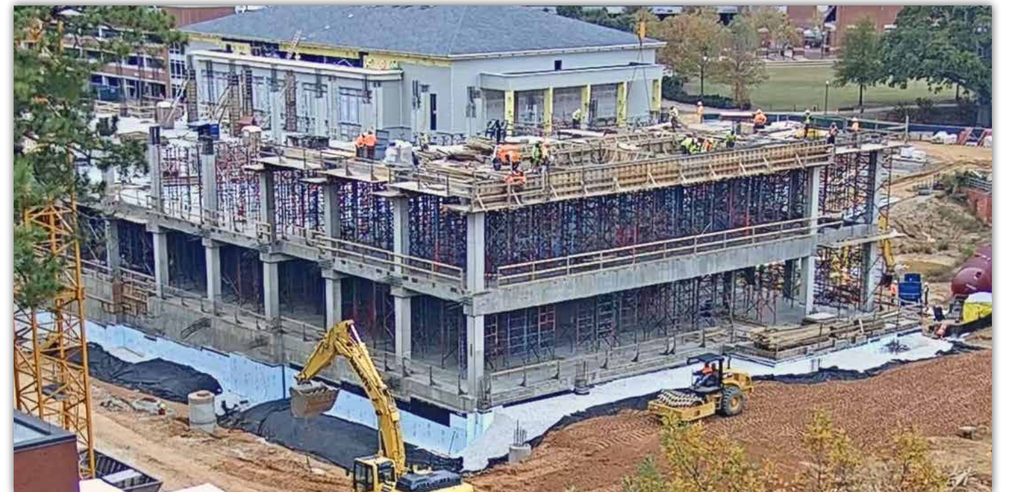
The east side of the ACLC as viewed from the Dudley Hall webcam. This shows a portion of the third floor construction currently underway.
