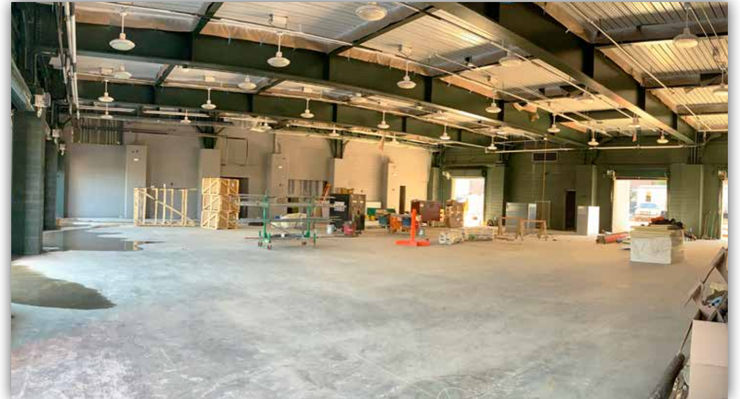
Painting and lighting installation continues inside the building. Artificial turf and batting cage netting will soon be installed.
