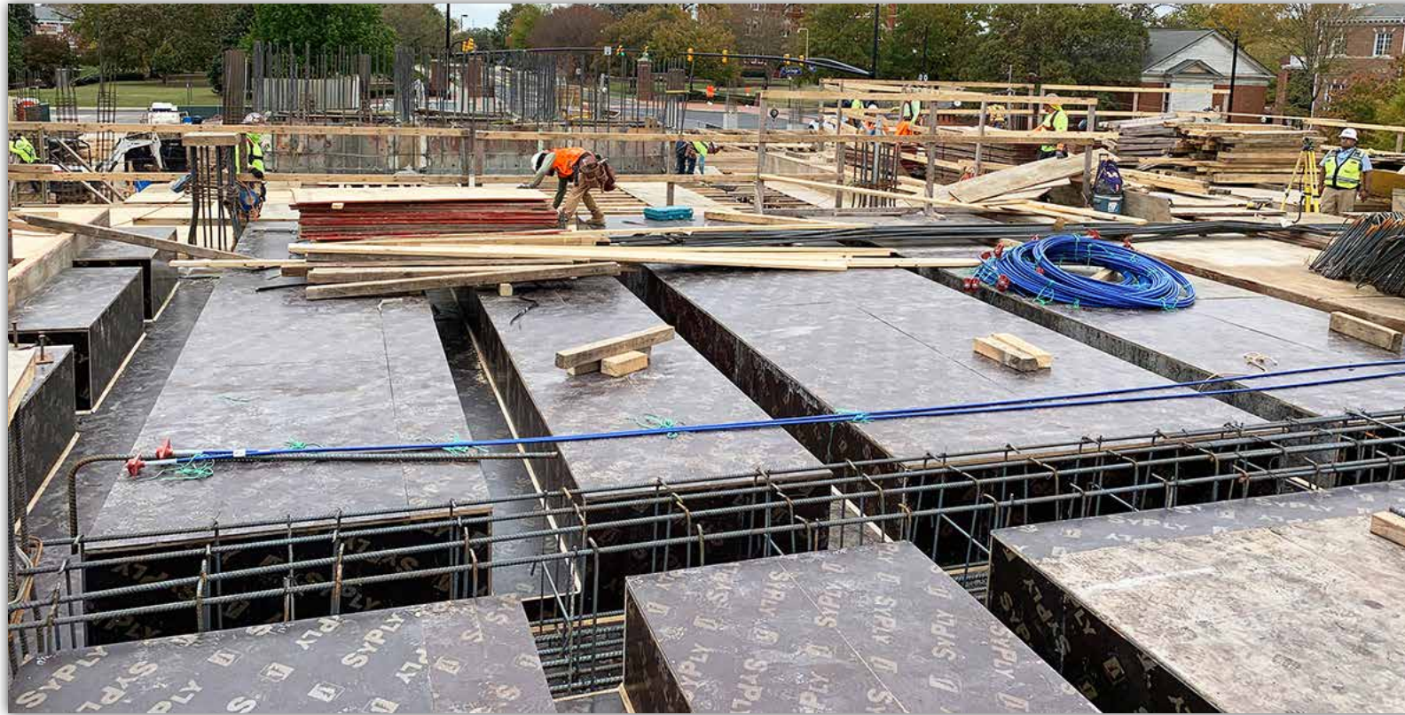
Elevated form work and rebar are being installed prior to the second floor concrete pour. Photo courtesy: Matt Jackson.
