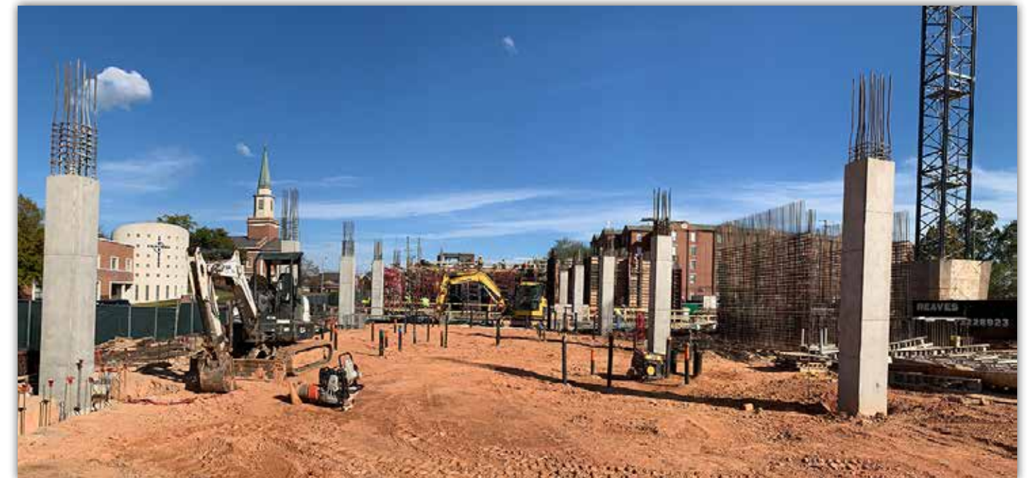
These concrete columns will support the second floor section of the building located at the intersection of South College Street and Thach Avenue.
