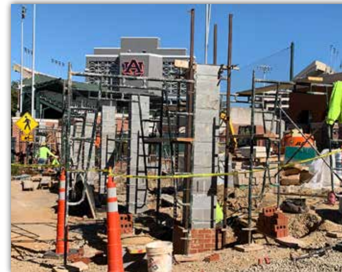
Concrete columns are being erected to support the new fence in front of the building.
