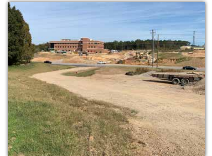
Work is underway on a new service road leading from Shug Jordan Parkway to the Swine Unit.
