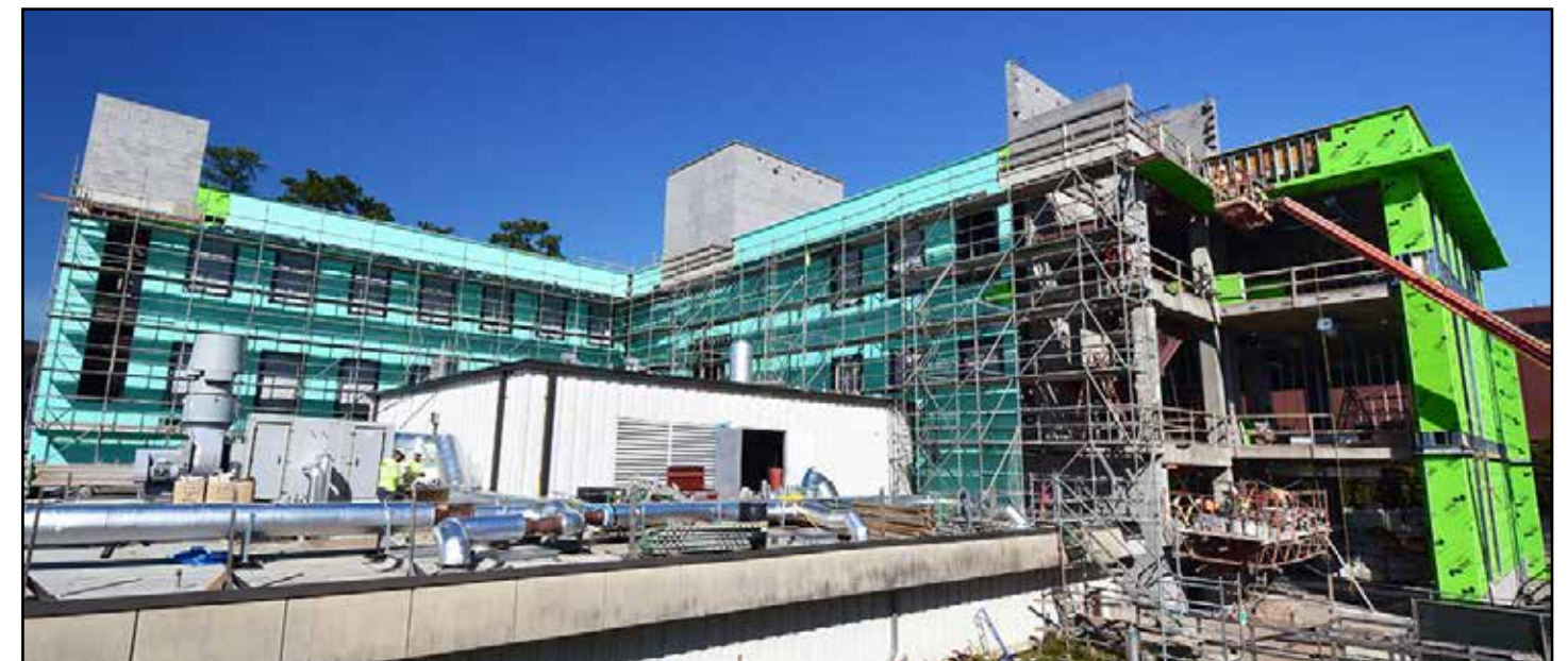
This view shows how the new addition connects to the original portion of the Leach Science Center.
