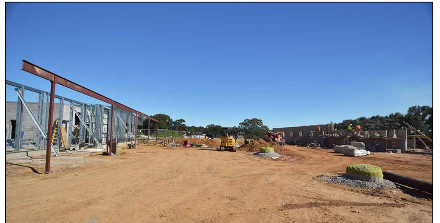
The equestrian team's support building and barn are being built adjacent to one another.
