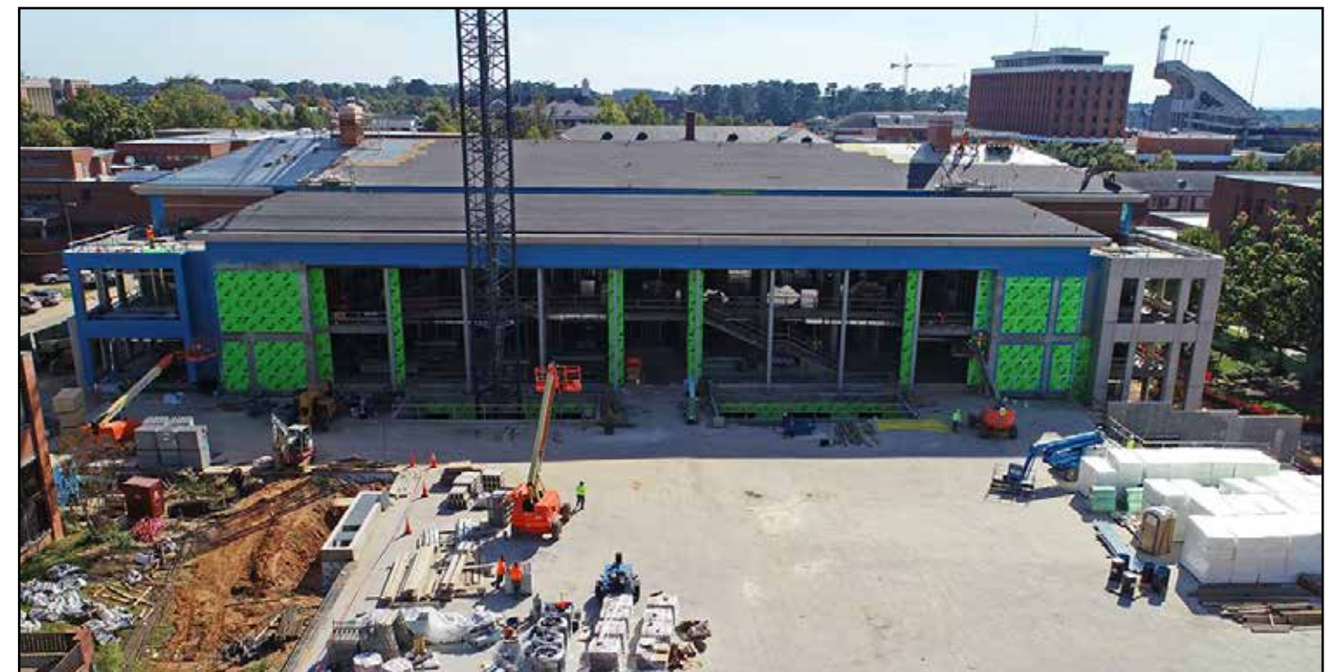
A frontal view of the building with the future courtyard in the foreground.
