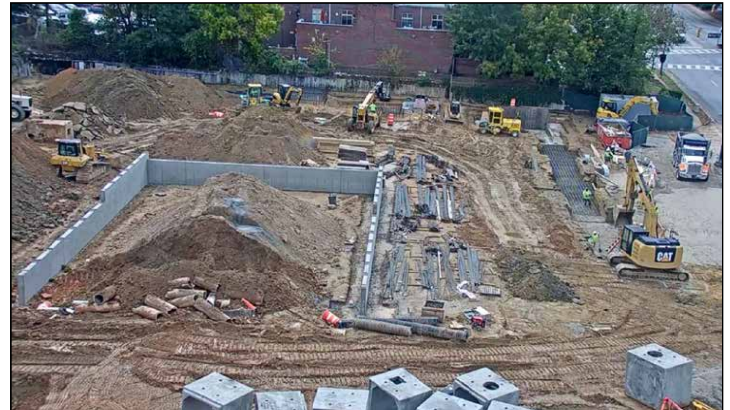
Concrete foundation walls for the ramps can be seen along with concrete culverts that, once installed, will help control rainwater during storms.
