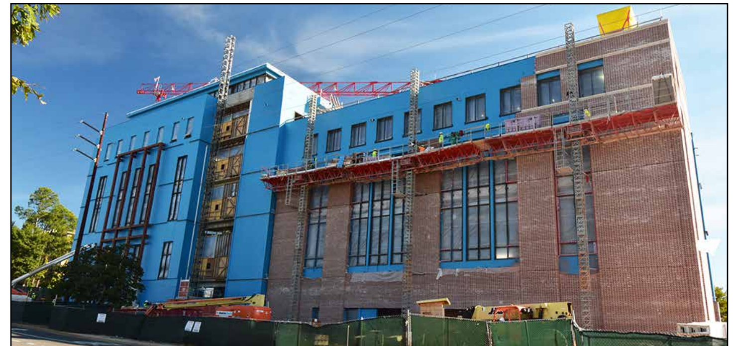
Brick installation can be seen from the South Donahue Drive side of the building.
