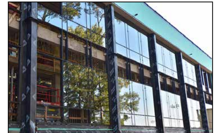
Window installation has begun on the north side of the building facing Jordan-Hare Stadium.
