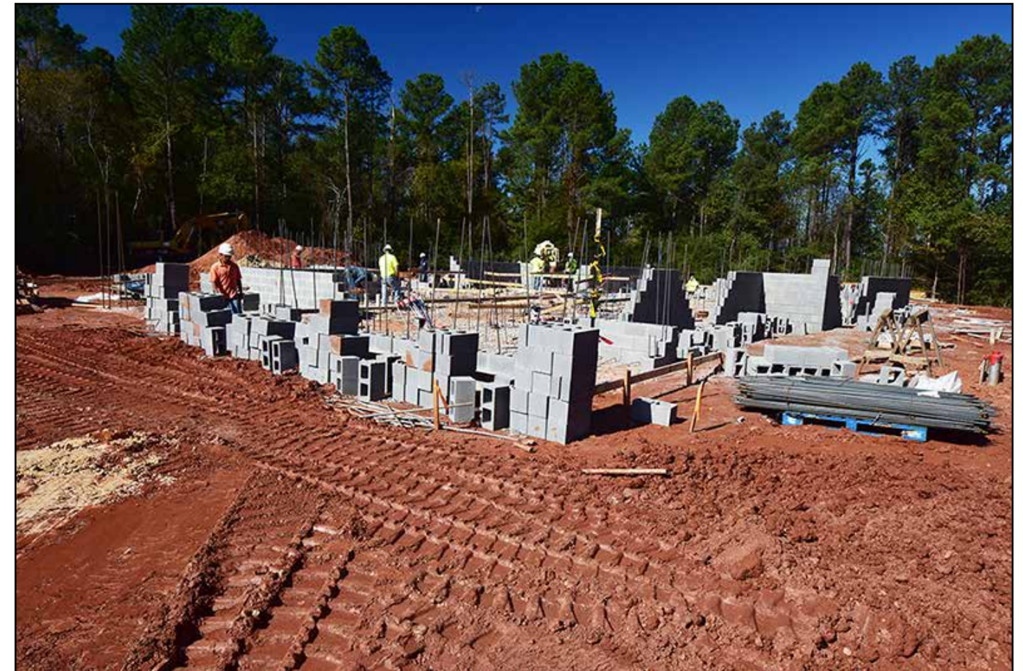
Concrete block walls can be seen going up at the Poultry Science Infectious Disease Lab construction site.
