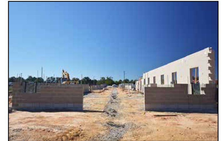
The barn's block installation begins to frame the four sides of the building.
