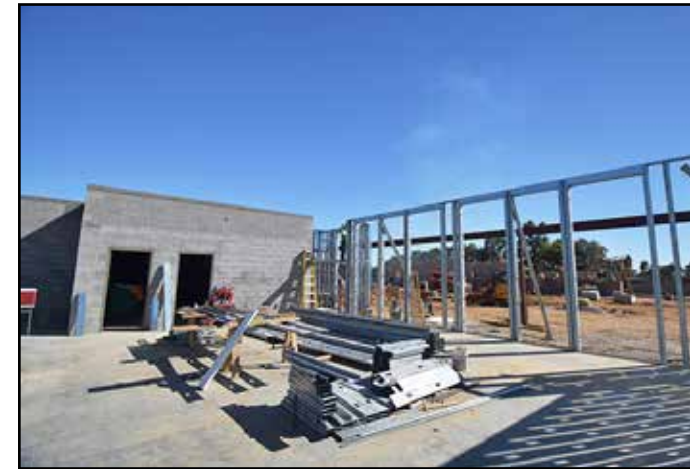
Metal studs, used to build the walls, are ready to go up inside the support building.
