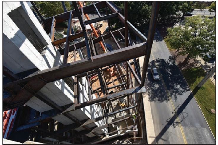
A view of the elevator shaft and stairwell frame facing South Donahue Drive.
