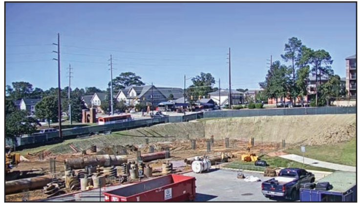
A view of the construction site from the Graduate Business Building webcam.
