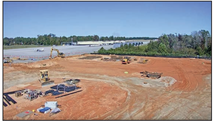
A view of the Airport Aviation Education Facility from the project webcam.
