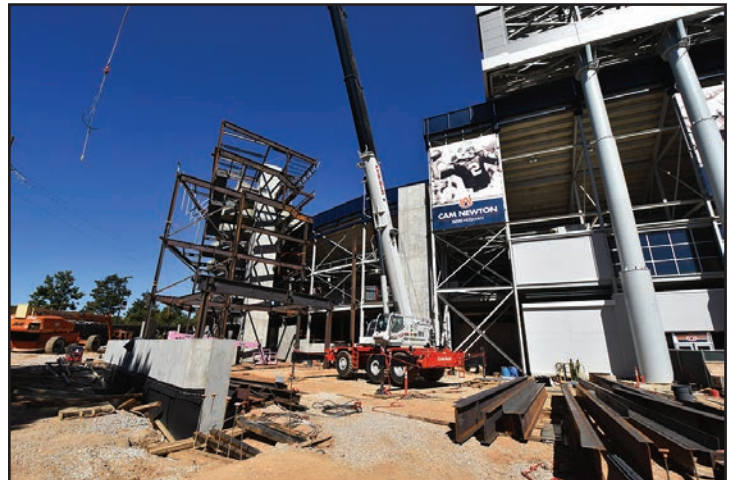
A view of the site and structural steel that will soon be installed.
