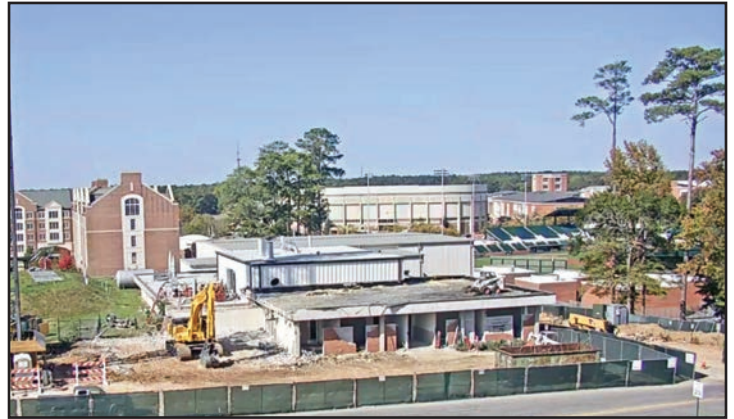
Demolition of the existing brick section of the Leach Science Center has begun.
