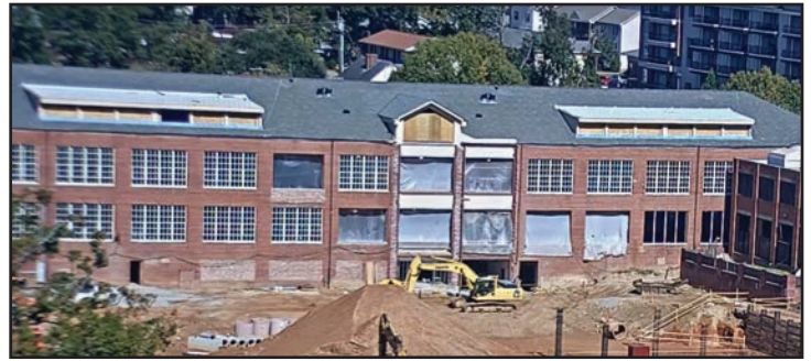
Construction of the new roof dormers and gable (center) are well underway.
