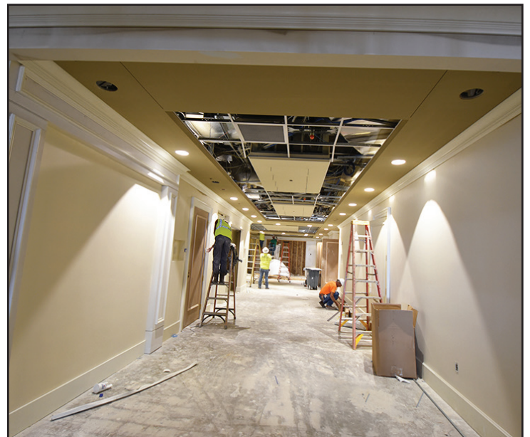
Carpet and ceiling tile installation will soon be complete in the main hallway.
