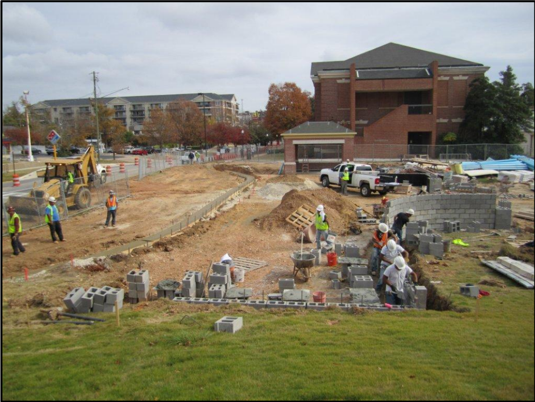
Tiger Concourse and Ginn Plaza – Magnolia Street Transit Bus Drop Off—Looking East
