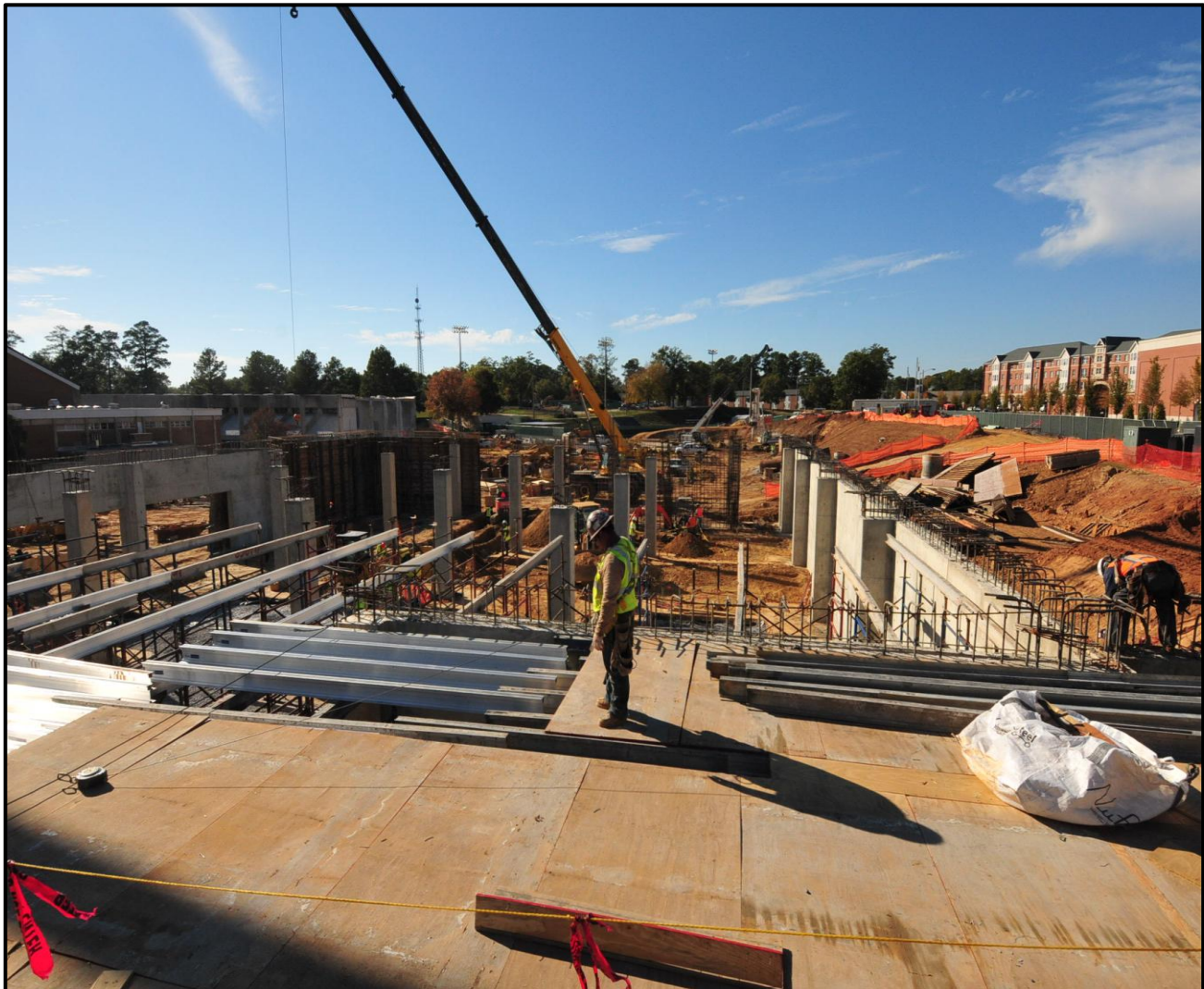
AU Recreation and Wellness Center – View of Elevated Slab, Foundation Walls, and Columns
