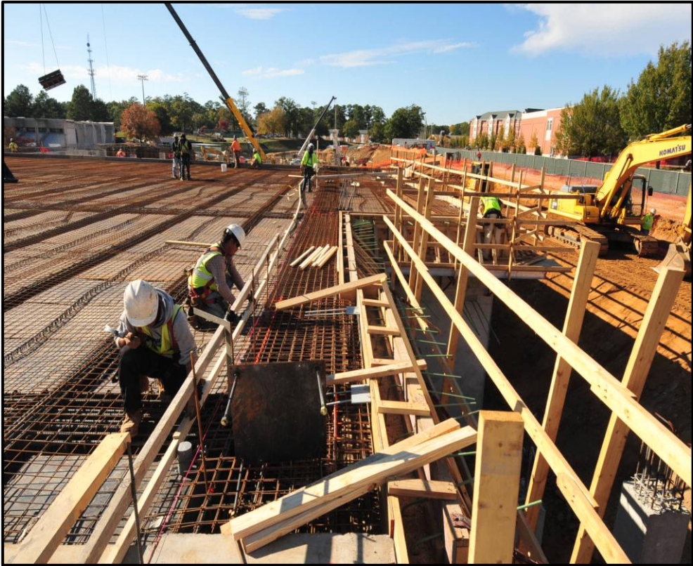
AU Recreation and Wellness Center – Preparation of Elevated Slab for Concrete Pour
