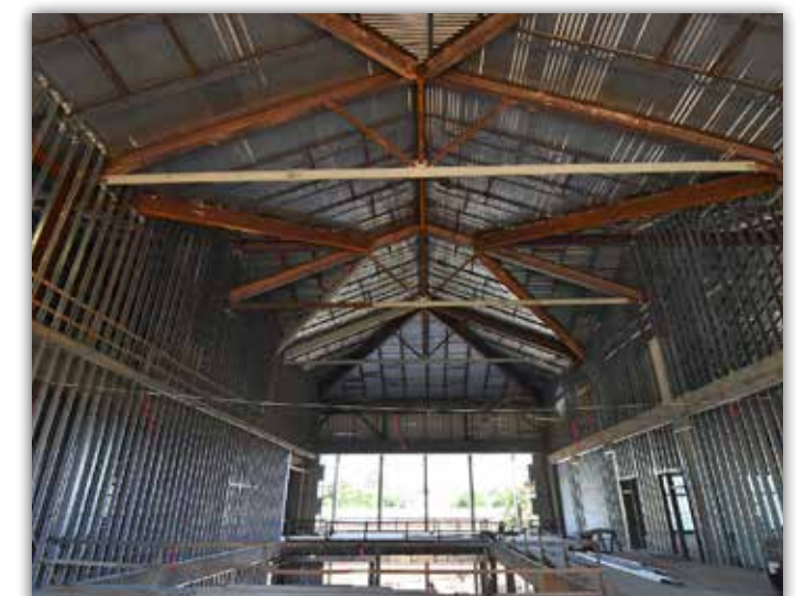
West atrium framing is complete. Overhead piping and duct work installation will start next.
