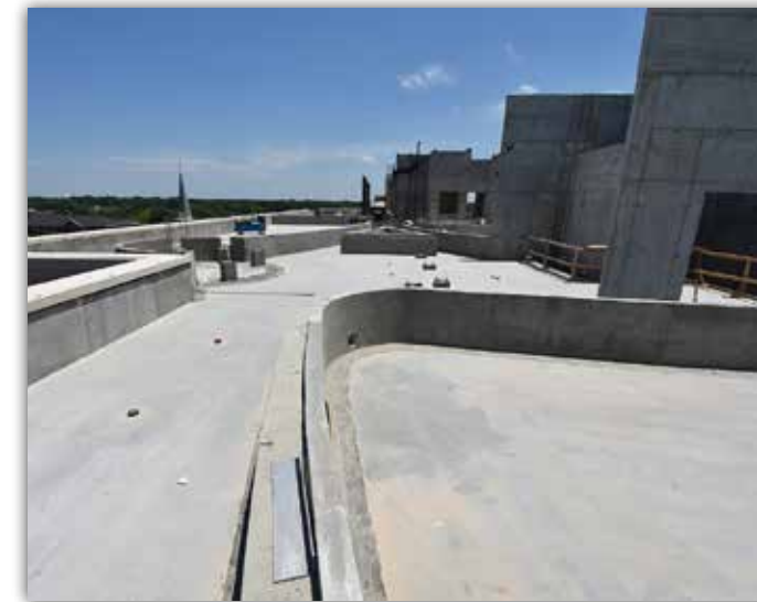
Concrete form work nears completion for the rooftop terrace and pool area.
