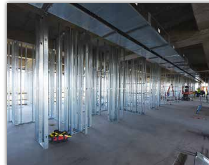
Interior framing is ongoing on level four, which will enclose the hotel guest rooms and suites.
