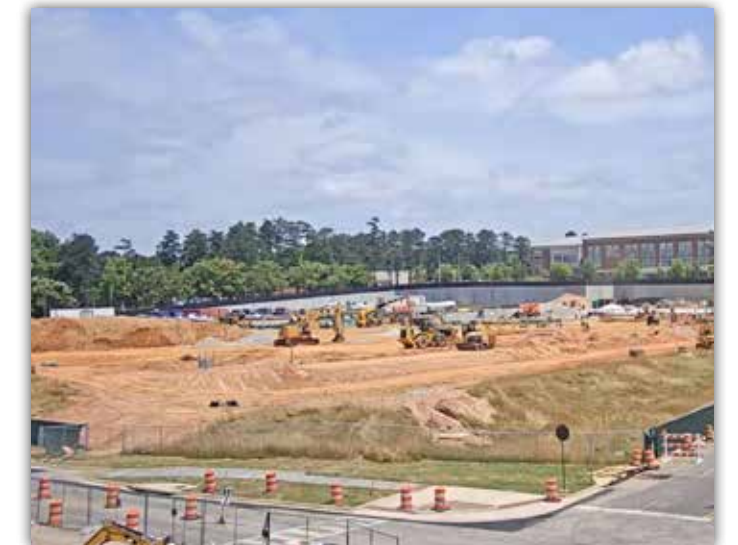
A webcam view of the site shows how busy contractors are preparing the grounds for upcoming foundation work.
