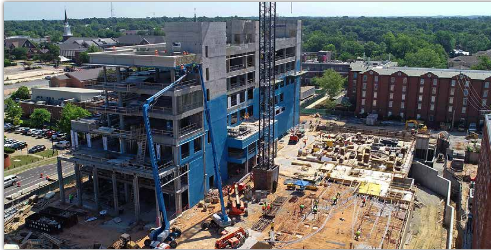
The Tony and Libba Rane Culinary Science Center's concrete structure has reached the rooftop level.
