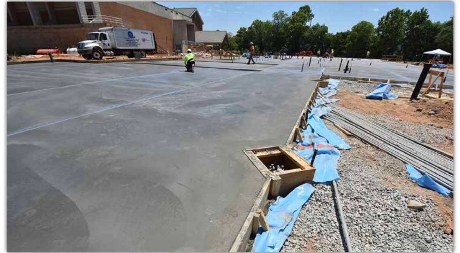
The concrete foundation for the locker room, equipment storage and main utility areas has been poured.
