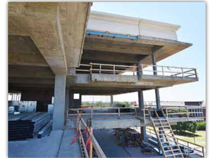
Interior metal frame work will soon begin for each of the condos.
