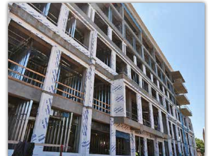
The portion of the building facing north, with architectural features and balconies protruding towards East Thach Avenue, is framed and waterproofed.
