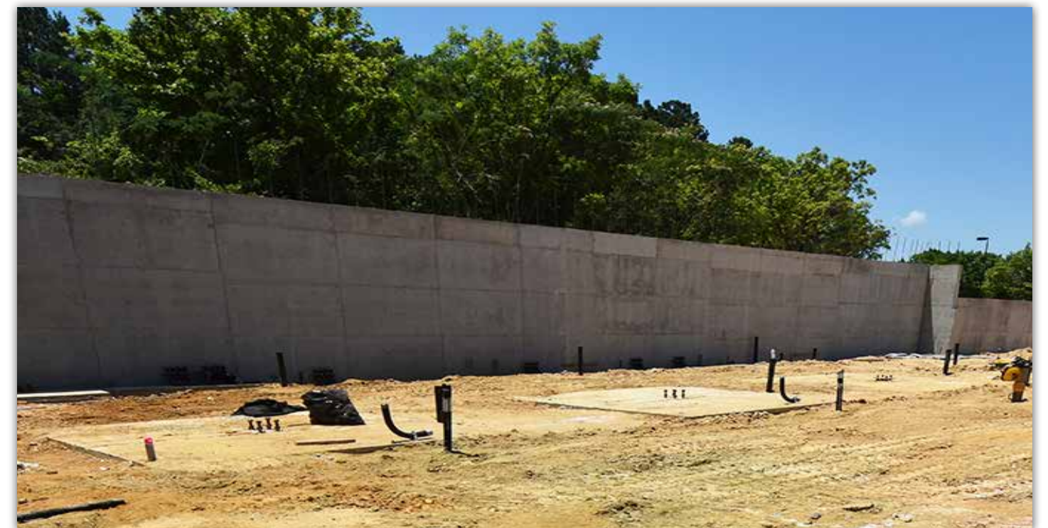
These concrete squares on the ground are the foundations for structural columns.
