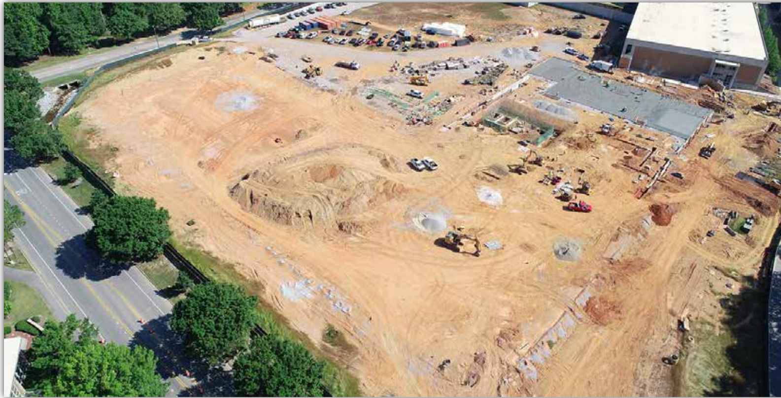
An aerial view of the Football Performance Center shows where utility work continues and the concrete foundations are being poured.
