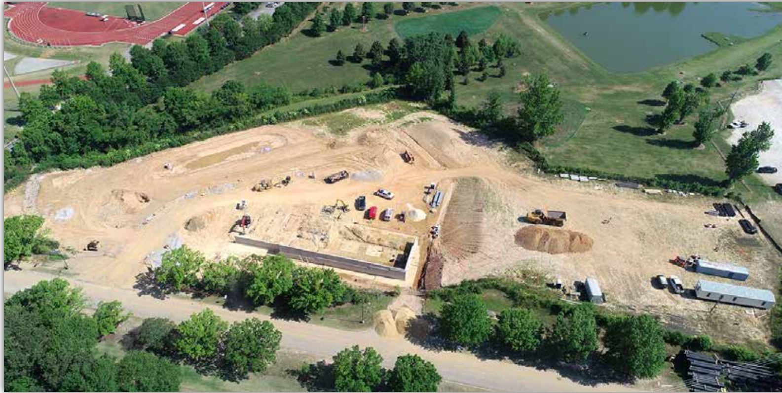
An aerial photo of the Chilled Water Plant site. The first concrete walls are starting to go up.
