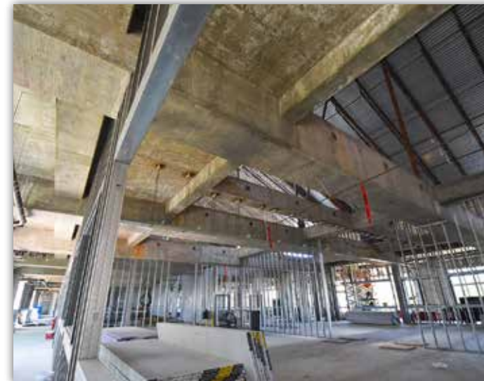
Interior metal framing is complete. Mechanical, electrical and plumbing installation will follow overhead and in the wall.
