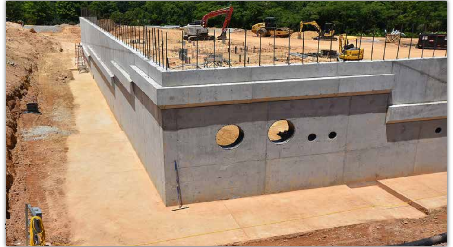
The first floor retaining wall has been poured in place with holes cut out for the hot water and chilled water piping.
