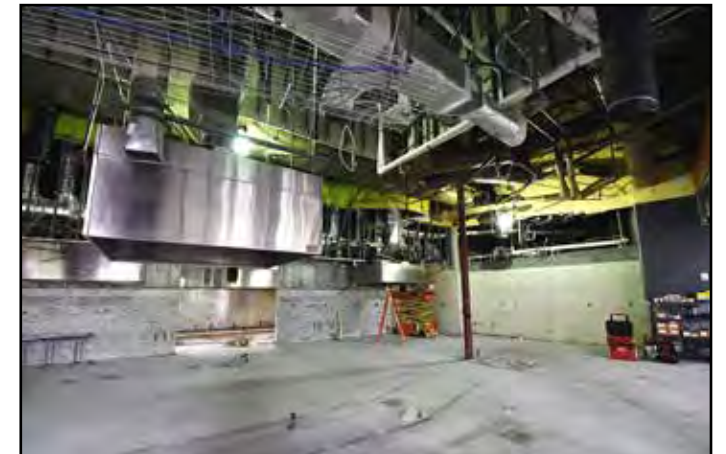
The food preparation area is ready for the new construction to begin.
