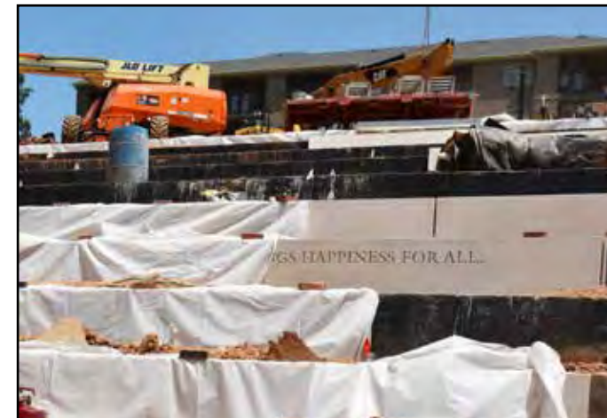
Construction of the seat wall continues with installation of precast materials that include the Auburn Creed.
