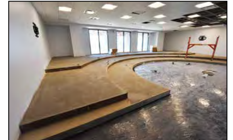
A plastic cover protects carpet that has been installed in the case study classroom.
