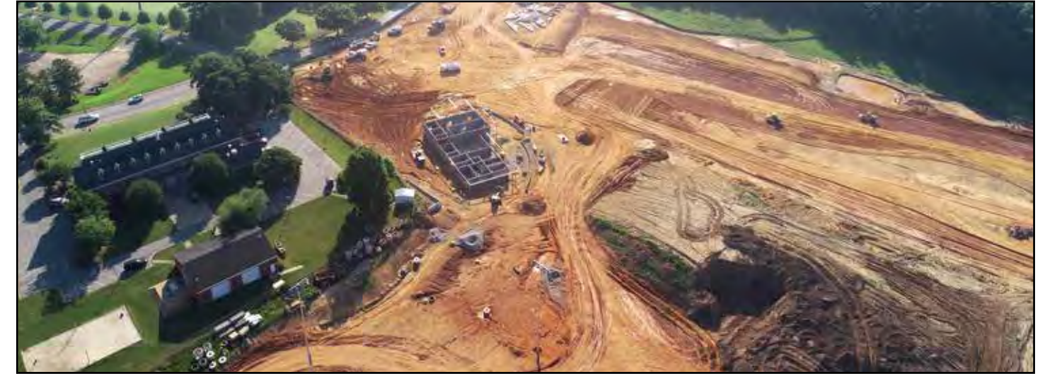
A view of the site looking toward Lem Morrison Drive shows the parking lot area and construction of the field house.
