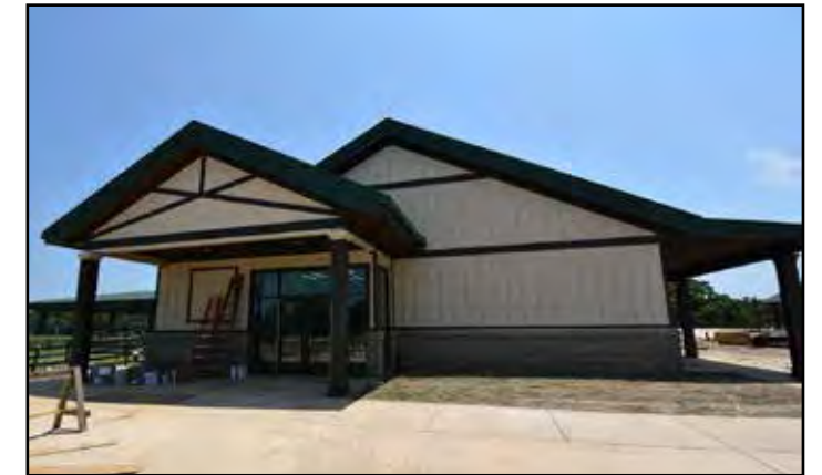
Final touches are being placed on the outside of the team support building.
