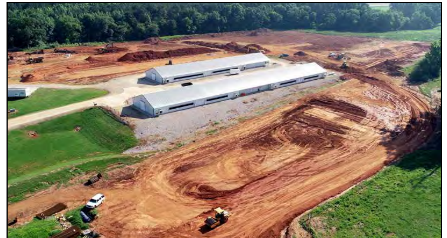
Site work continues for the pen-houses, hatchery, breeder house and ancillary buildings.
