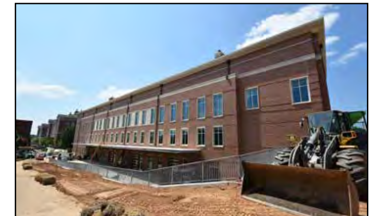
The back of the building, which faces Foy and Tichenor halls is ready for landscaping.
