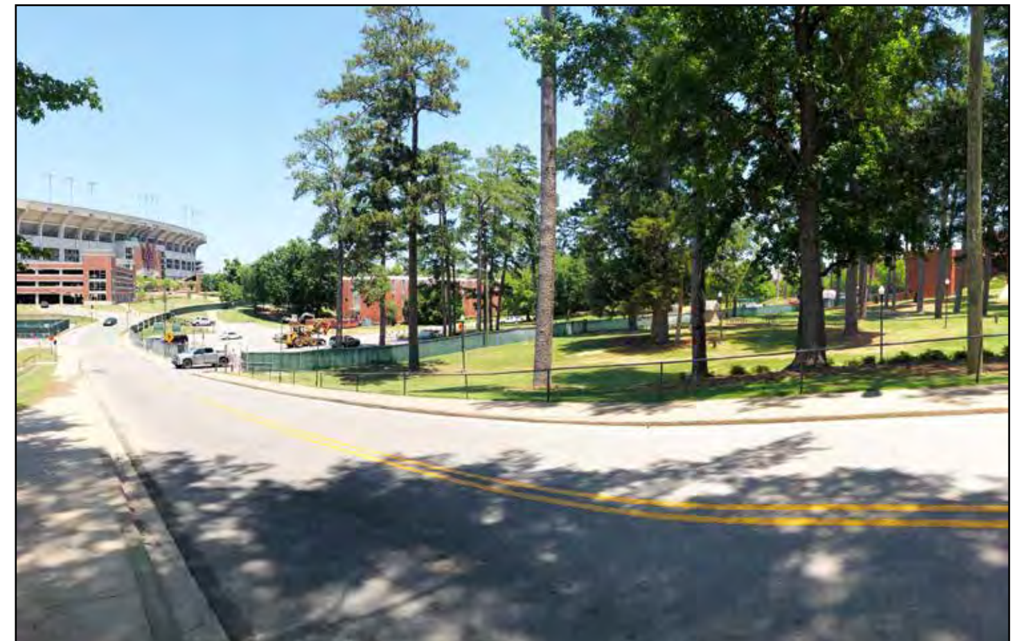
Construction fence is being installed around the project site in preparation for the demolition of Allison Laboratory.
