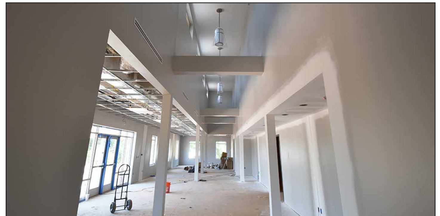
Interior work on the center continues as doors and windows are being installed.
