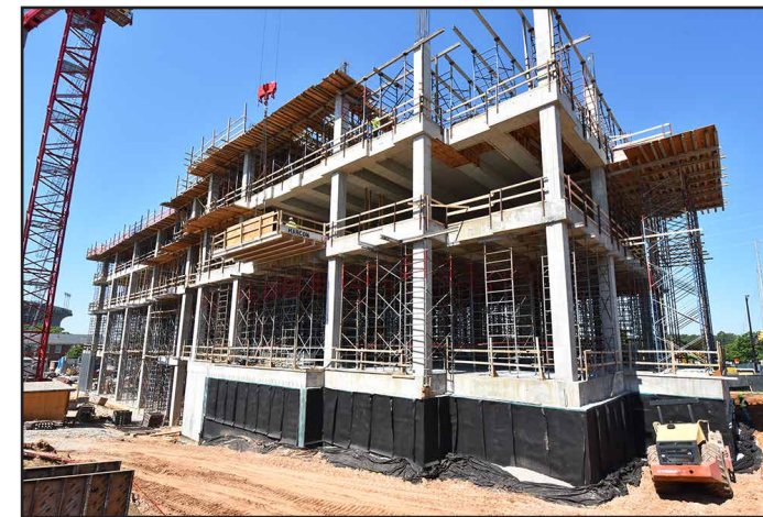
A designated safe room sits at the bottom of the building, surrounded by concrete.
