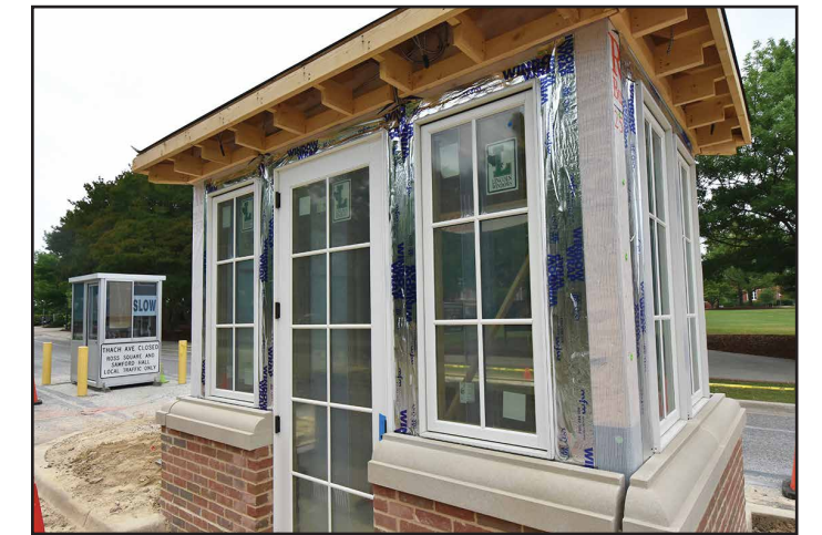
The welcome kiosk is nearing completion and is much more spacious than the previous kiosk.
