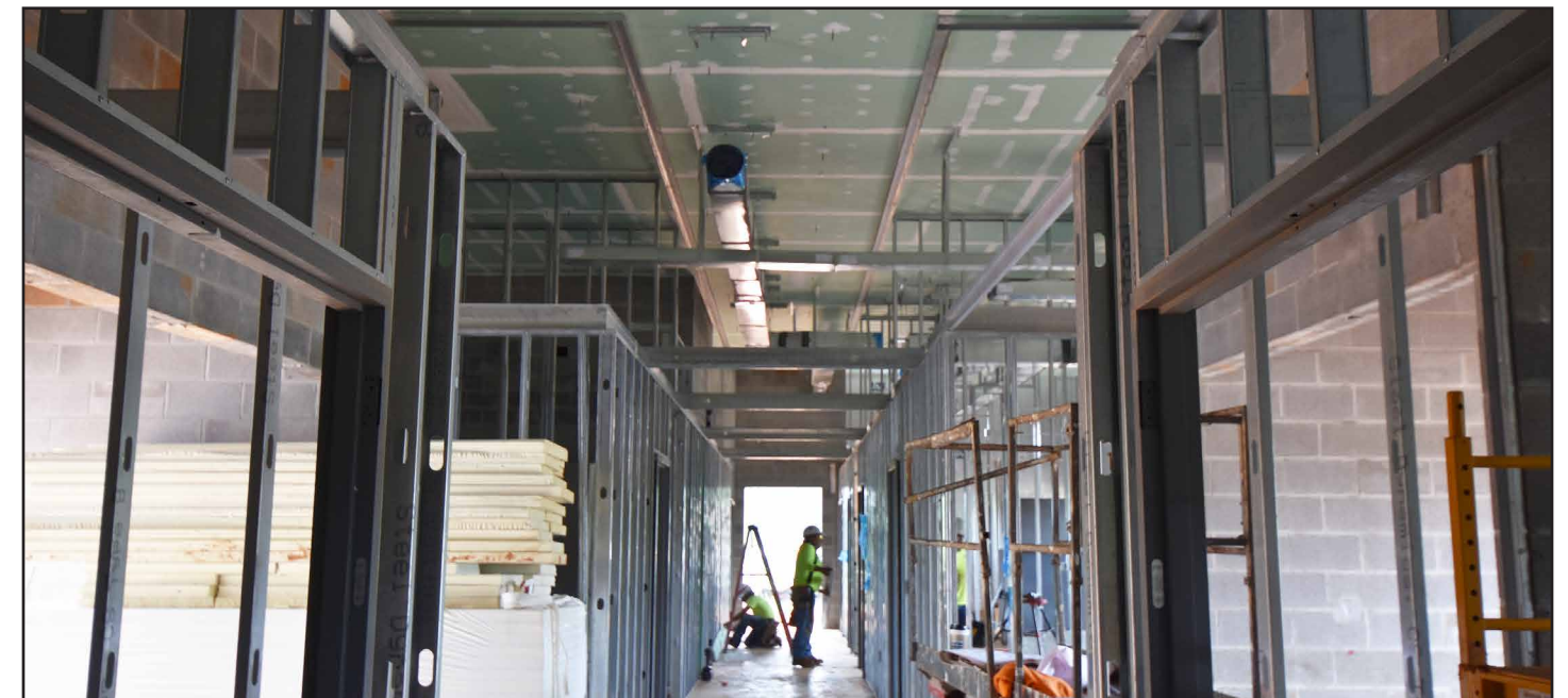
Drywall has been placed on the ceiling of the main hall, as well as metal framing for future rooms.
