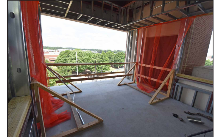
Front elevator access work continues at the rear of the press box area.
