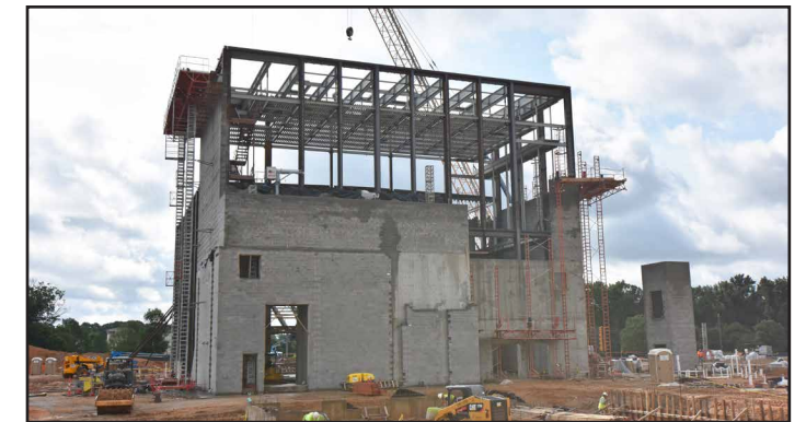
The erection of the structural steel for the stage "fly tower" is nearing completion.
