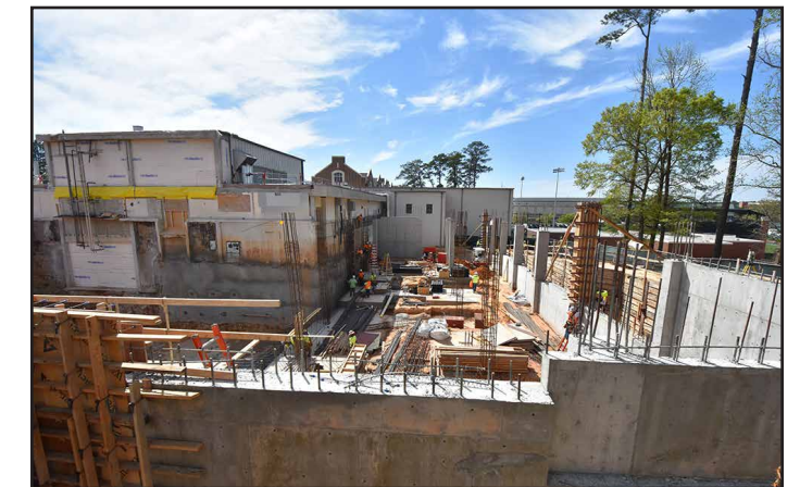
This project involved a major excavation of three sides of the existing building.
