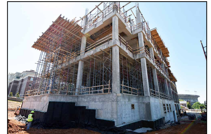
The back view of the building as structural work continues on the inside and outside.
