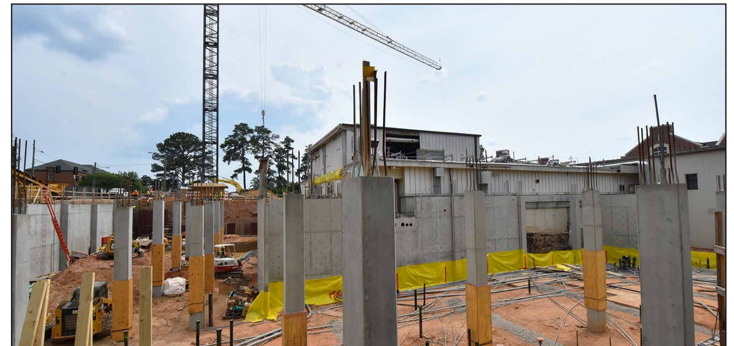
Concrete columns have been poured for the south end of the new addition's basement.
