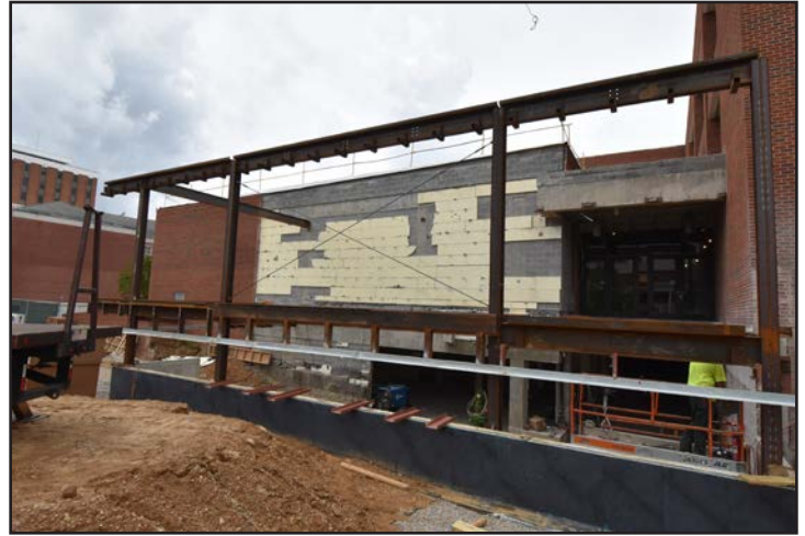
The original entrance has been removed, and structural steel is being erected.
