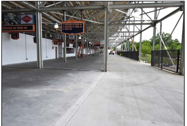
Looking west, the area to the right is the new concourse expansion.
