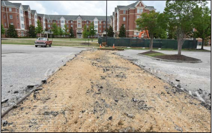
Utility work is in progress in the parking lot located south of Campus Safety.
