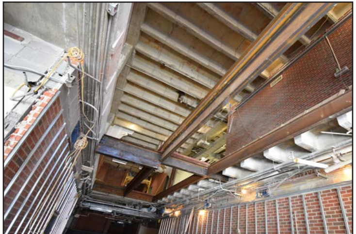
View from ground floor to first floor of the steel structure being erected.
