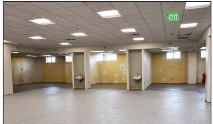
Installation of vinyl flooring in the lab area of the north building has begun.
