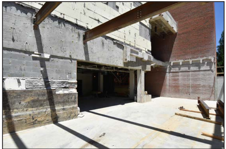
View of ground level exterior construction where a wall has been removed.
