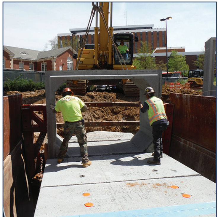
Crews install a portion of the box culvert under the north end zone parking lot.
