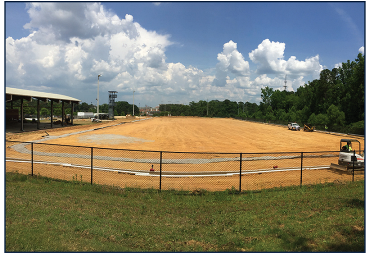
Earthwork and field drainage installation of the artificial turf field is underway.
