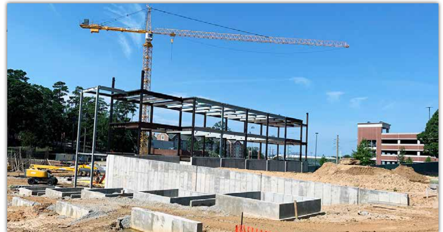
Tiered steps and a walkway are being formed, which will lead to a courtyard between the Central Dining Hall and ACLC.
