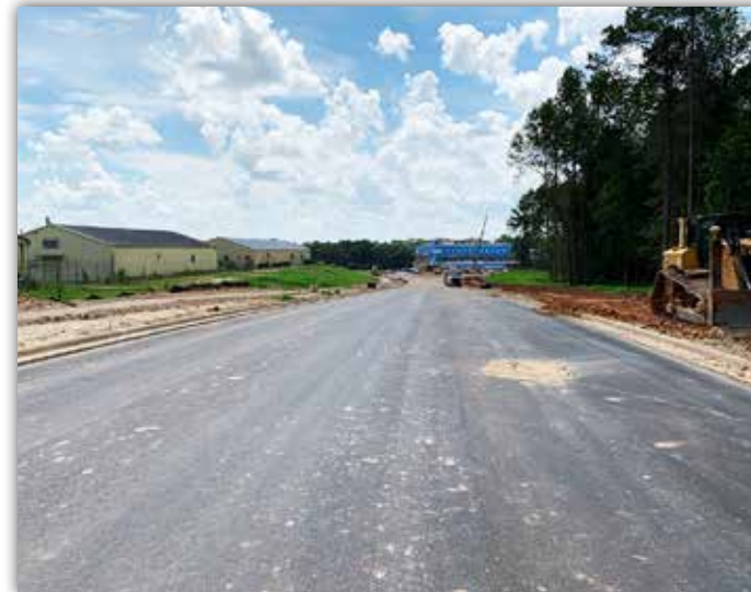
The first layer of asphalt has been applied to the new road up to where the traffic circle begins.
