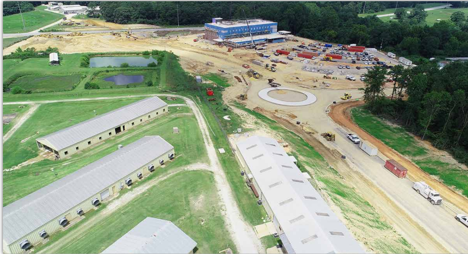
An aerial view of the project shows how Camp Auburn Road will extend past a new traffic circle and on to Shug Jordan Parkway.
