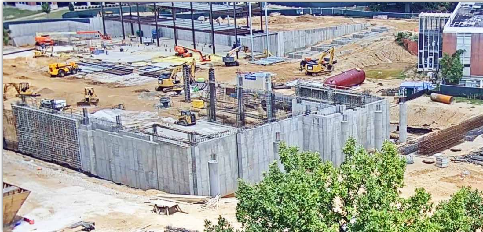
A view from the ACLC webcam gives a picture of the basement concrete wall construction to date. Watch construction live at https://aub.ie/SDR3nb .
