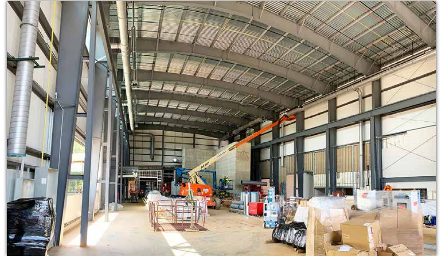
The interior of the testing laboratory is busy with ongoing wall framing, and electrical and mechanical installations.
