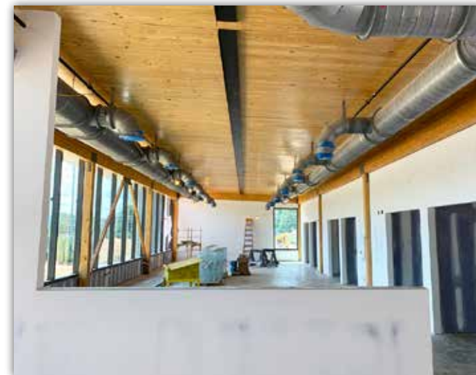
The windows and wood ceiling have been installed in the administrative area.
