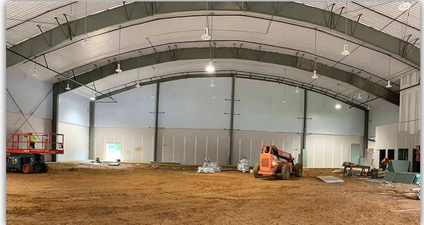
Preparations are being made, inside the building, for installation of the turf field.
