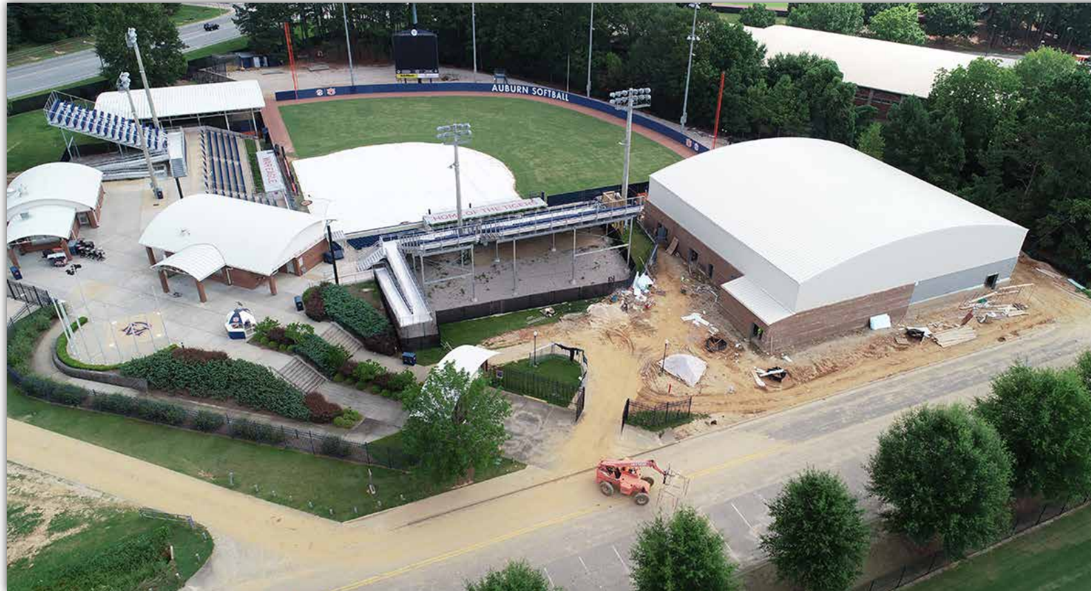
This aerial photo shows where the new building is located just adjacent to the Jane B. Moore Softball Complex. The exterior framing is complete and brick installation is ongoing.
