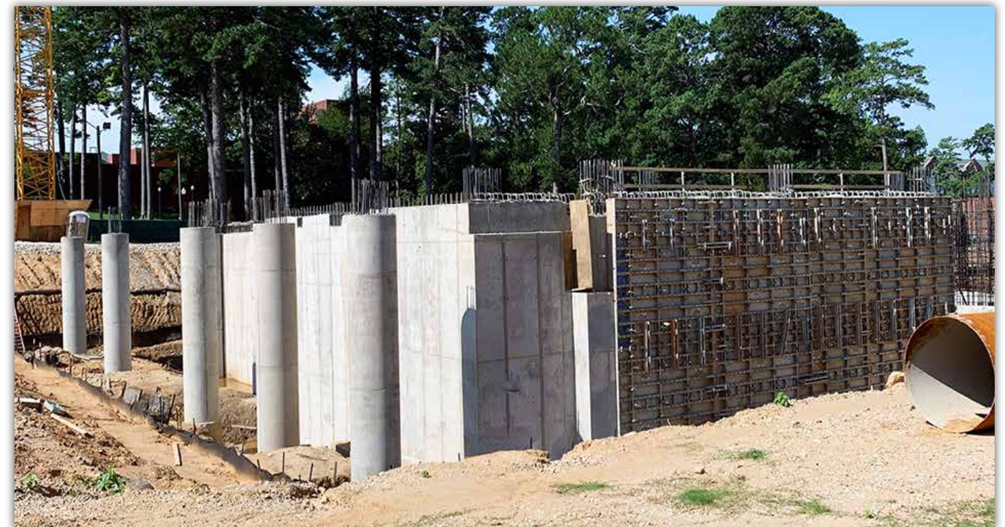
These five free-standing round piers will support columns on the upper levels of the building.
