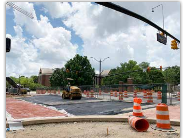
Installation of new curbing and sidewalks has moved to the East Thach Avenue side of the intersection.
