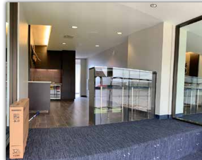
New carpet has been installed. Anchor bolts are in place for the new tiered fixed seating.
