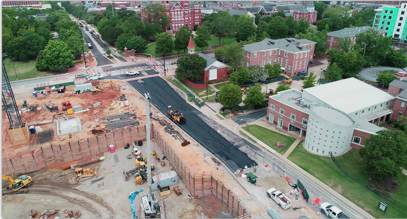
Paving of East Thach Avenue is now complete, while paving of West Thach Avenue is ongoing.
