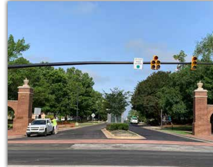
West Thach Avenue has been repaved following installation of underground power and water piping.
