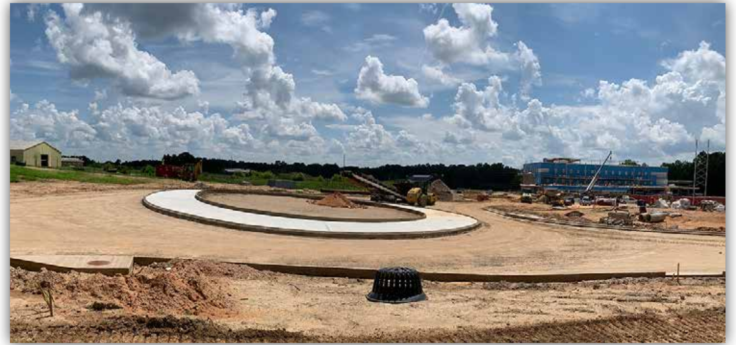
The traffic circle has been formed. Next steps include putting down the first layer of asphalt.
