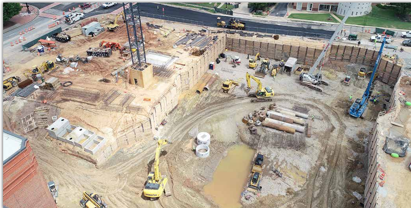
Retaining wall work is ongoing for the basement (located on the right side of the photo).
