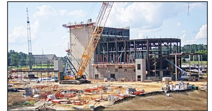
Structural steel work on the front of the house is almost complete.
