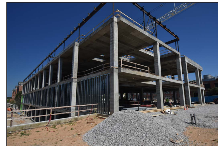
Exterior metal wall framing is beginning to take place on the east side of the building.
