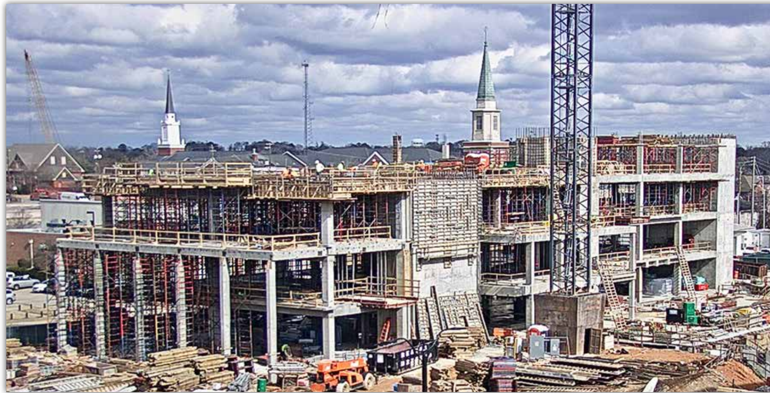
The Tony and Libba Rane Culinary Science Center's concrete structure is continuing to rise vertically. As seen in this image from the RBD Library, the structure is continuing with the fourth level out of six total.
