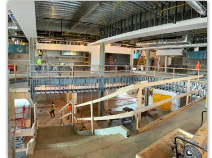
Kitchen equipment is being installed in the second floor food venues that surround the monumental staircase.
