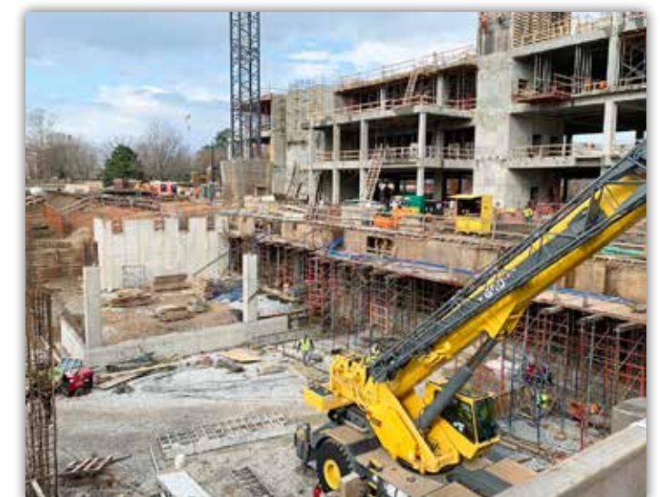
Framing continues for the underground loading dock, where future deliveries will be made to support the entire facility.
