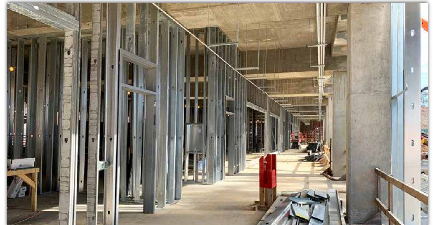
Metal framing installation is making good progress on the first floor inside ACLC.
