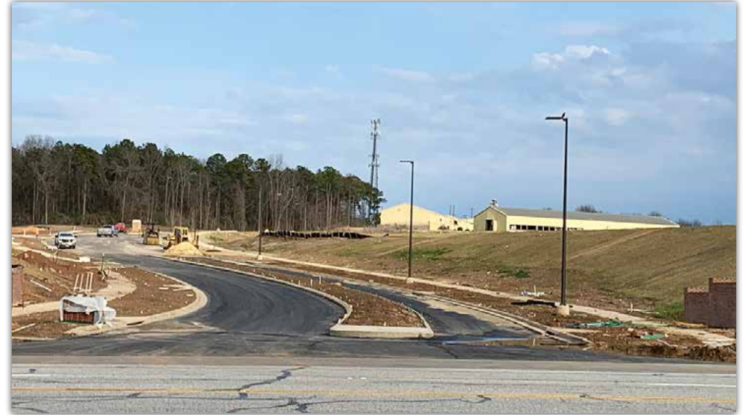
Curbing and sidewalks are complete at the Shug Jordan Parkway entrance. Landscaping will begin soon.
