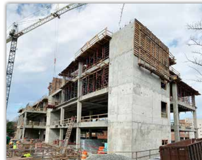
Construction at the Laurel Hotel's first floor entrance will soon have framed interior walls to delineate the hotel entrance from the rest of the culinary center.
