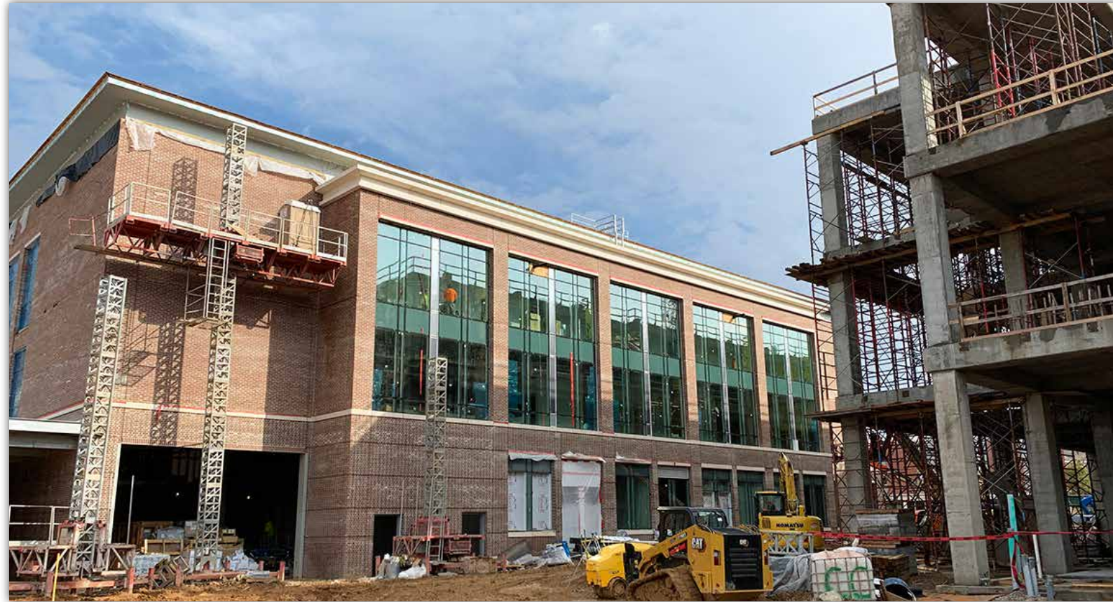
Brick work is complete on the south facing side of the Central Dining Hall. Second and third story window installation is complete.
