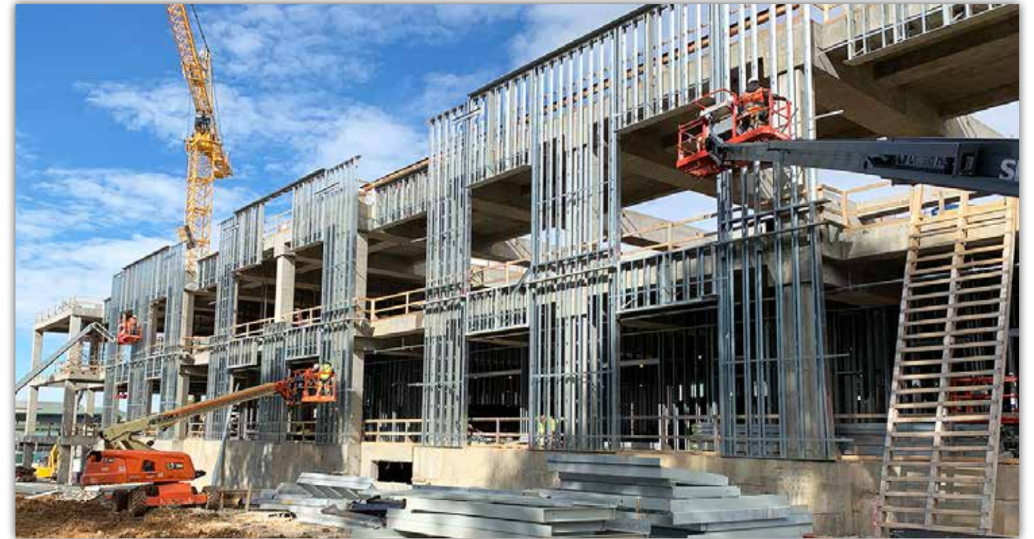
Metal framing is underway on the south facing side of the building.
