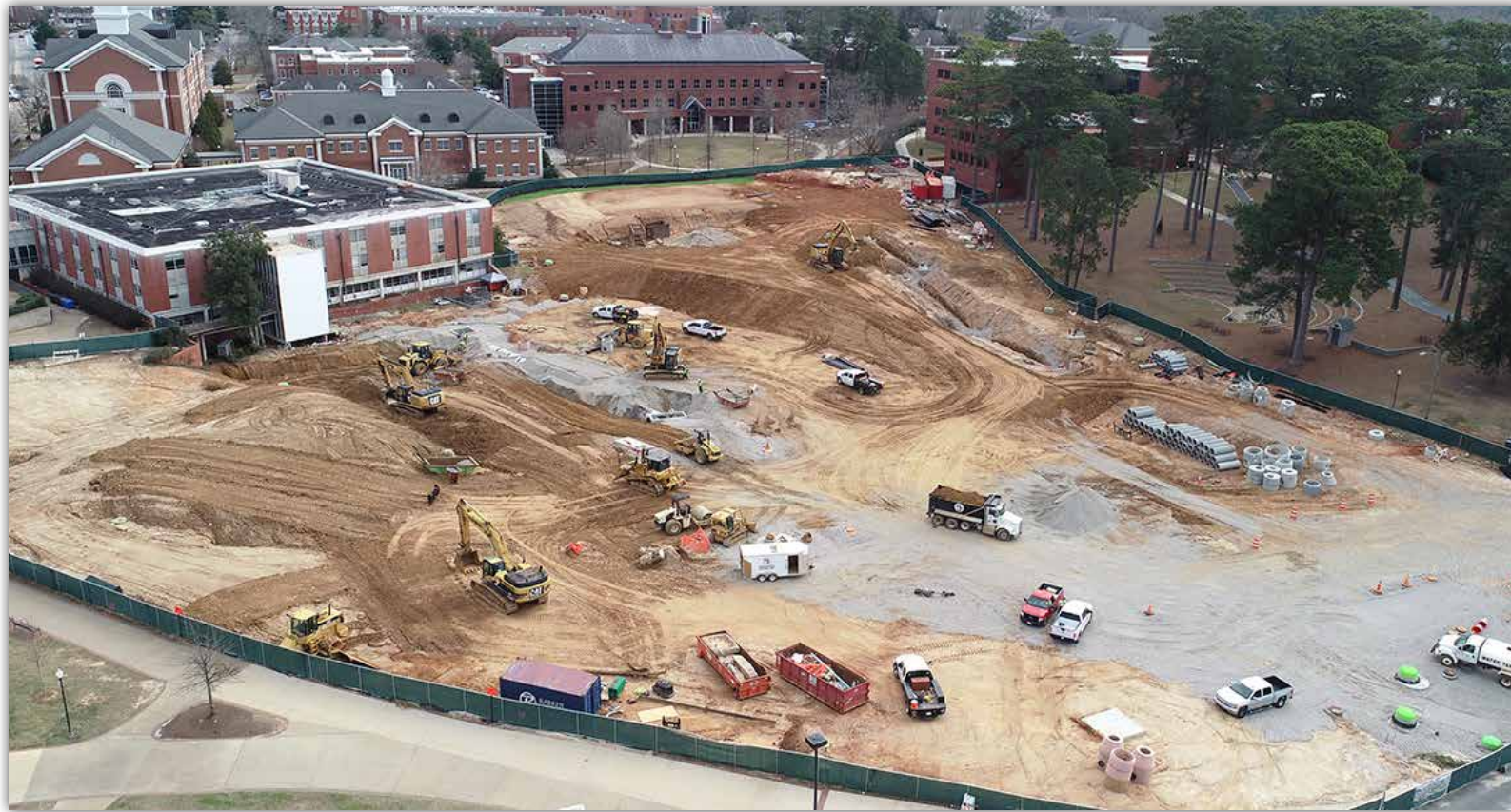
Installation of the stormwater drainage system and main electrical underground work is complete.
