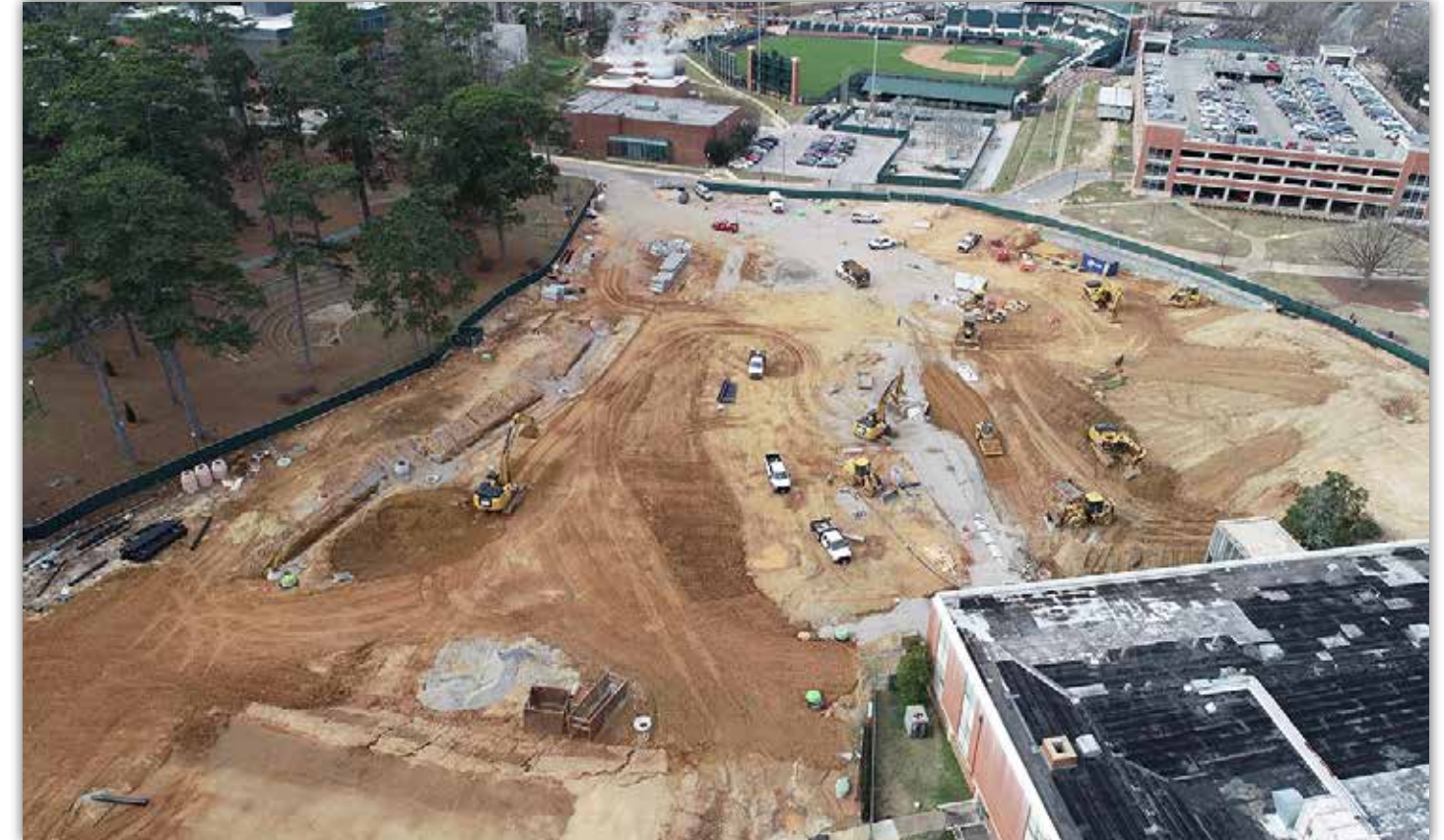
Earthwork is also underway to construct building pads for both the ACLC and Central Dining facilities. Phase II of the project, which is scheduled to begin in March, will include construction of the two buildings.
