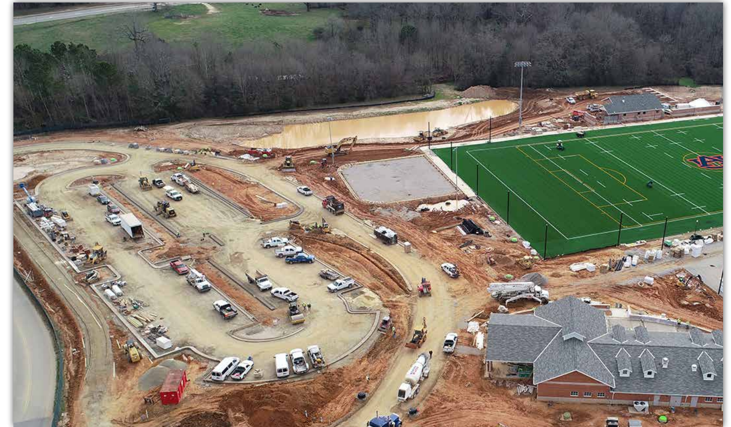
Concrete curbing is being placed for the parking lot. The fieldhouse is shown to the lower right.
