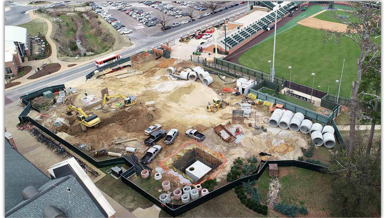
Installation of the stormwater drain system is underway at the AU Baseball player development site.
