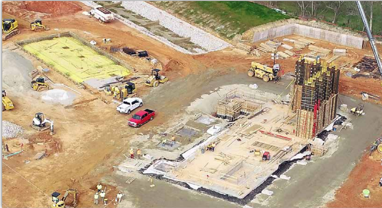
The yellow foundation in the top left is the beginning of the administrative section of the building. This section will connect to the testing laboratory portion of the new facility on the right.
