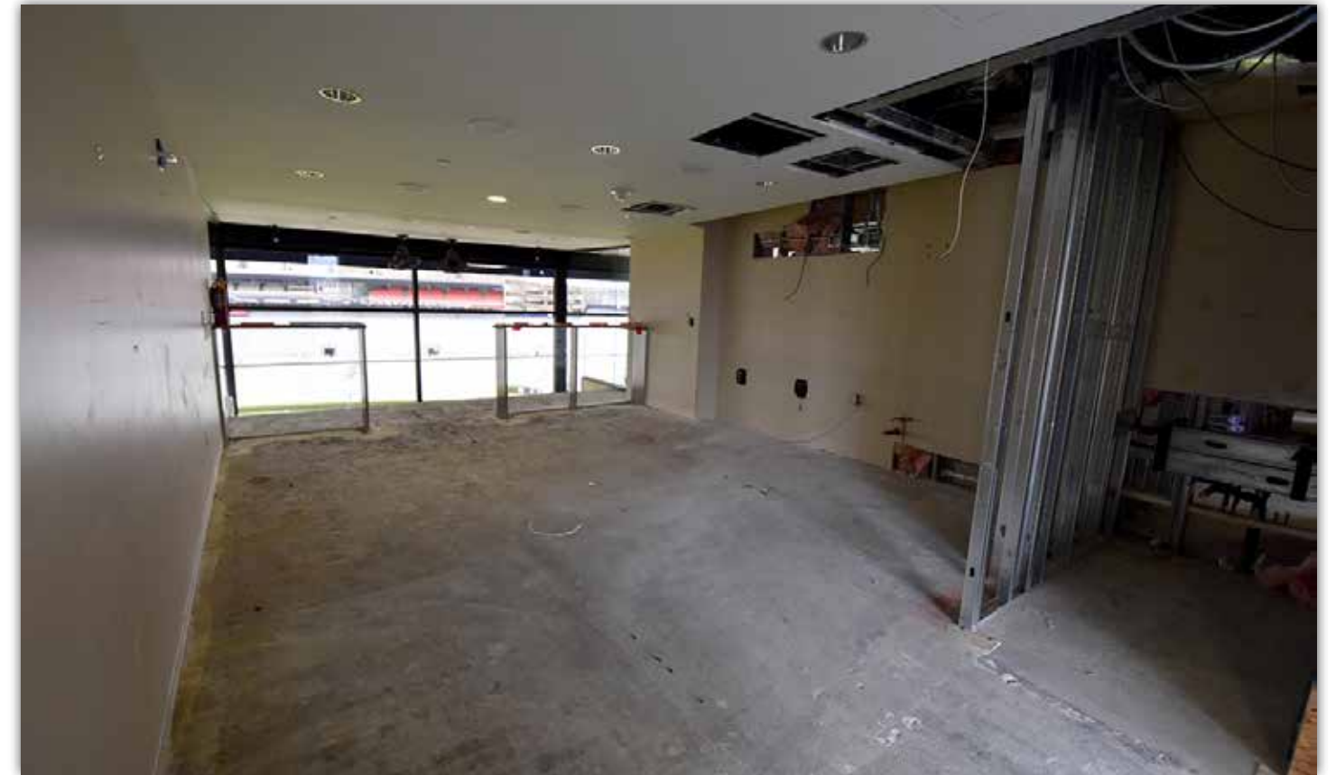
Demolition is complete in this suite, and construction of the new walls has begun.
