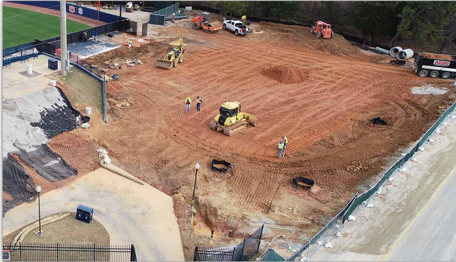
The site pad for the AU Women's Softball player development improvements project is nearing completion, which will allow concrete footings to be installed.
