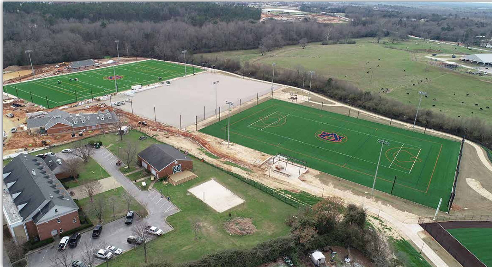
Four of the five new fields are complete - two softball, one soccer and one multipurpose . Construction of the remaining multipurpose field (the area in grey) is ongoing.
