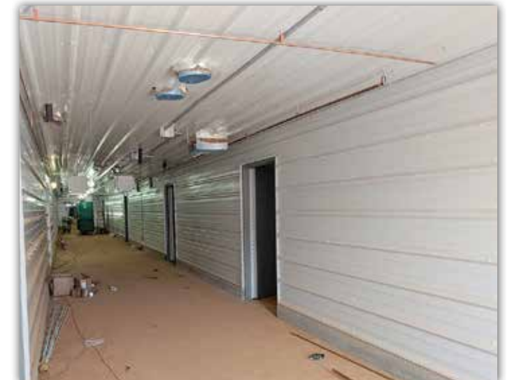
Interior view of the battery house, which will be used as a testing facility.
