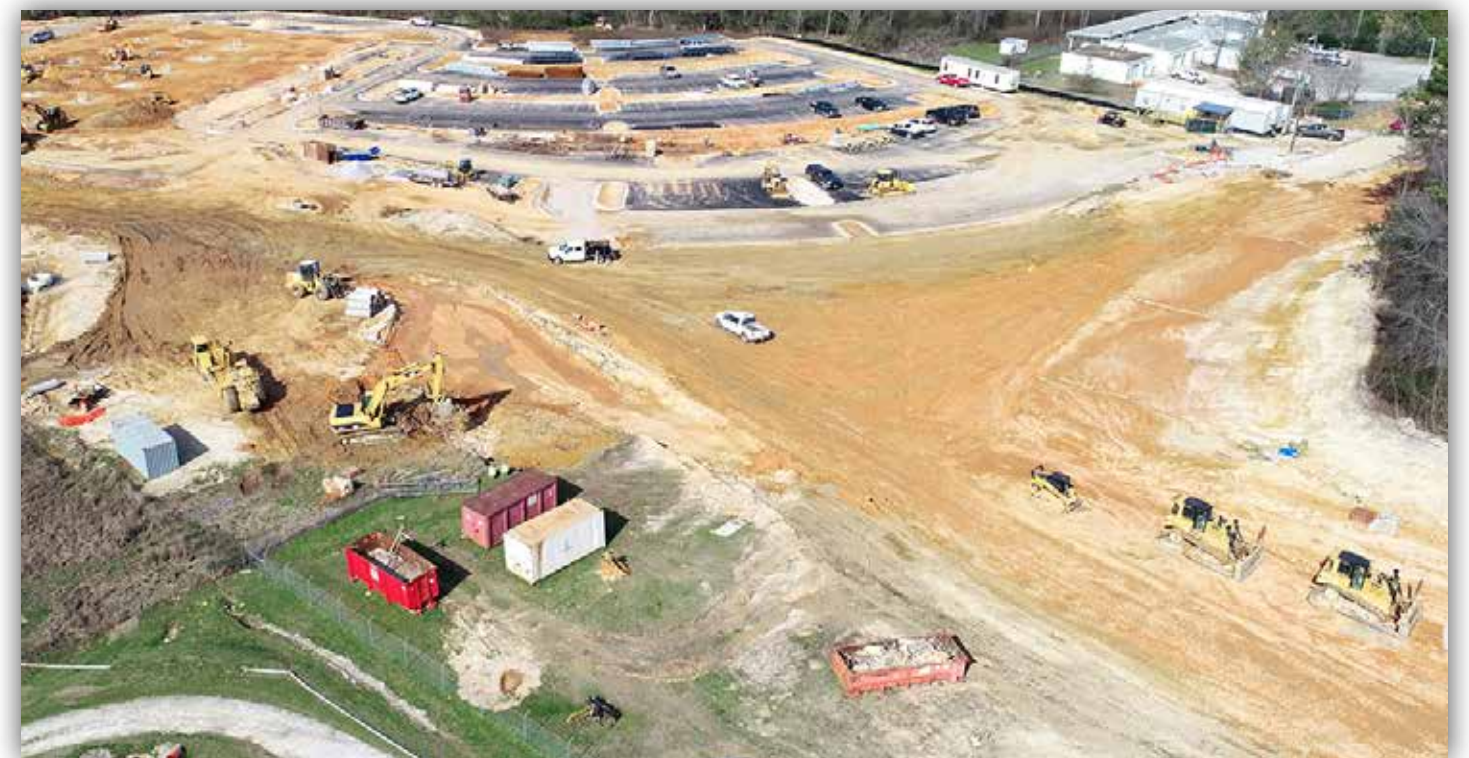
Grading has begun for the traffic circle (located in the center of this photo). The construction located in the top left corner of this photo is a separate project to build a Health Science Facility for the East Alabama Medical Center.
