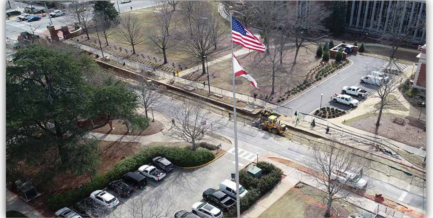
Installation of water and electrical utility lines has begun on West Thach Avenue near Ross Square.
