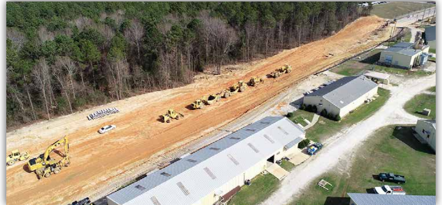
Road construction is underway to extend Camp Auburn Road to Shug Jordan Parkway.
