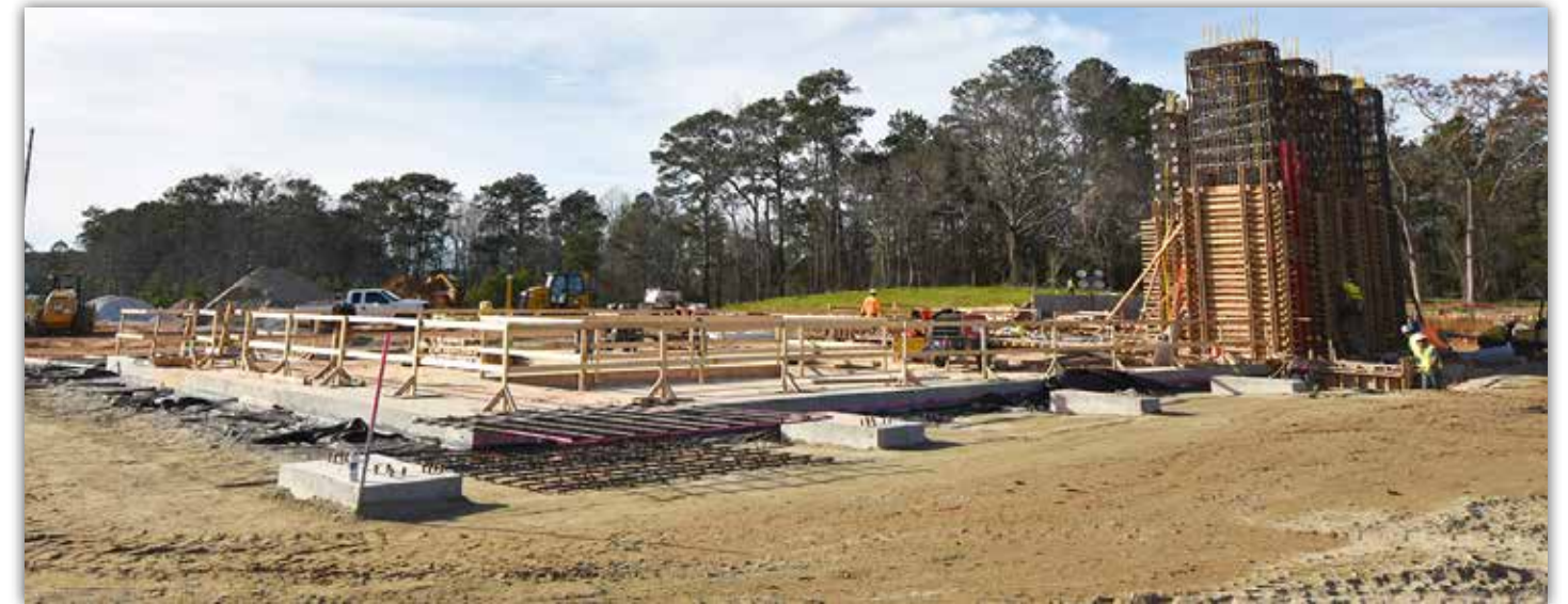
The strong floor and wall are taking shape. Structural testing will take place in this area of the building.
