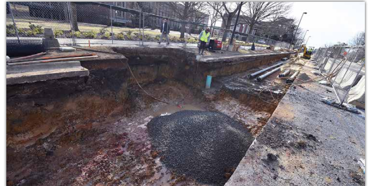
Excavation continues as underground power and water piping is placed along Thach. The utilities will supply the future Tony and Libba Rane Culinary Science Center with the resources it requires for everyday operations.
