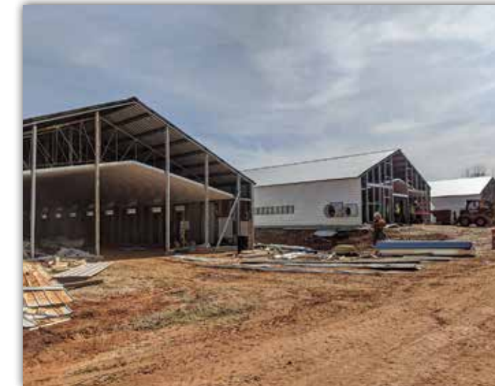
Construction of the pen houses is underway. These buildings will house chicks and chickens at the Poultry Research Farm.
