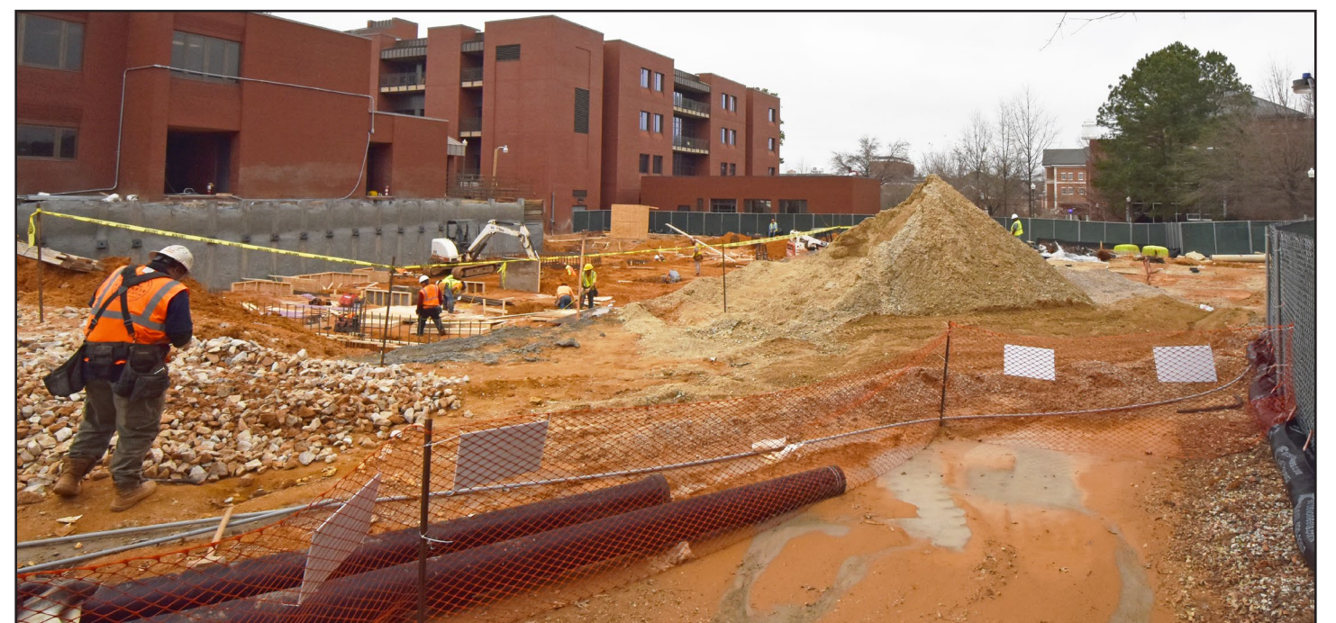
Site work continues to progress in preparation for construction of the building foundation.
