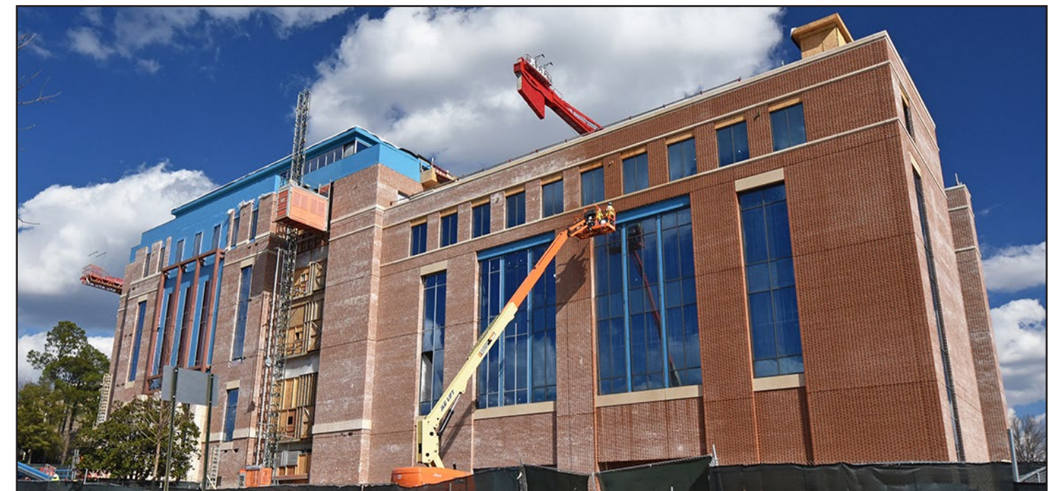
Brick installation nears completion on the South Donahue Drive side of the building.
