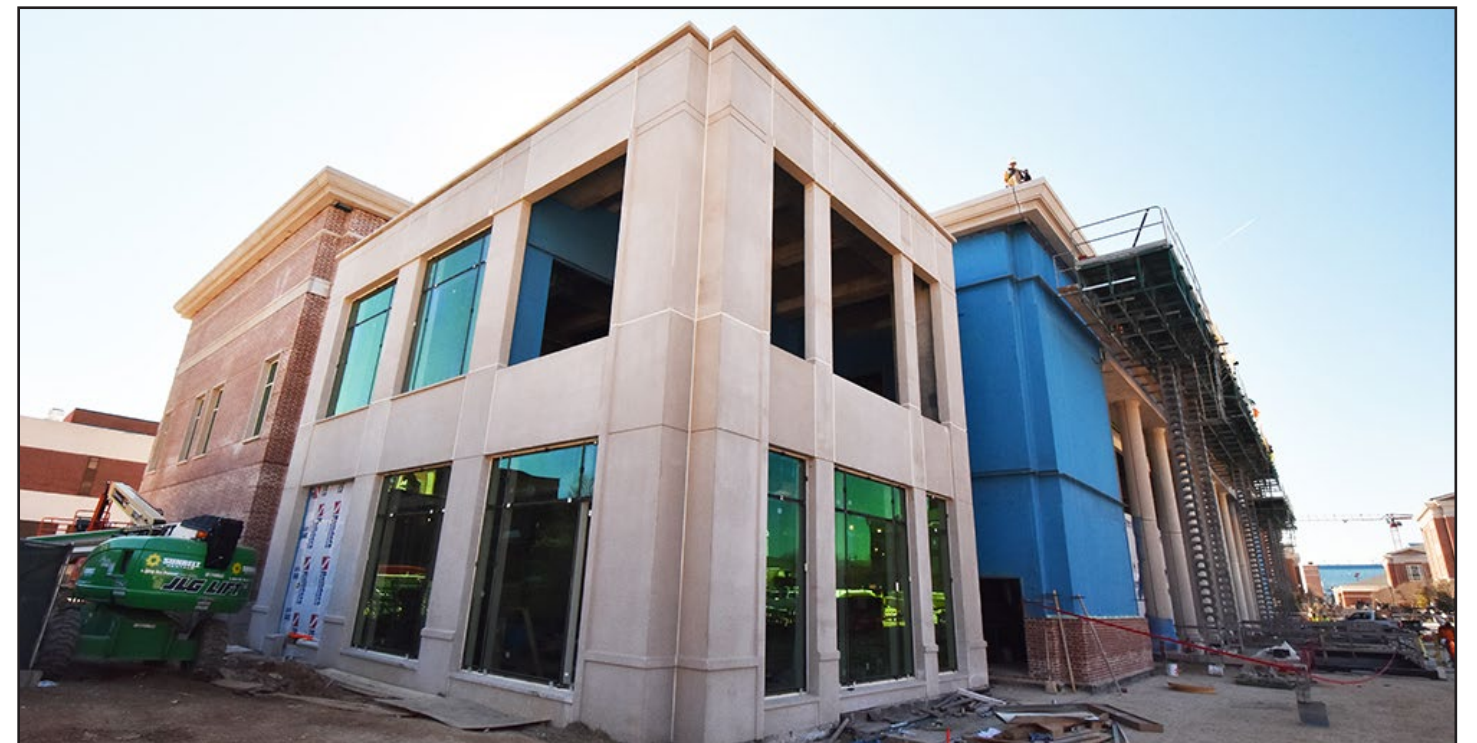
A view of the northeast corner of the building from Wilmore Drive. The first floor of this section will be a food service area. The second floor will be a balcony attached to a conference room.
