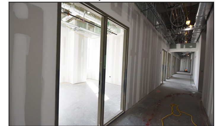
Drywall is going up for the office spaces located on the second floor.
