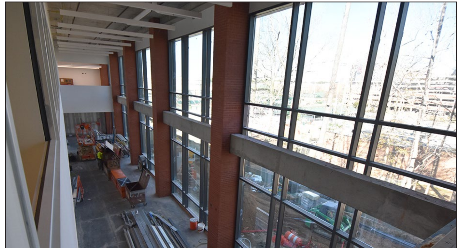
This two-story atrium will welcome students and faculty to the new center.
