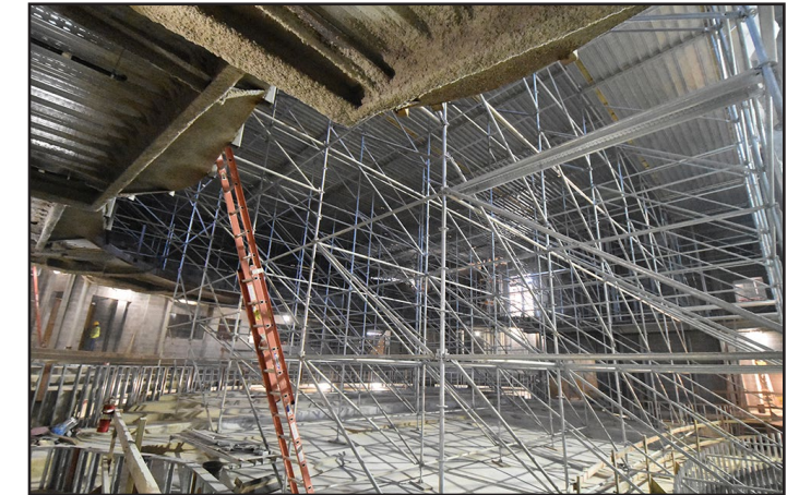
Scaffolding to be removed in March following completion of auditorium ceiling work.
