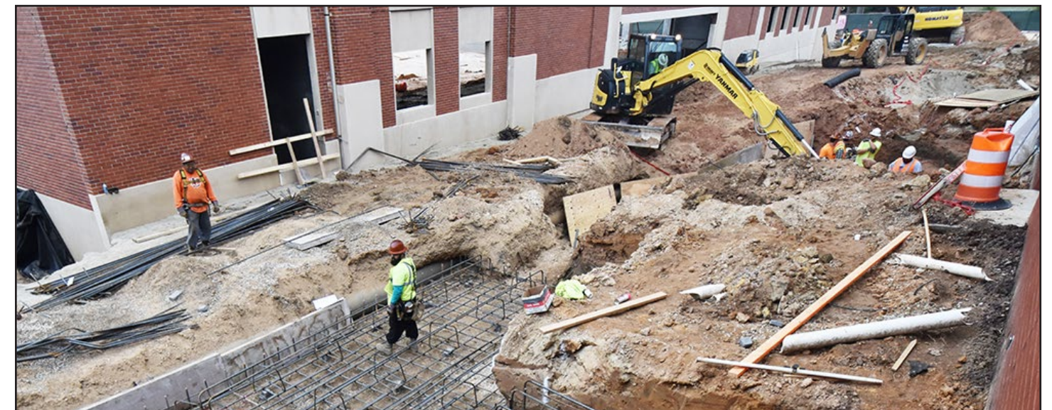
The south stairs currently are being rebuilt to connect the hotel and the parking deck.
