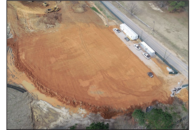
The parking lot of the Recreation Field Expansion is starting to take shape.
