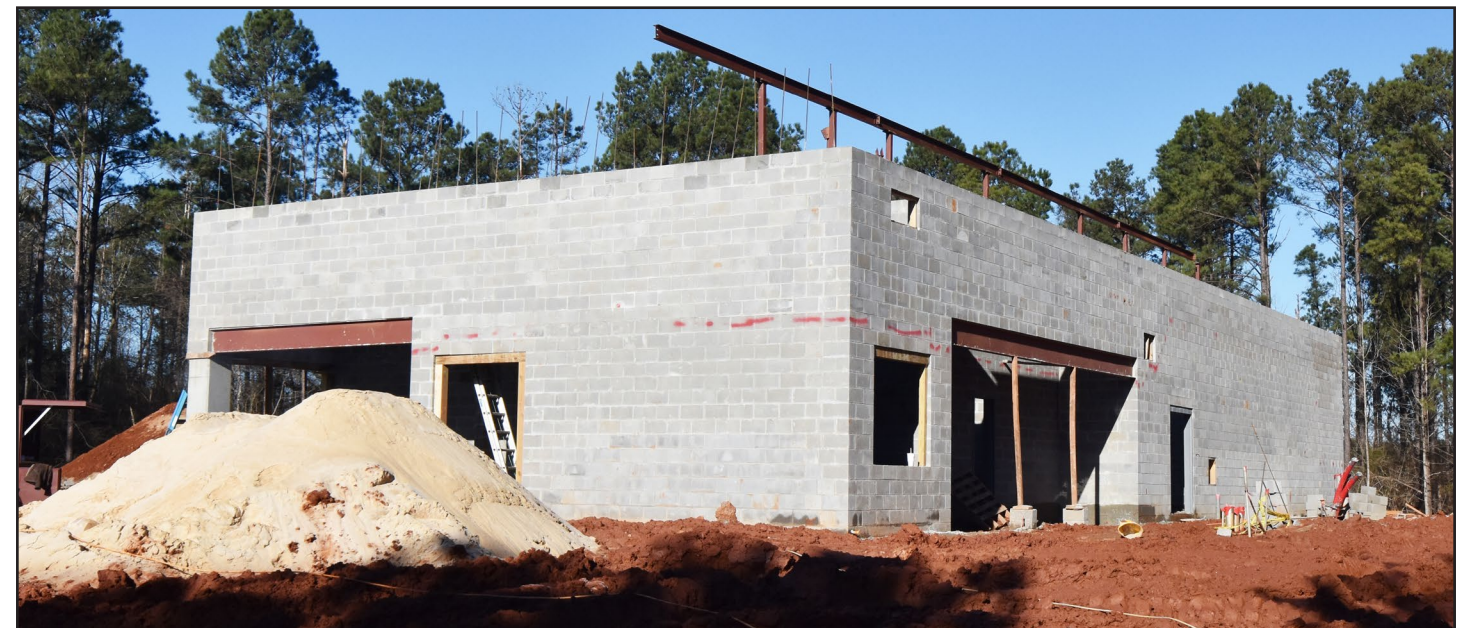
Block work for the Poultry Science Infectious Disease Lab is almost complete.
