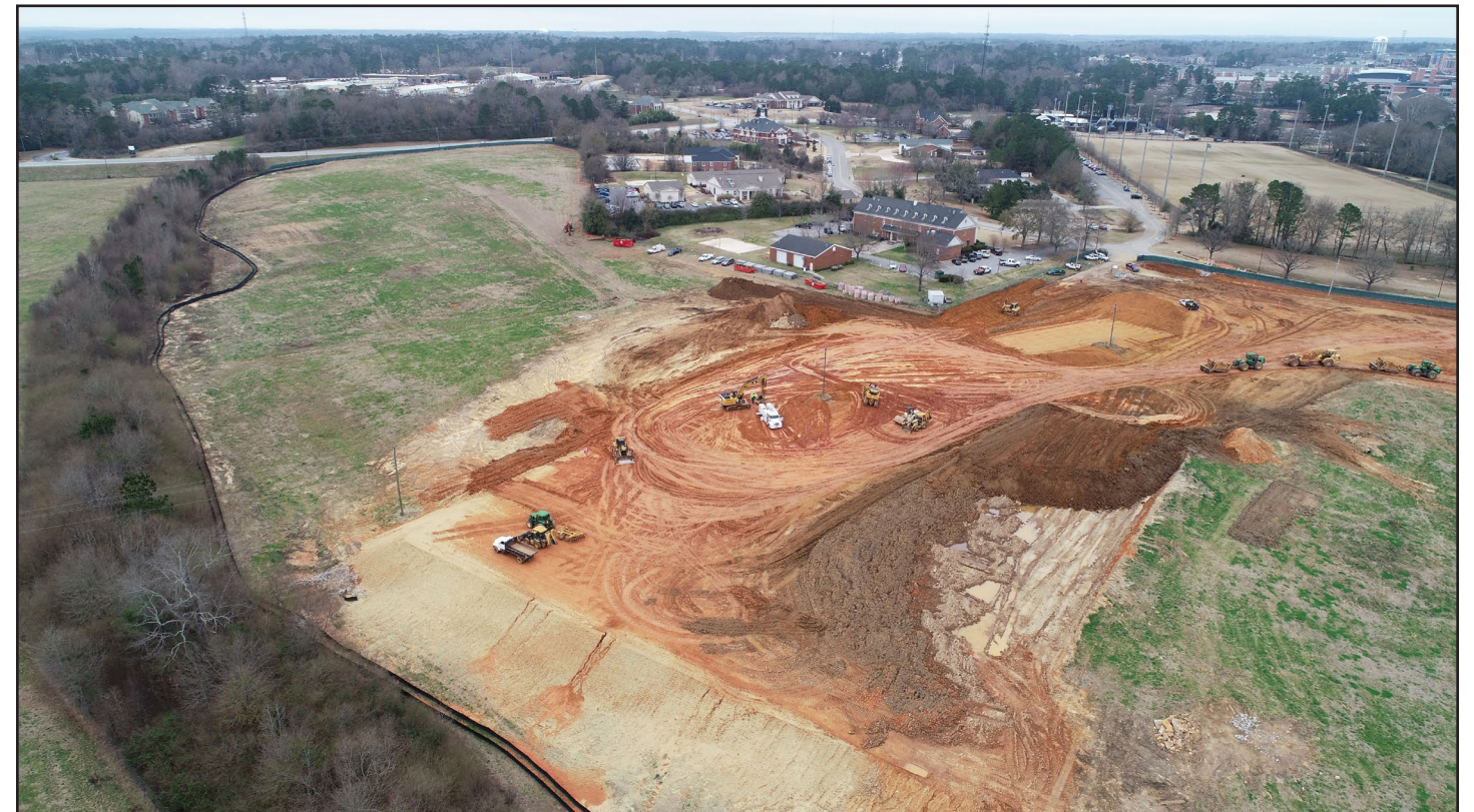
Grading for field two is nearing completion. The locations of fields three, four and five appear to the left in this photo.
