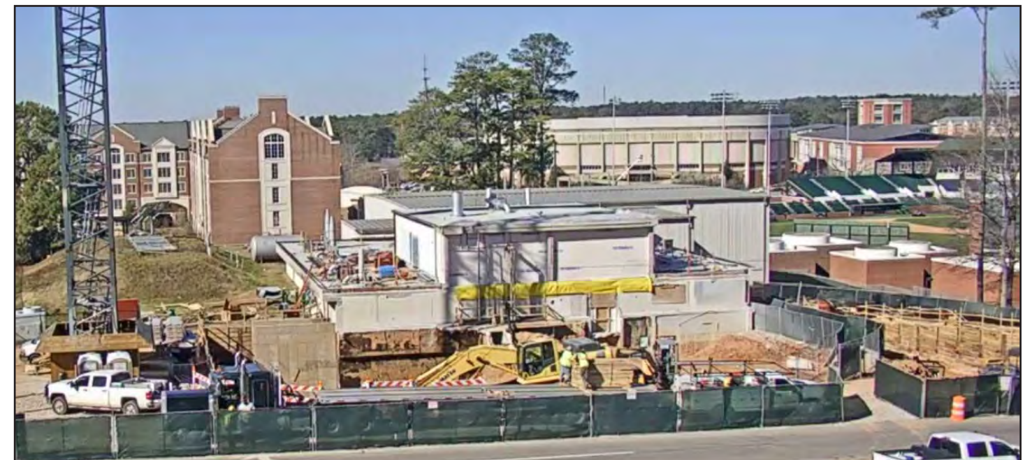
This view from the construction webcam gives an overall picture of the construction site.
