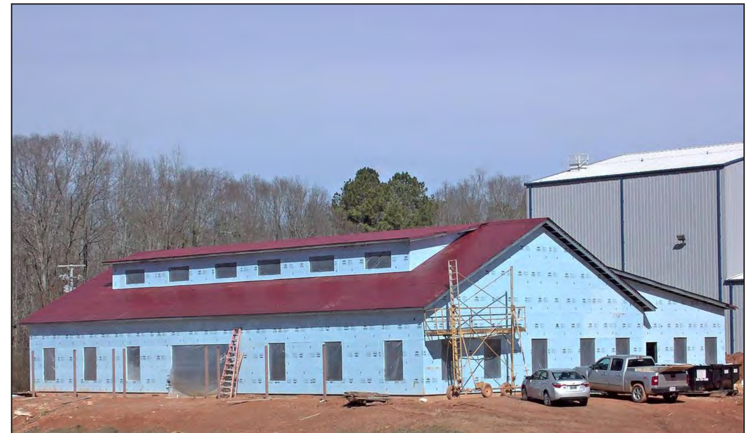
The view from the College of Agriculture's webcam shows where exterior insulation is being installed.
