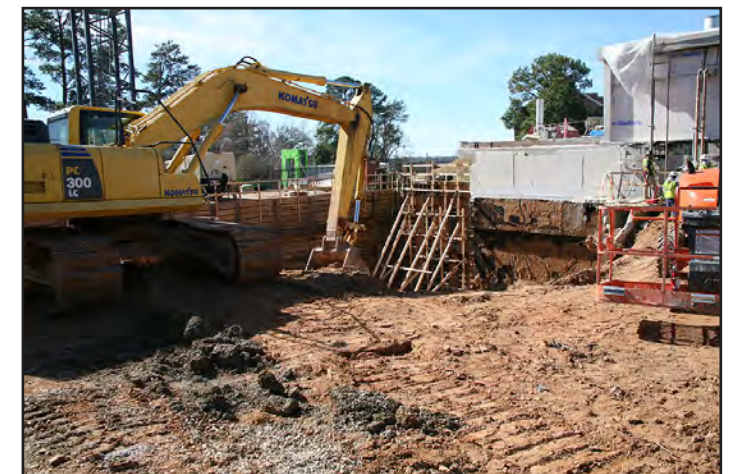
Forms are being built so that the concrete foundation can be poured.
