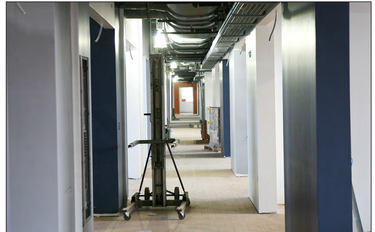
The new look is beginning to take shape as walls are being painted on the second and third floors.
