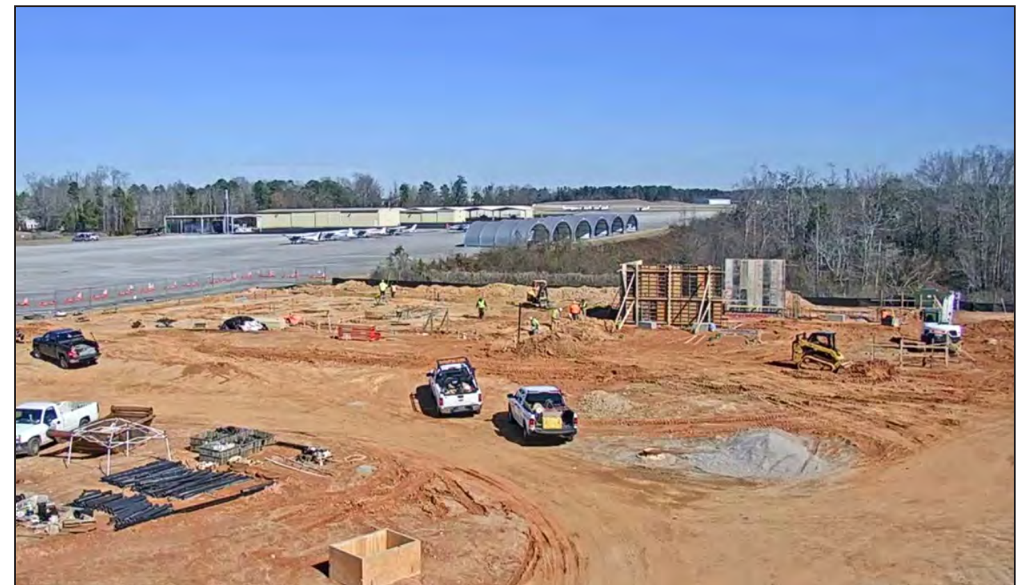
This view from the construction webcam gives an overall picture of the construction site.
