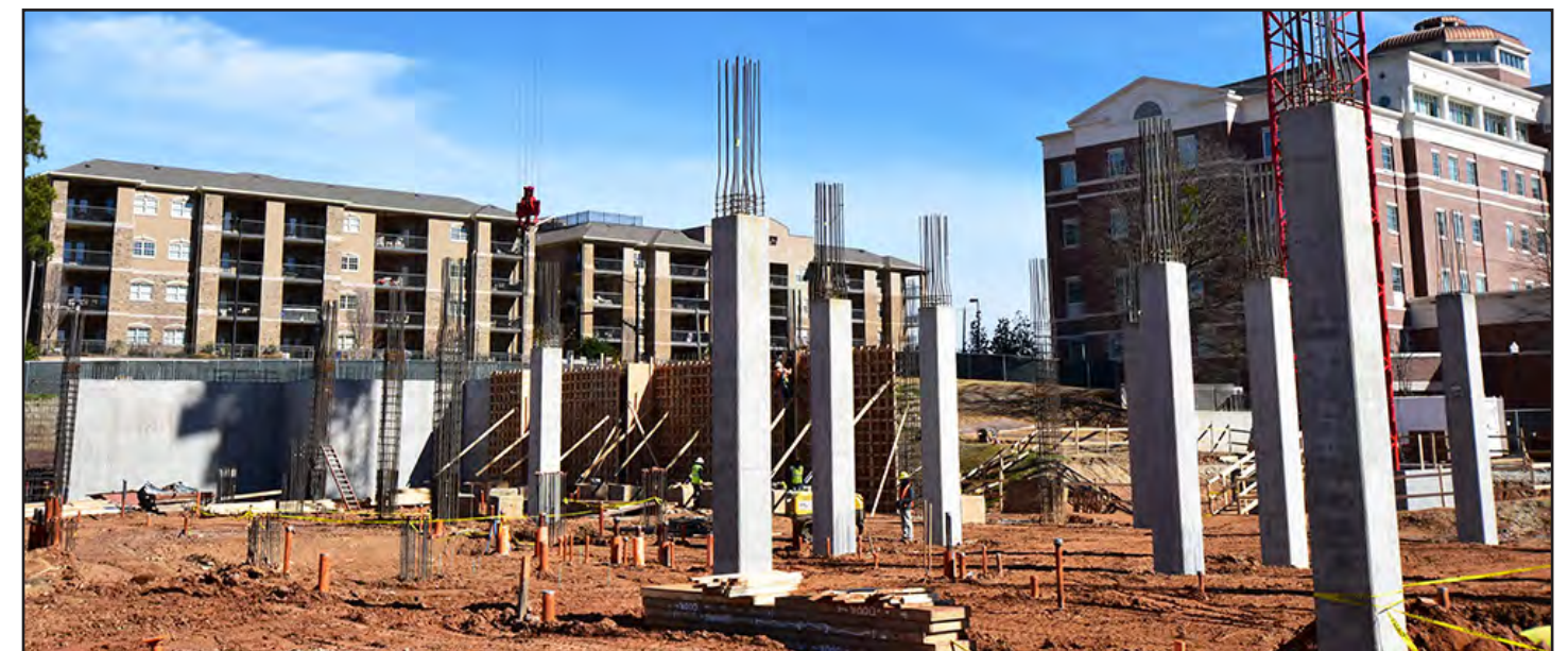
Concrete foundation walls are being poured on the northern side of the construction site.
