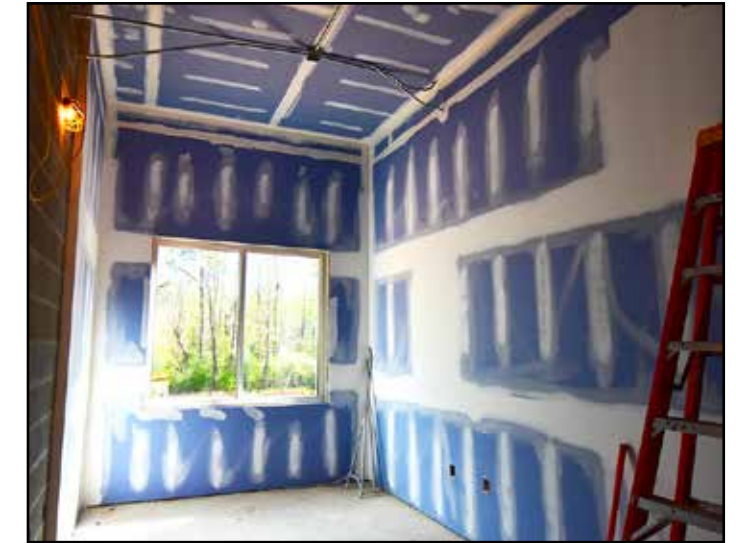
Drywall installation is complete and ready for paint inside this office space.
