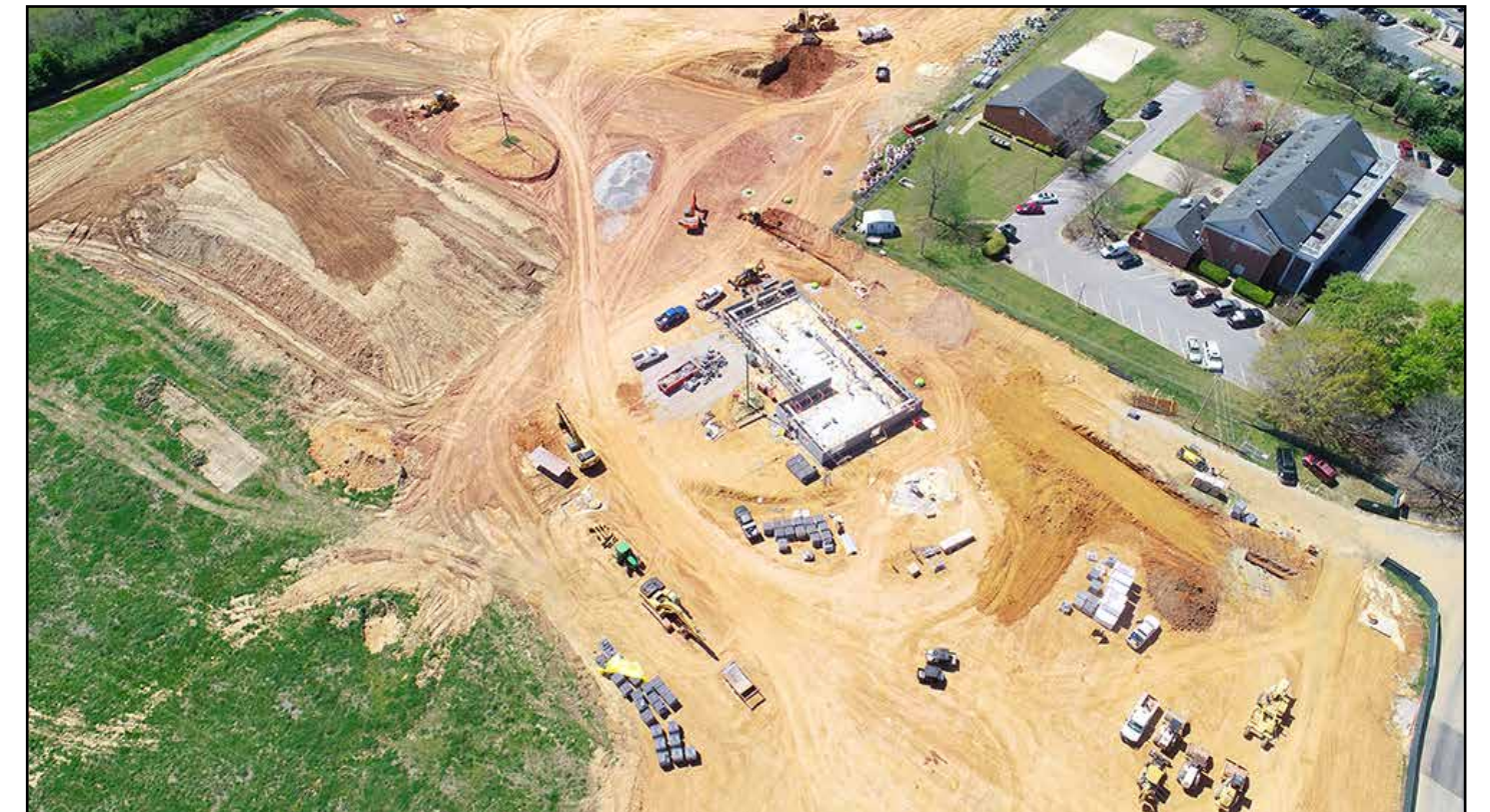
Block walls are being erected for the field house (center), while field two (left of the field house) is being used for topsoil storage.
