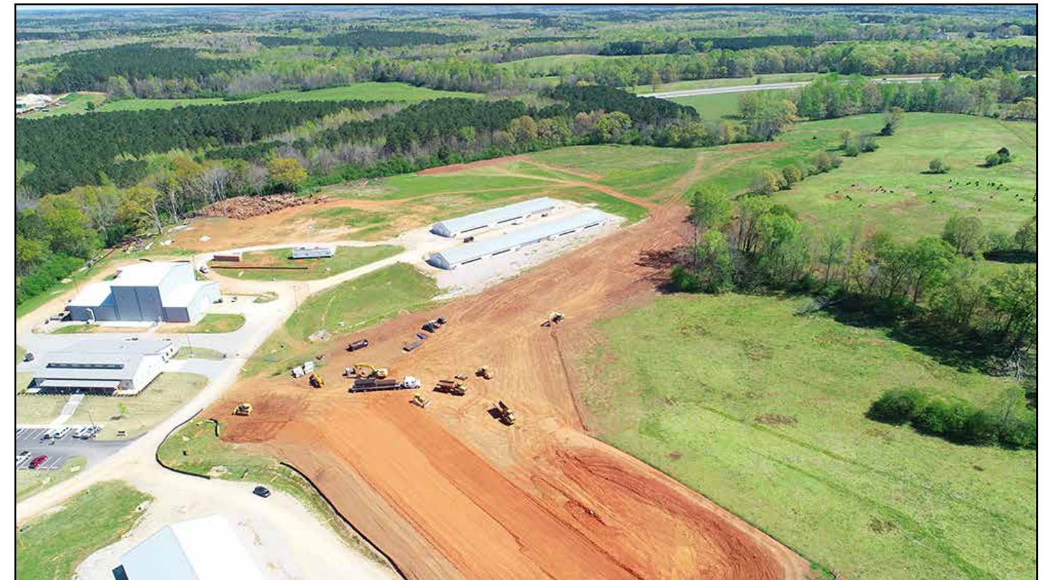
Site work continues to progress in preparation for pouring of the processing plant foundation (lower center). In the center of the photo, site work has begun for the ancillary buildings.
