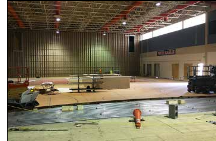
The extended stage and new wall in the multipurpose event space is nearing completion.
