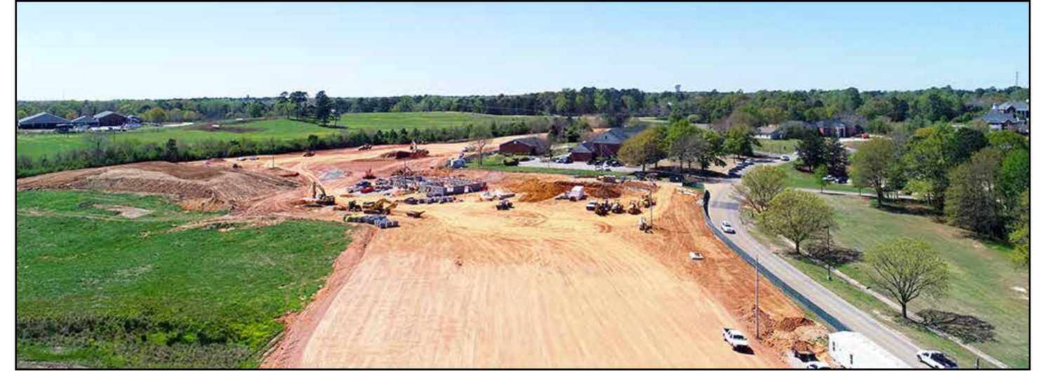
A view of the site from Woodfield Drive looking toward Wire Road shows the parking lot area and construction of the field house.
