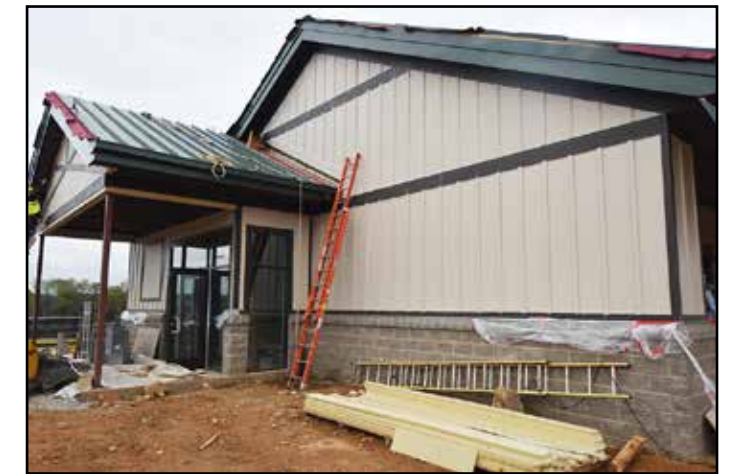
Entrance to the team support building where window and siding installation is complete.
