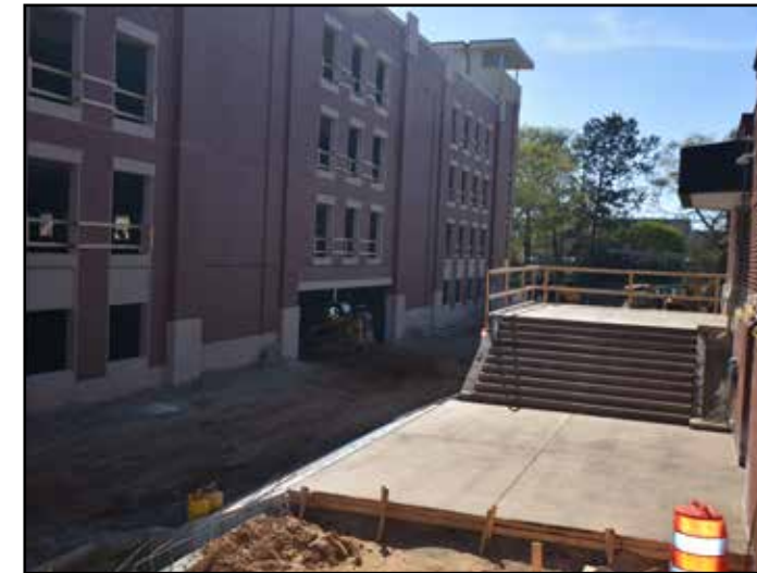
The south stairs adjacent to the hotel are currently being rebuilt to provide better access to the parking deck.
