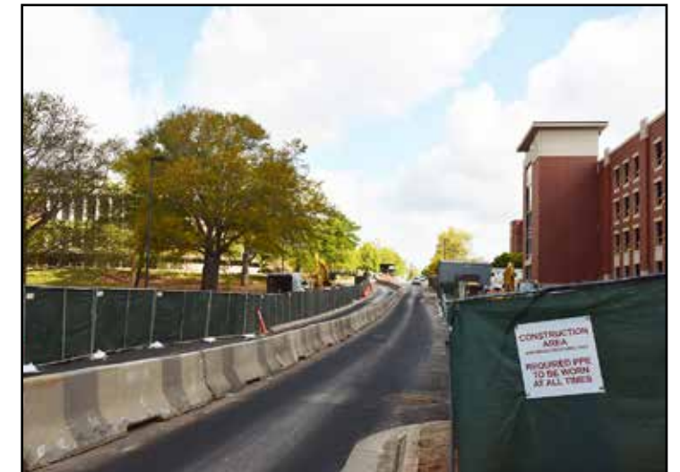
Road work is now complete in the eastern side lanes of South College Street in front of the construction site and has transitioned to the west side.
