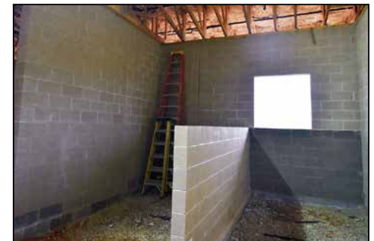
Once complete, this area will serve as grooming stalls inside the new barn.
