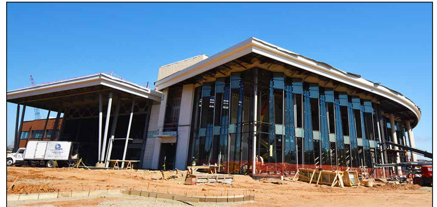
An exterior view of the glass curtain wall installation for the main lobby.
