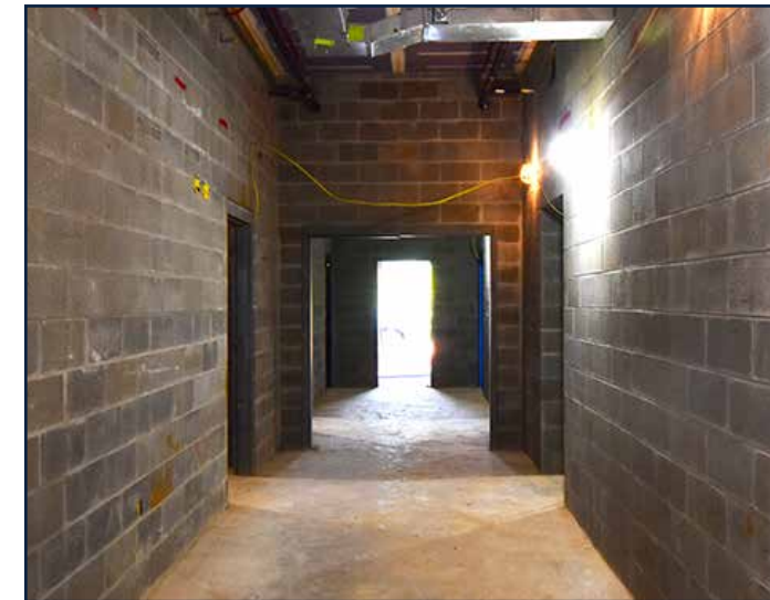
Construction of the interior block walls is complete and painting will begin soon.
