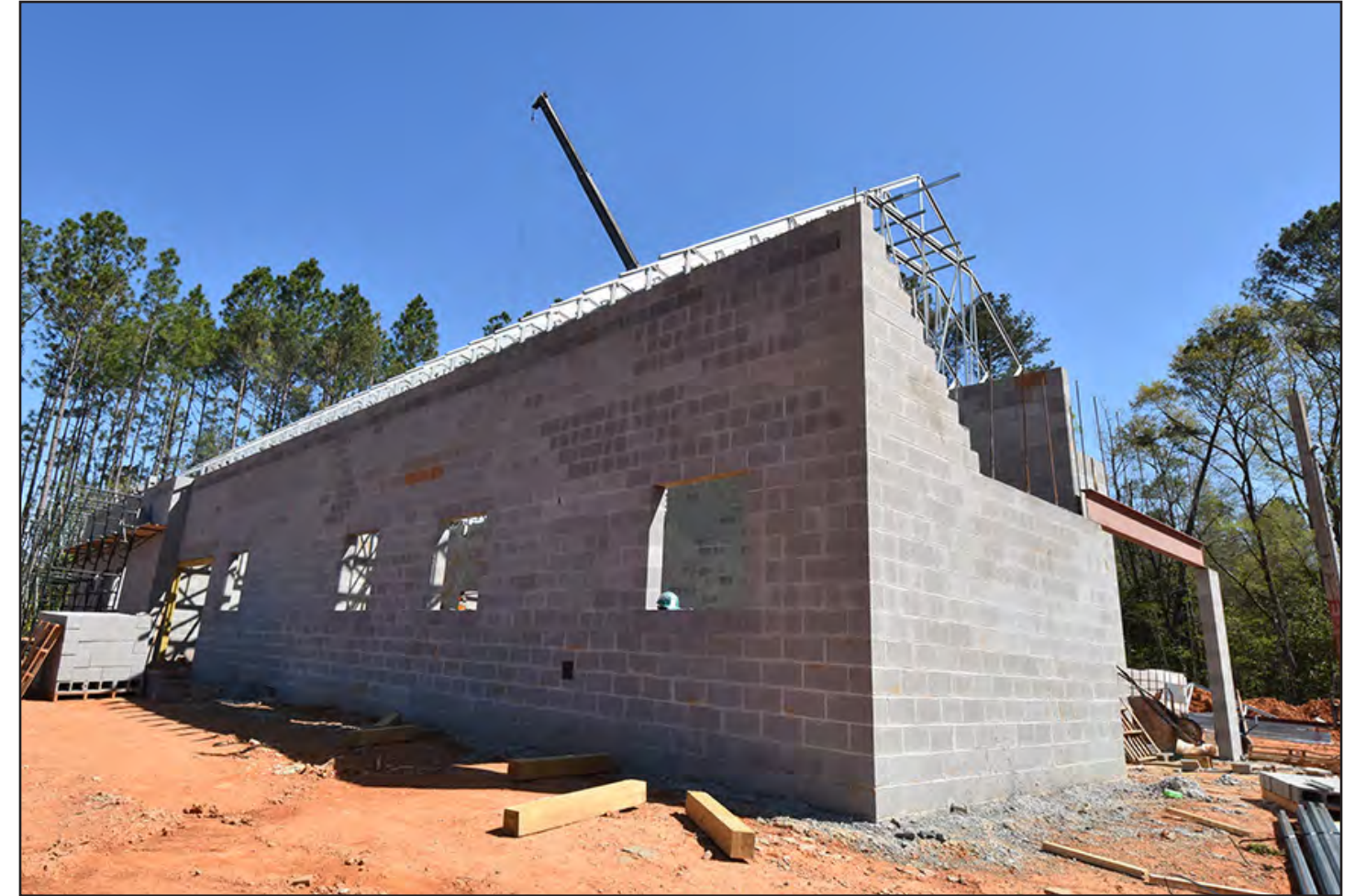
An alternate view of the building's block frame and metal roofing trusses.
