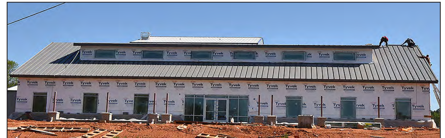
A view from the front of the center shows where columns are being installed, and final roofing details are being completed.
