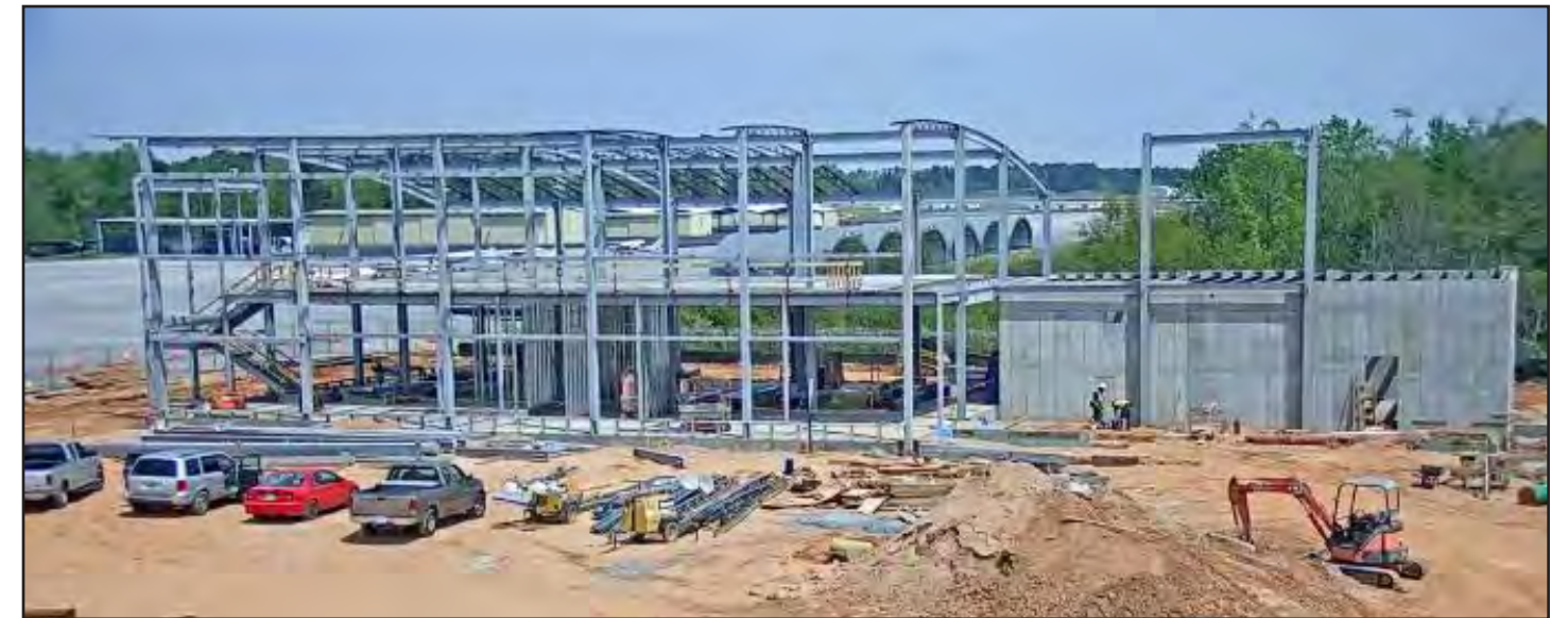
This view from the construction webcam gives an overall picture of the construction site.
