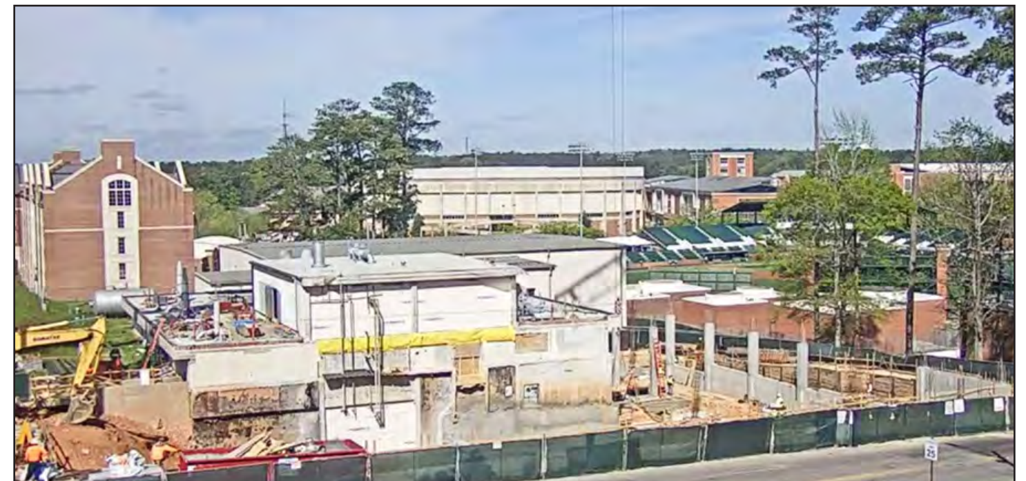
This view from the construction webcam gives an overall picture of the construction site.
