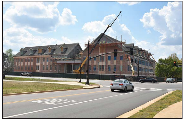
View of the new School of Nursing facility from Lem Morrison Drive.
