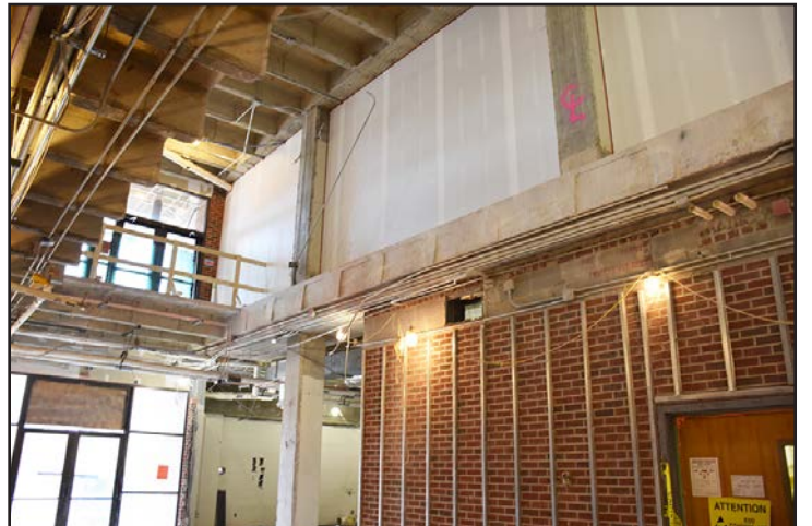
The flooring on the second level has been removed to create an atrium.
