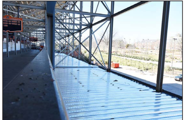
New metal decking shows extent of concourse widening. Diagonal bracing to be removed prior to completion.
