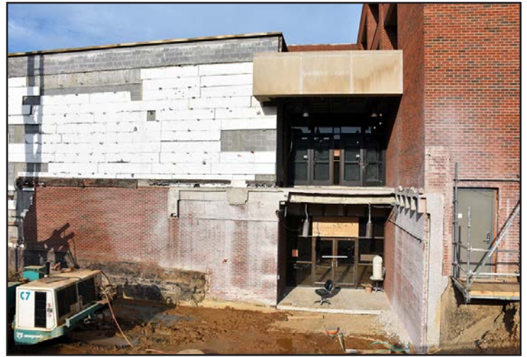
The original Broun Hall entry has been removed.
