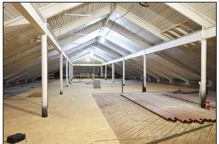
Third floor demolition is complete and ready for partition construction to begin.
