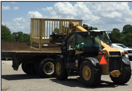
Joey Ellis uses a Lull to put the platform on a truck for transportation to Samford Lawn.
