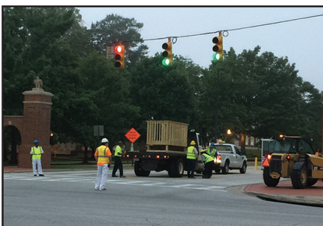
Everyone worked to ensure safety of the crew and pedestrians during the move, which took place at 6 a.m. to avoid traffic.
