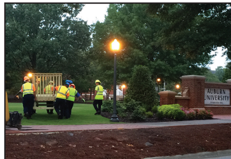
Crews carry the platform across Samford Lawn to avoid driving across the grass.
