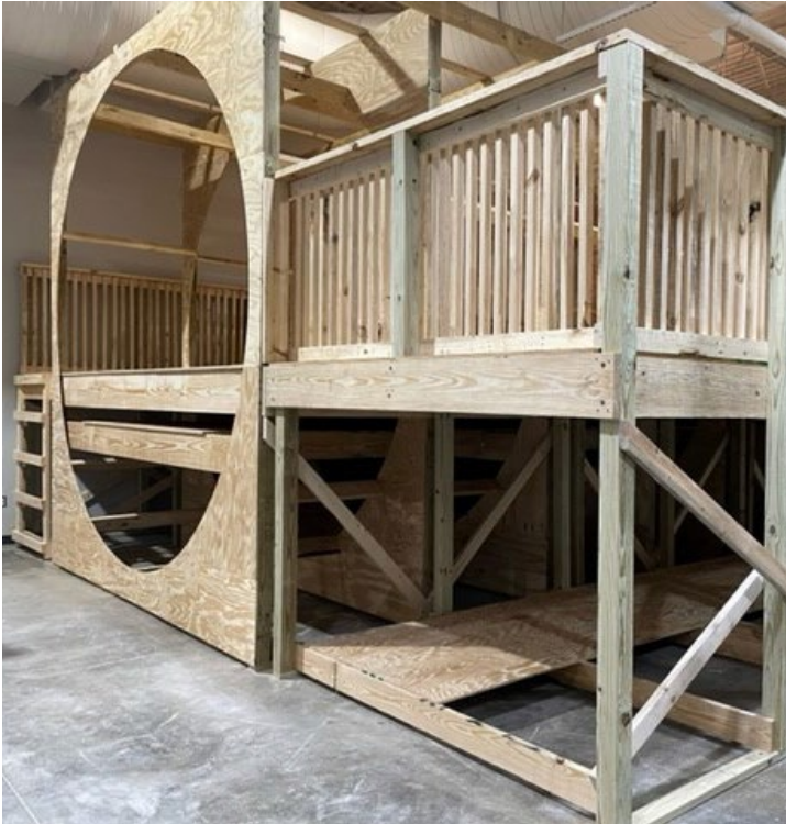
In-House Construction built this base structure for the university's first RFID research fuselage.
