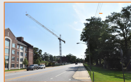
The construction crane for the Leach Science Center addition has been put into place. The crane is 130 feet tall and 246 feet wide.
