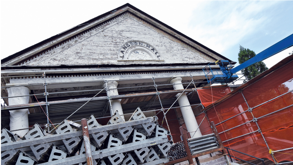
The wood and columns around Langdon Hall are being restored as part of a three-phase repair and restoration project being completed on the almost 180-year-old building.
