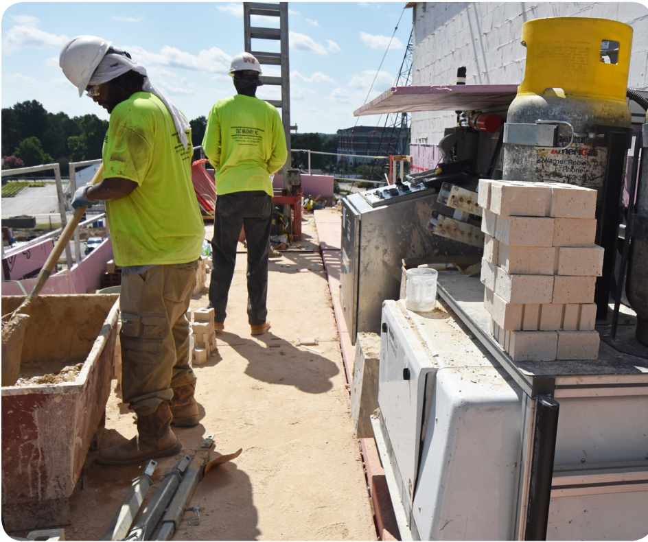
Masons load mortar and bricks into SAM, allowing it to continuously build the programmed pattern.
