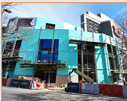
Jordan-Hare's Gameday Support Facility currently is being built along the outside of the stadium.
